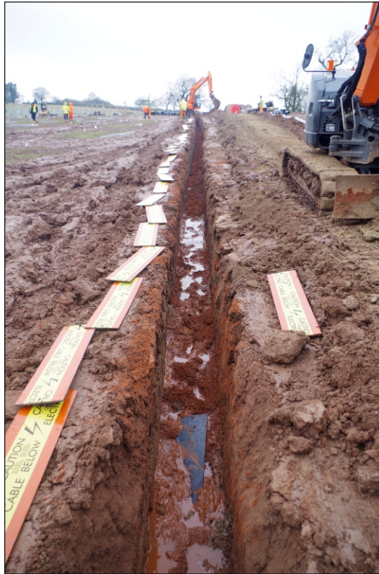
Plate 5: Overview of length of Trench 3, eastern edge of Site, looking north, no scale
