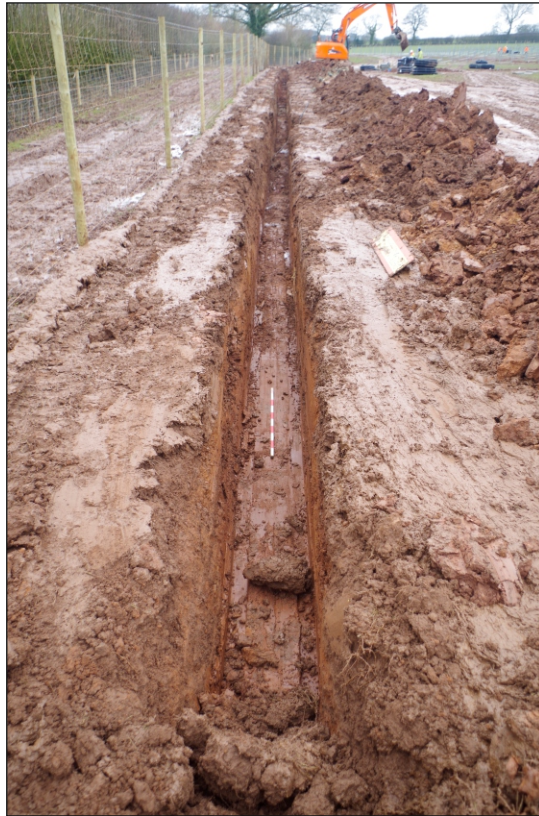
Plate 3: Overview of length of Trench 2, southern edge of Site, looking west, 1 x 1 m scale
