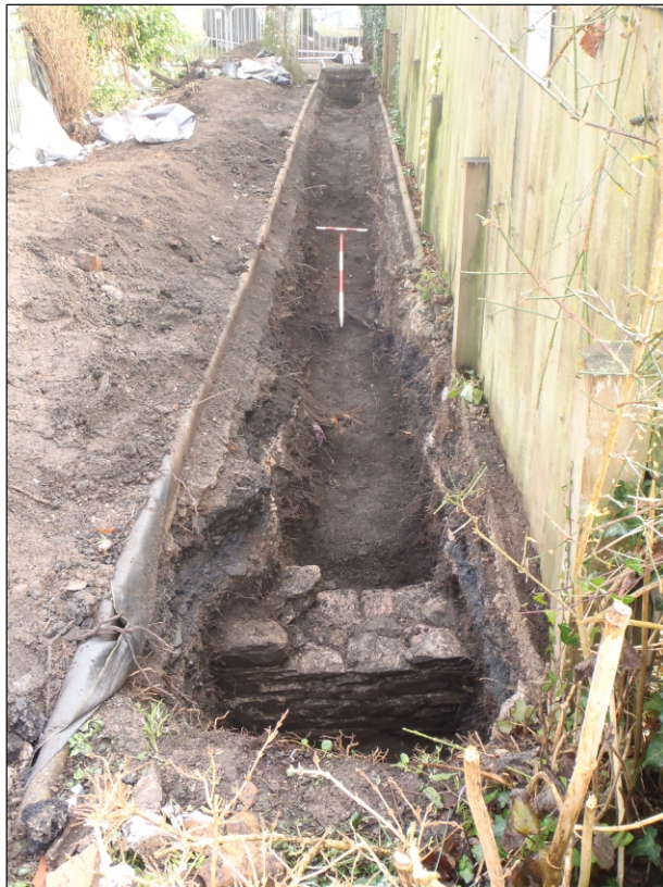
Plate 2: Full length of Trench 1 after excavation, looking east, 1x1m and 0.50m scales
