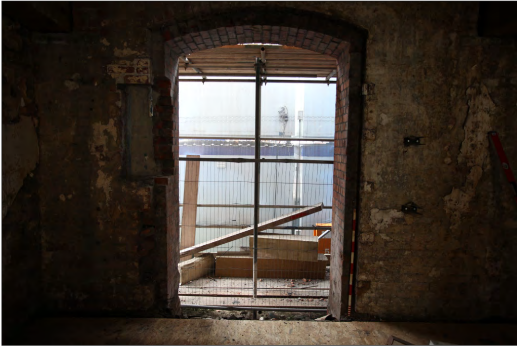
Plate 3: The ground floor of Huller House, doorway in northern corner of eastern elevation, 1m scale
