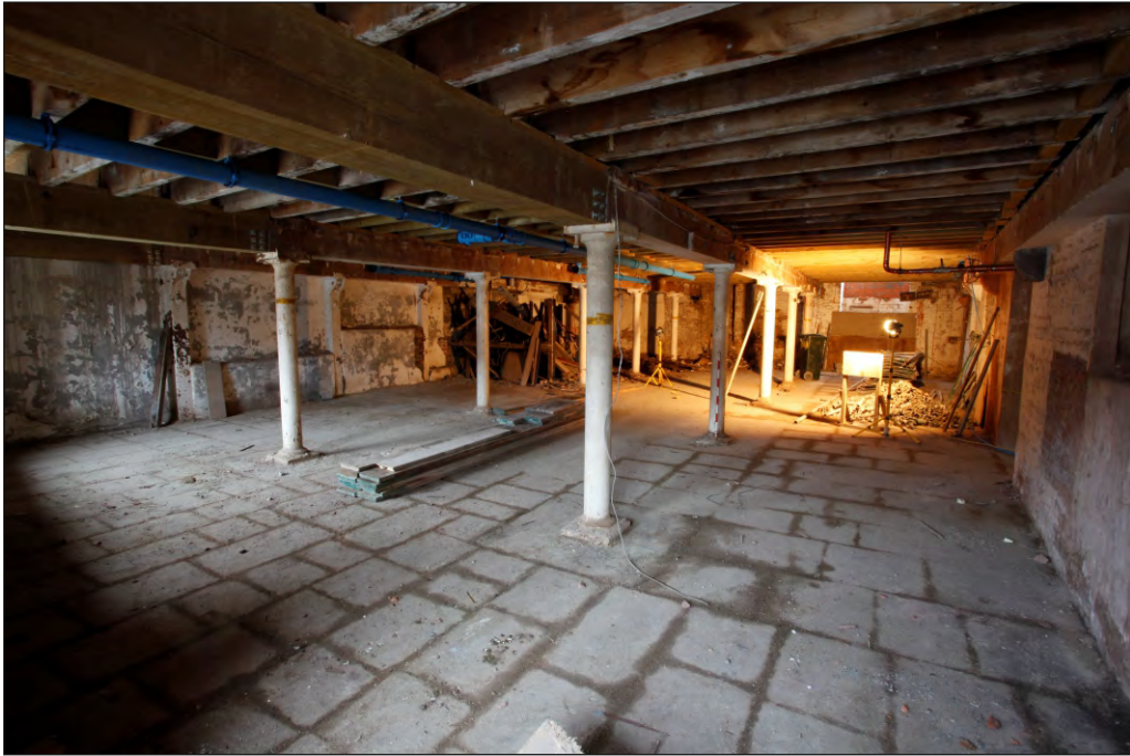
Plate 5: Basement of Huller House, northern elevation looking towards NE corner, 1m scale
