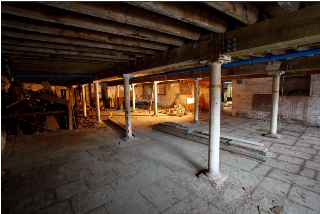
Plate 4: Basement of Huller House, iron columns and flagstone floor, looking towards SE corner, 1m scale
