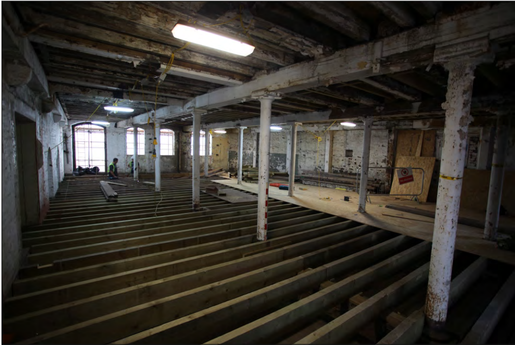
Plate 1: The ground floor of Huller House, looking towards the NW corner, 1m scale
