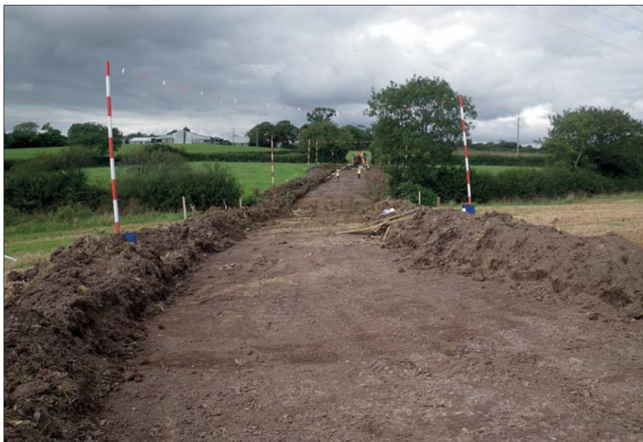
Plate 8: Working shot; Excavation of the RMA Haul Road in Field 36 viewed from the south-west
