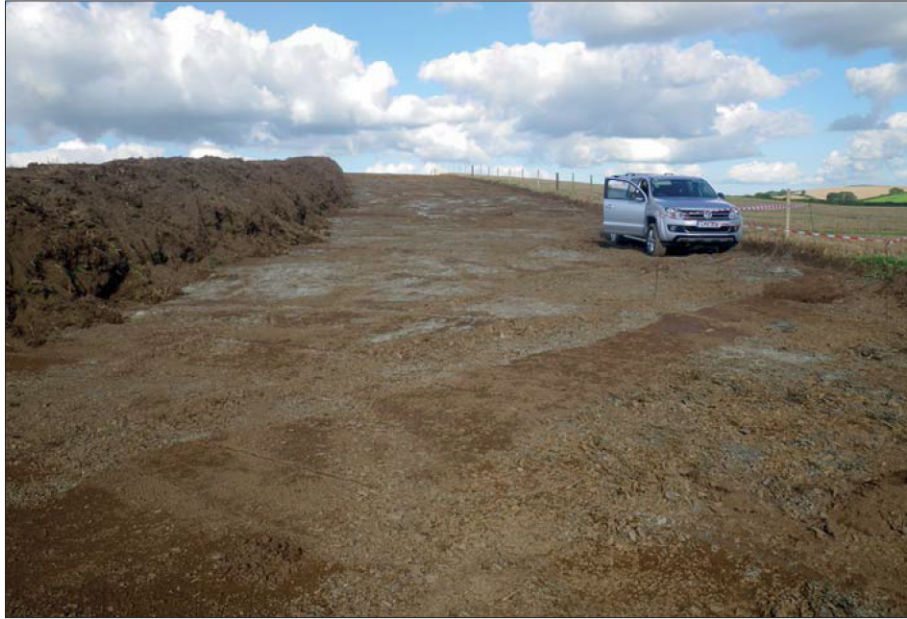
Plate 3: View of Earthworks Surcharge Haul Road in Field 40 from the south-west with 80317 in the foreground
