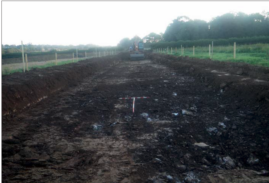
Plate 5: Working shot; Excavation of the RMA Haul Road in Field 8 viewed from the west (1 x 1 m, 1 x 2 m)
