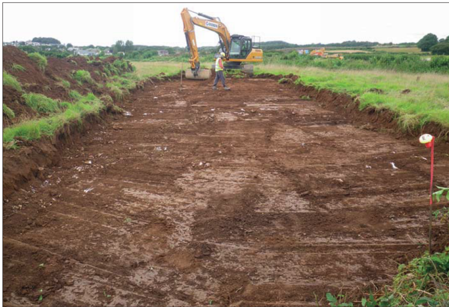
Plate 4: Working shot; Excavation of the RMA Haul Road in Field 5 viewed from the east
