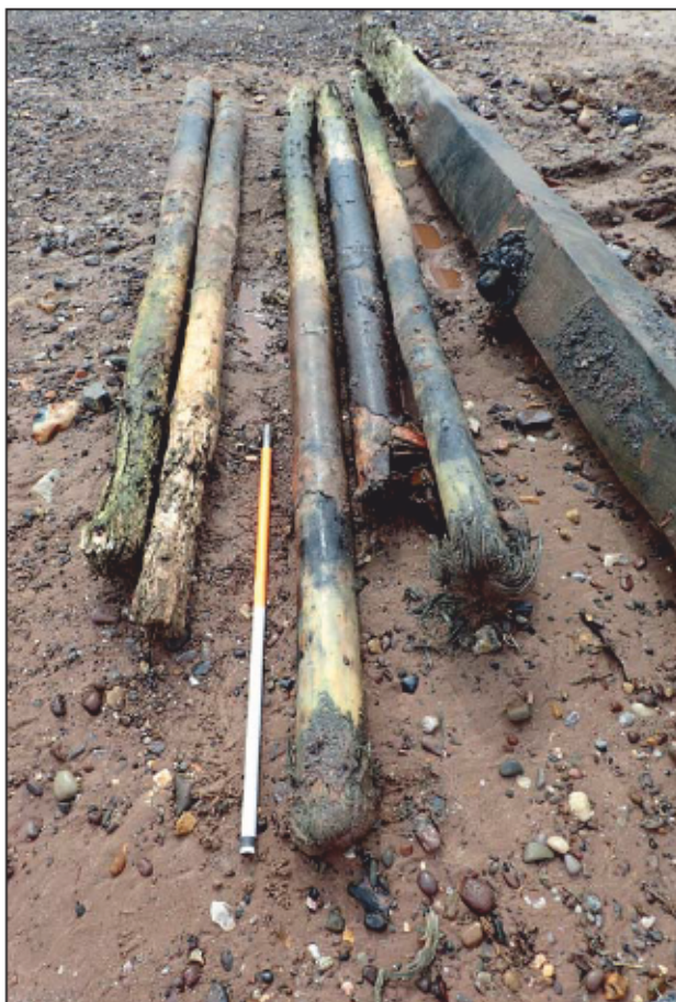
Plate 5: Softwood round posts from the 'Zig-Zag' groyne with piling damage
