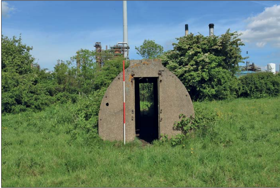
Plate 37: View of western elevation of Air Raid Shelter 3, with truncated escape hatch projecting from the roof
