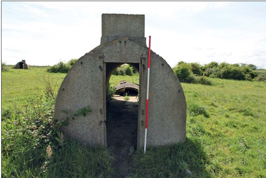
Plate 34: View of eastern elevation and entrance to Air Raid Shelter 2, with truncated escape tunnel projecting above
