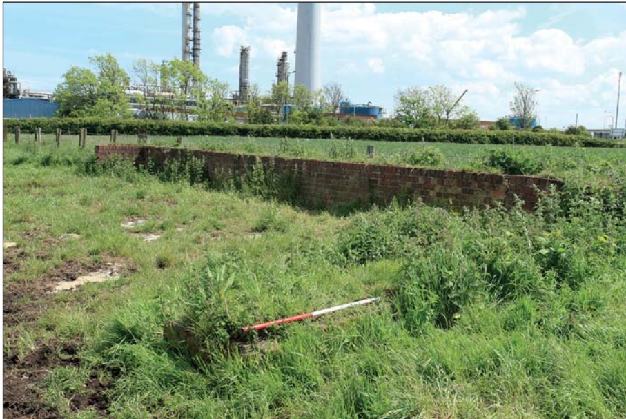
Plate 4: View of partially collapsed south-western wall
