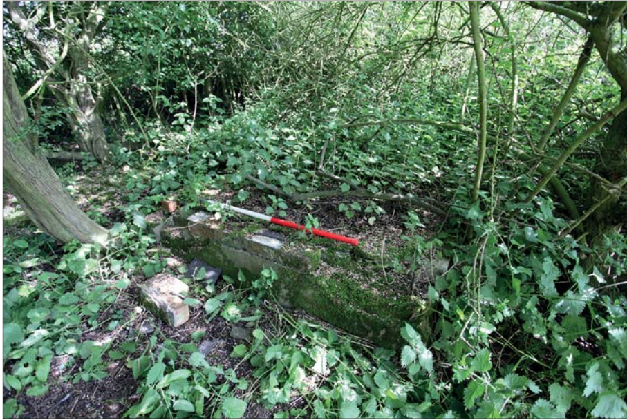
Plate 29: View of foundations of projection at northern end of C2 with remnants of slate damp-proof coursing visible
