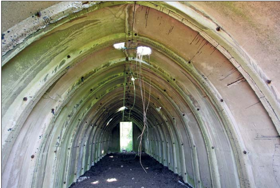
Plate 38: View of interior of Air Raid Shelter 3 with joints of pre-cast arches visible
