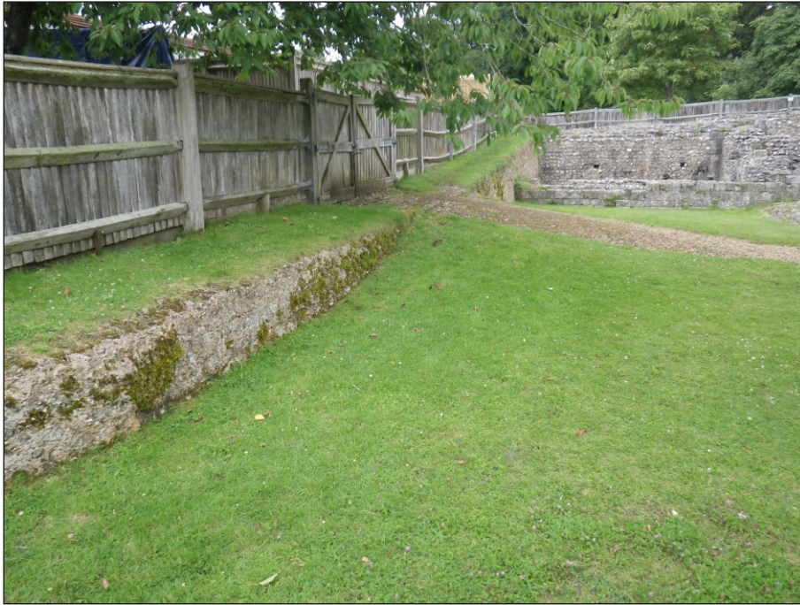
Plate 1: Western return of the fence line prior to replacement, viewed from the north-east
