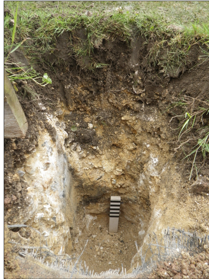
Plate 4: Post hole 18 at the west end of the fence to be replaced
