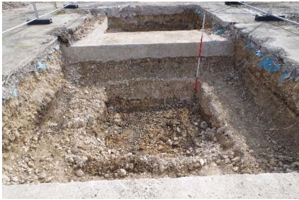
Trenches 7 and 8 showing later 20th century foundations and levelling over natural deposition
