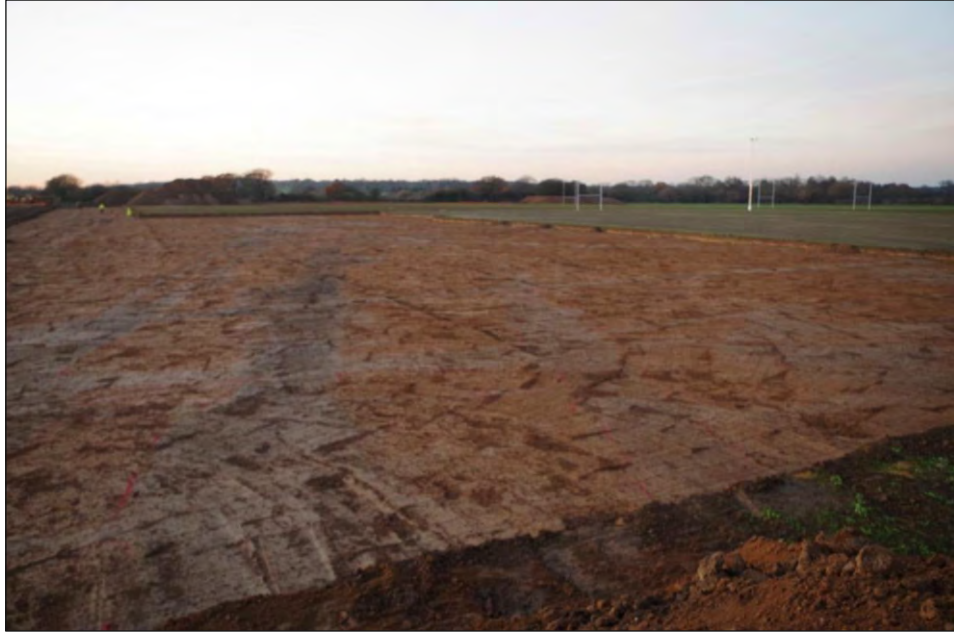
Plate 31: Pre-excavation photo of future clubhouse location within phase 1 excavation, view from the southeast
