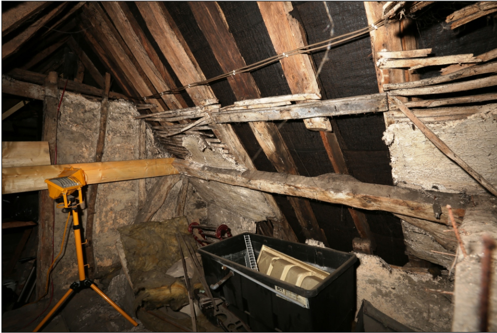
Plate 9: North side of roof in Bay 3, with cut rafter and possible trimmer for a window, looking north-west
