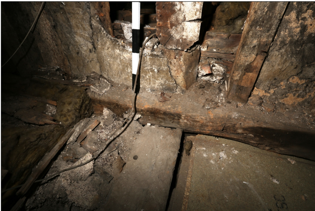
Plate 12: Forelock bolt in tie beam of Truss 4, with chock and chamfered beam of Bay 4, looking east
