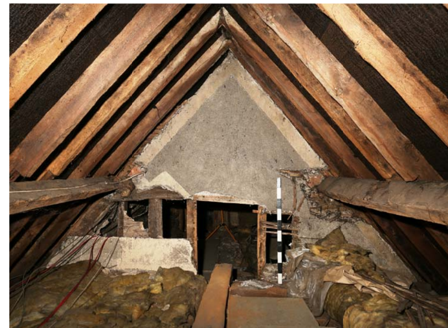
Photograph of Truss 4, viewed from the east, showing rendered gable end covering studwork.
