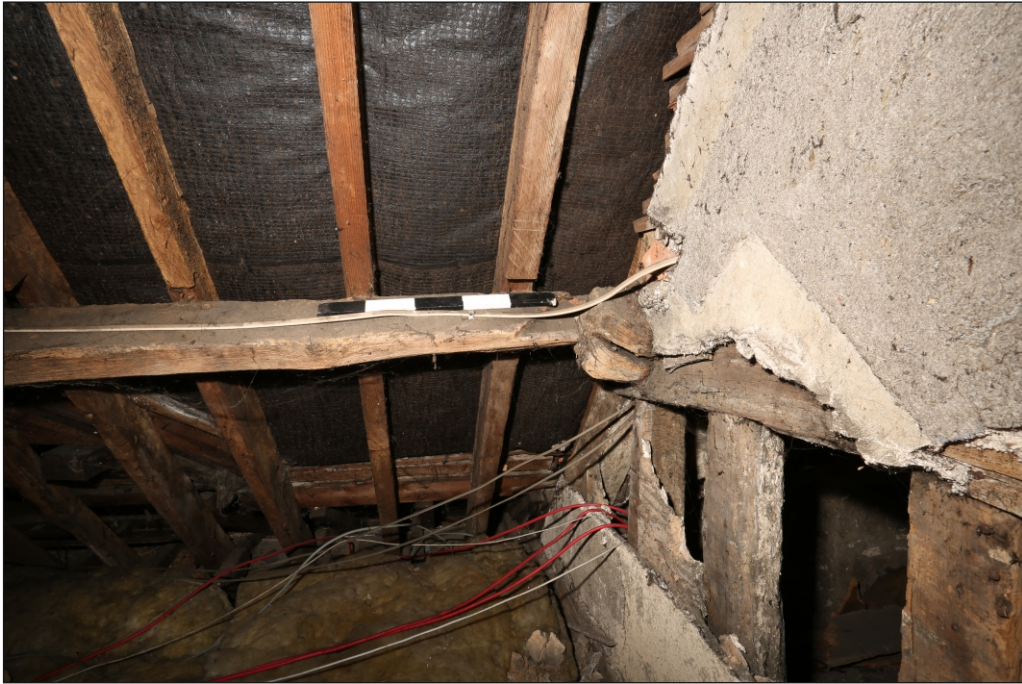
Plate 11: East face of Truss 4 with exterior plasterwork and protruding purlin end, looking south
