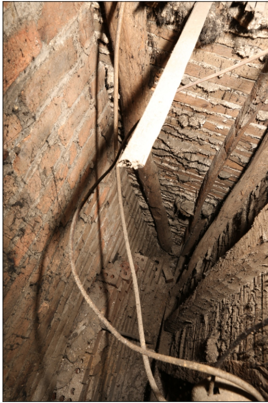
Plate 5: View looking down void beside east of chimney, showing fireplace on first floor blocked with bricks, looking north-west
