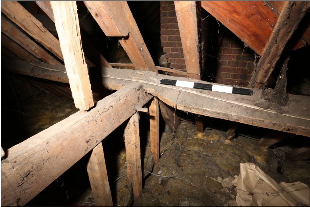
Plate 15: Cut away purlin on the south side of Bay 4 and its scarfed joint to the purlin of Bay 5, looking south-east
