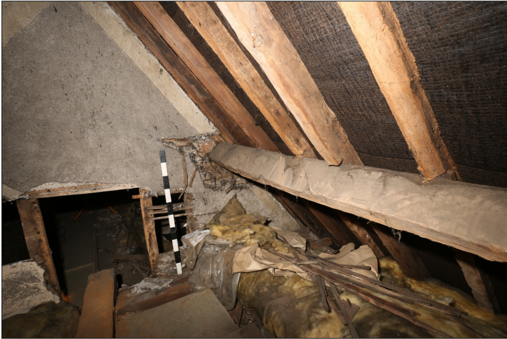
Plate 13: Purlin on north side of Bay 4, with a notch for a wind brace showing its earlier use, looking north-west
