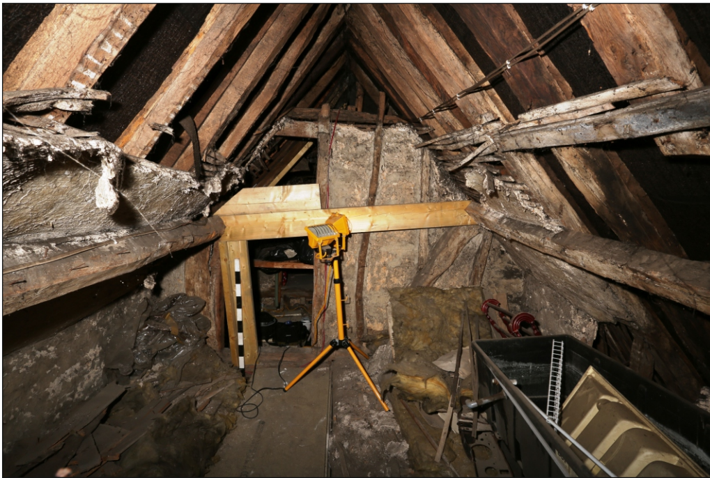
Plate 6: Truss 3 in Bay 3 containing north queen strut, looking west
