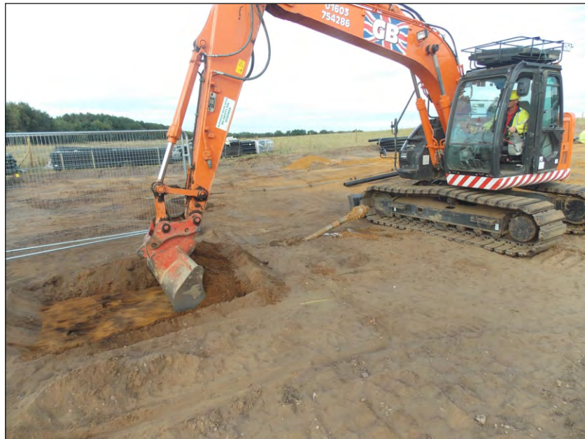
Plate 20: Working shot of the HDD receiver pit in the northern field, viewed from the west
