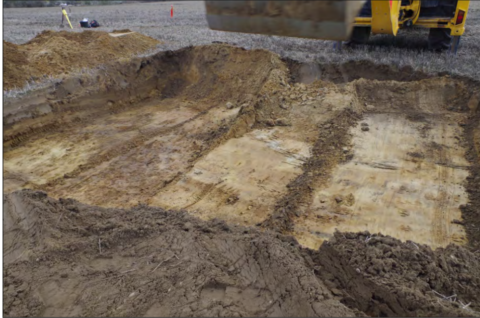
Plate 1: Working shot of machine excavation during UXO clearance, viewed from the west
