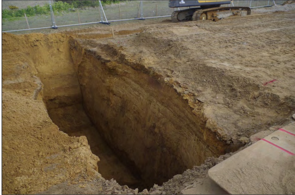
Plate 5: Deep excavation for winch anchor point in eastern field/compound area, viewed from the south
