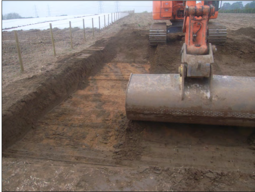
Plate 11: Cable easement in western field showing deep ploughing scars in natural sand, viewed from the east
