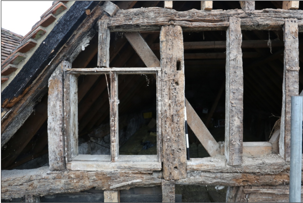
Plate 37: Reused timber stud and window located above the tie-beam in the south-east elevation
