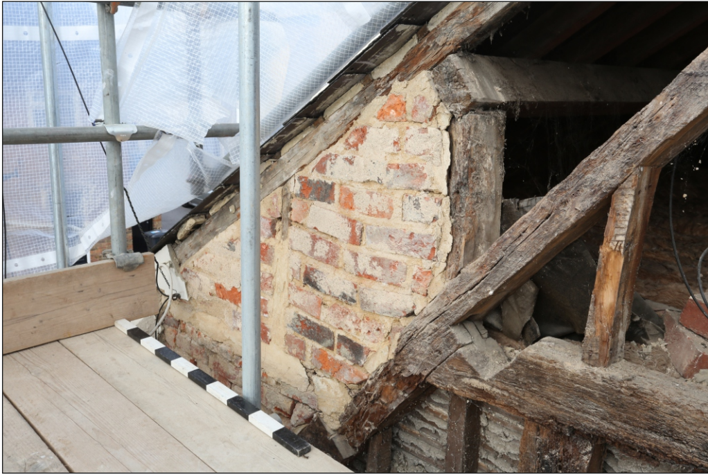
Plate 27: The north-west side of the south-west elevation at collar/roofspace level, showing the brick noggin infill and arrangement of the collar, principal rafter and purlin
