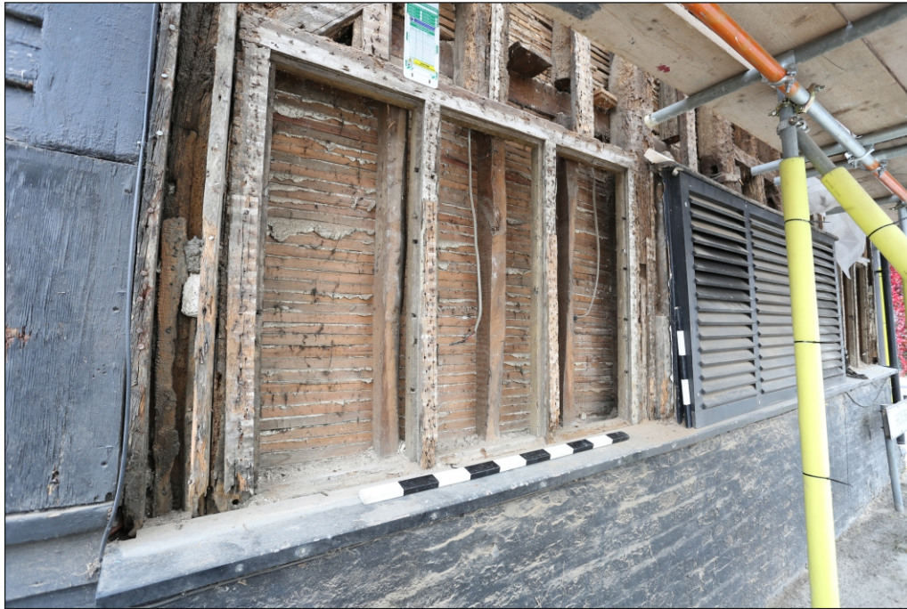
Plate 7: The north-east elevation at ground level, viewed from the east and showing a former window frame
