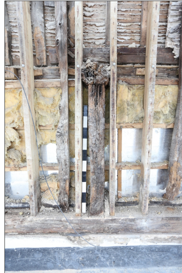
Plate 26: Post and ceiling beam supporting the first floor joists and floor boards in the SW elevation
