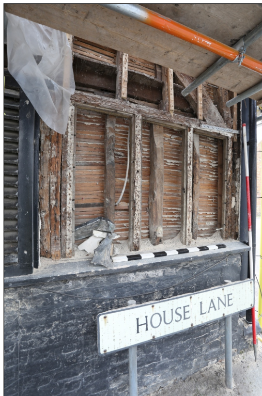
Plate 8: North-west side of the north-east elevation at ground level and showing a former window frame
