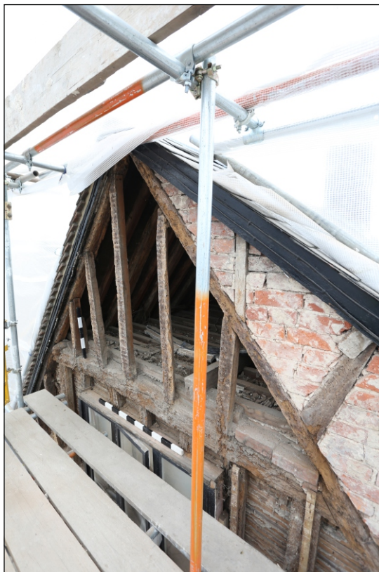
Plate 13: The north-east elevation at collar/roofspace level, viewed from the north-west, focused on the timber frame
