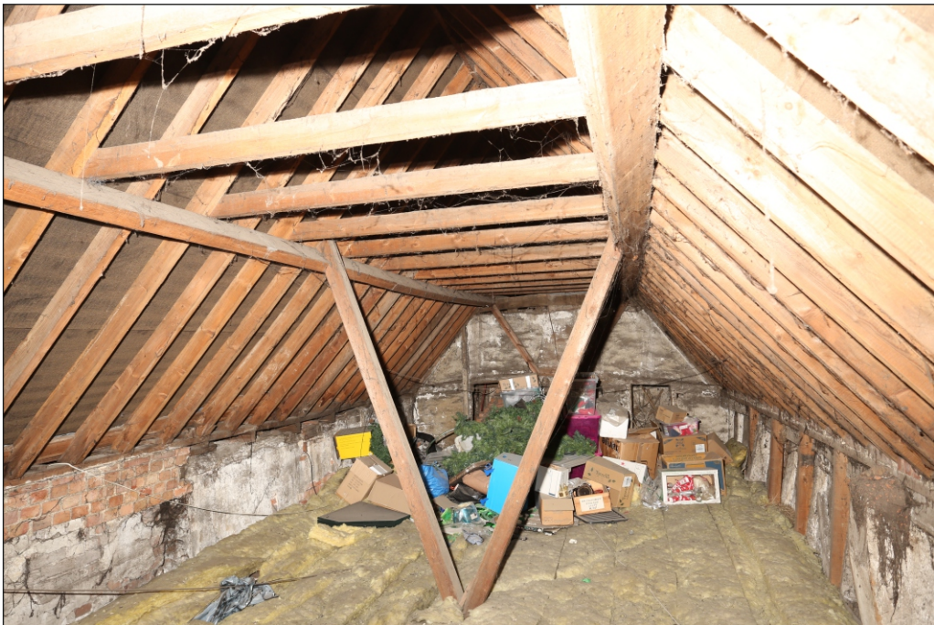
Plate 40: The roofspace within the north-east part of rear range, viewed from the south-east
