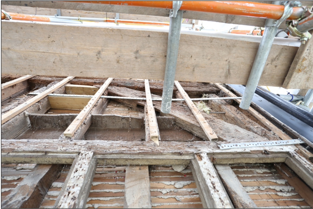
Plate 15: Empty mortise in the north-west up-brace in the north-east elevation
