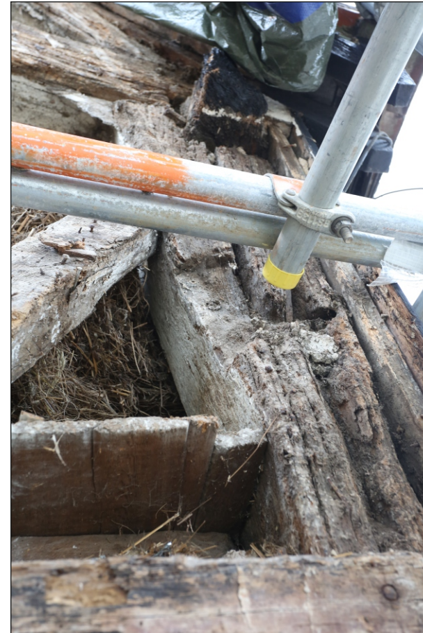
Plate 34: Detail of the empty half-lap joint on the north-east jowled post in the south-east elevation
