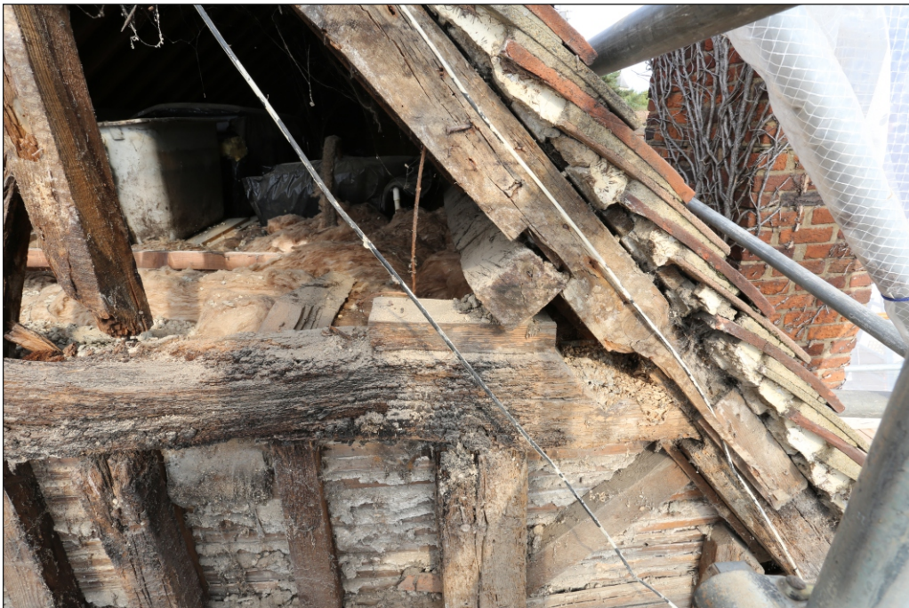
Plate 28: The south-east end of the collar and repositioned purlin in the south-west elevation
