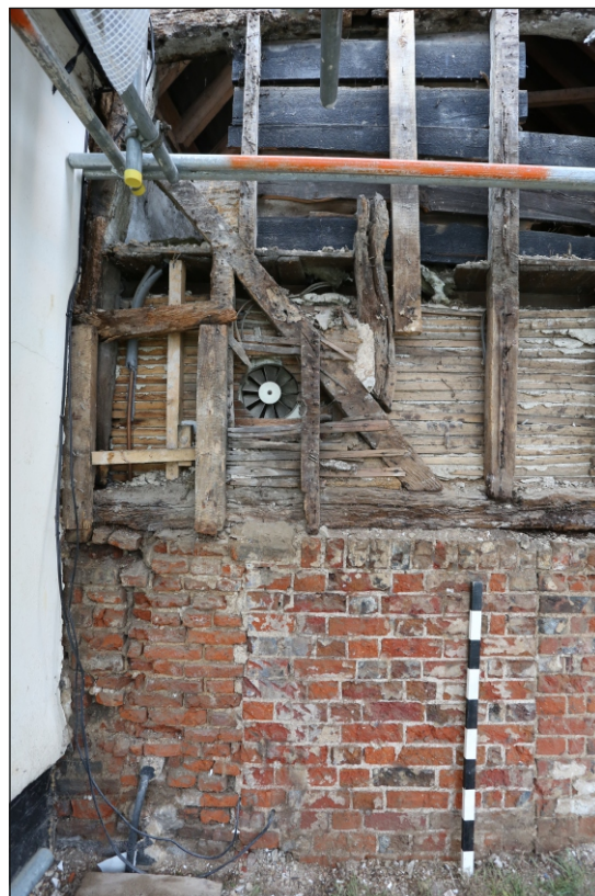
Plate 32: The south-west side of the south-east elevation showing the different phases of brickwork
