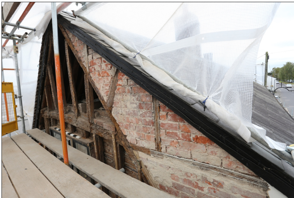
Plate 12: The north-east elevation at collar/roofspace level, viewed from the north-west and showing the brick noggin at the front of the building
