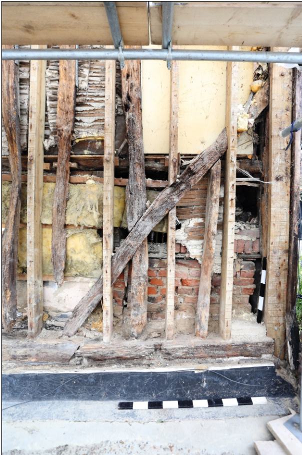
Plate 25: The south-east side of the south-west elevation at ground level showing the reused sill beam timber, south-east down-brace and brickwork behind
