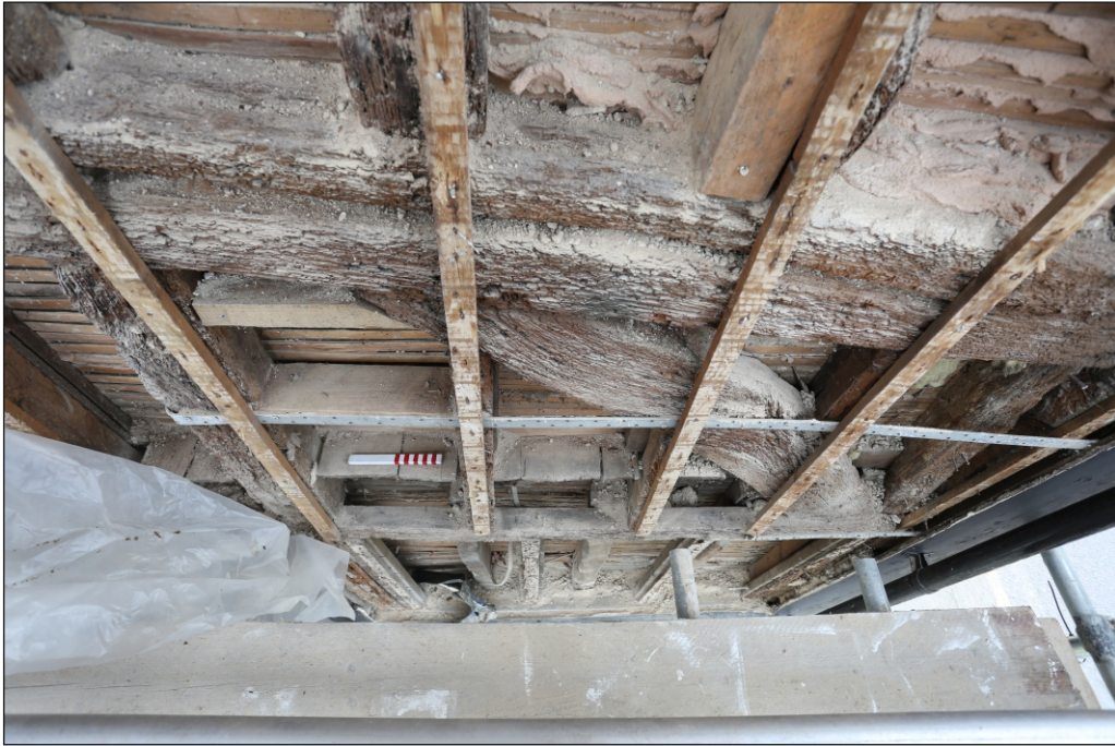
Plate 19: The first floor floorboards visible in the north-east elevation, viewed from above
