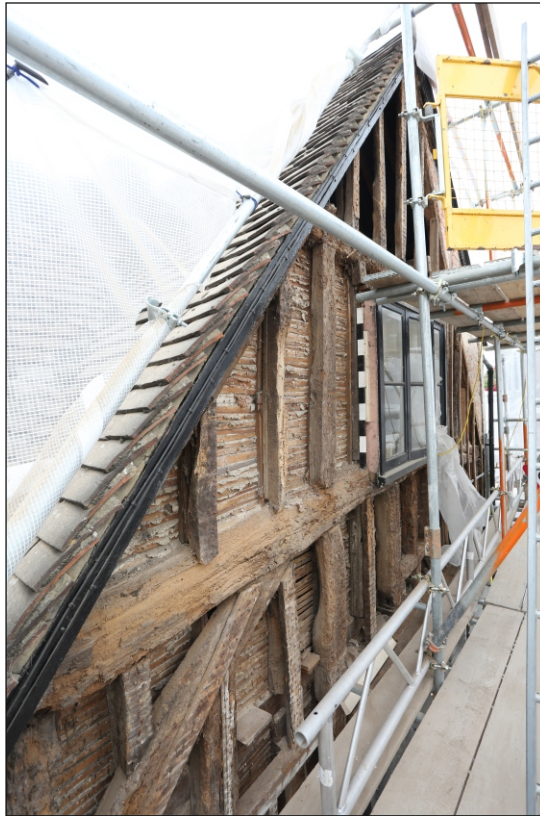
Plate 9: The north-east elevation at tie-beam/ first floor level, viewed from the east
