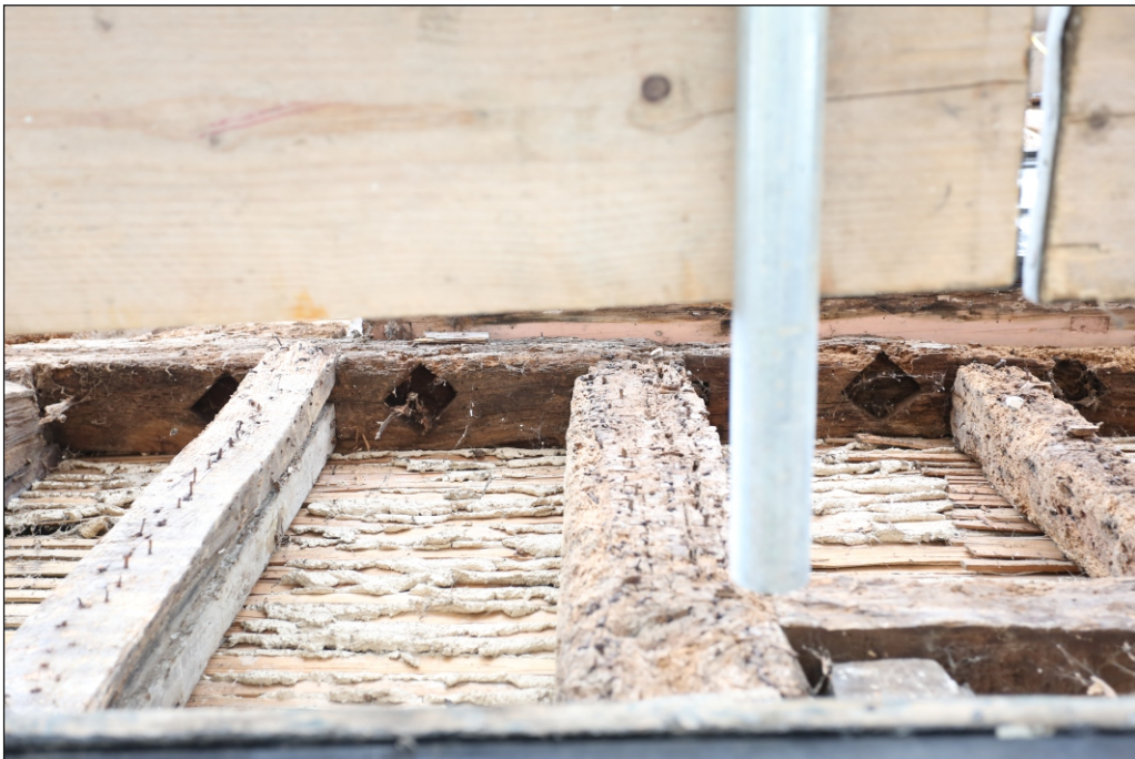
Plate 16: Diamond mortises in the soffit of the tie-beam of the north-east elevation. Probably for a diamond mullion window
