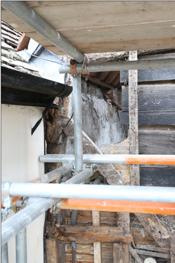
Plate 33: Detail of the south-west jowled post and down brace with an empty half-lap joint in the south-east elevation
