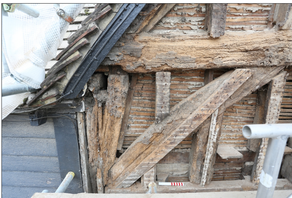
Plate 14: The south-east up-brace, tie beam and jowled post junction in the north-east elevation
