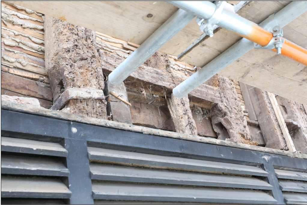
Plate 17: Empty mortices in the studs above the louvre in the north-east elevation. Also note the metal strap.
