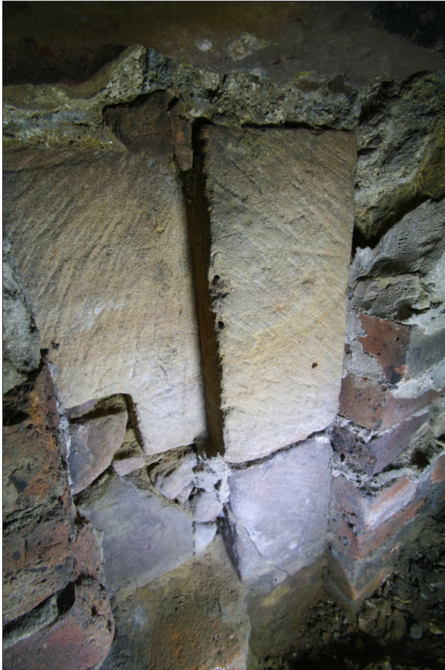
Plate 23: Detail of (109) with a rebated doorway jamb of a possible Saxon Church
