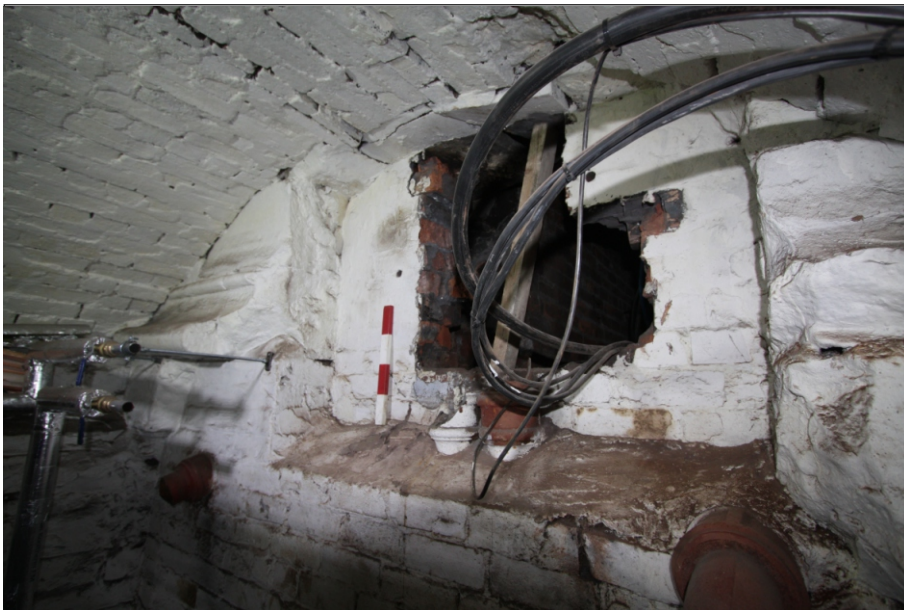
Plate 4: Detail of hole through the inserted brick wall to the west of the Boiler House
