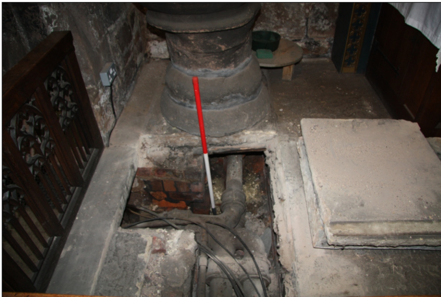
Plate 14: Duct running under the font within the north-east corner of the Jesus Chapel/ South Chapel
