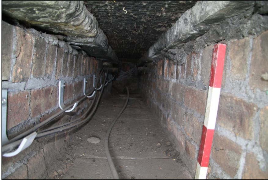
Plate 5: General view of the brick-lined duct with flagstone base and cast-iron grille
