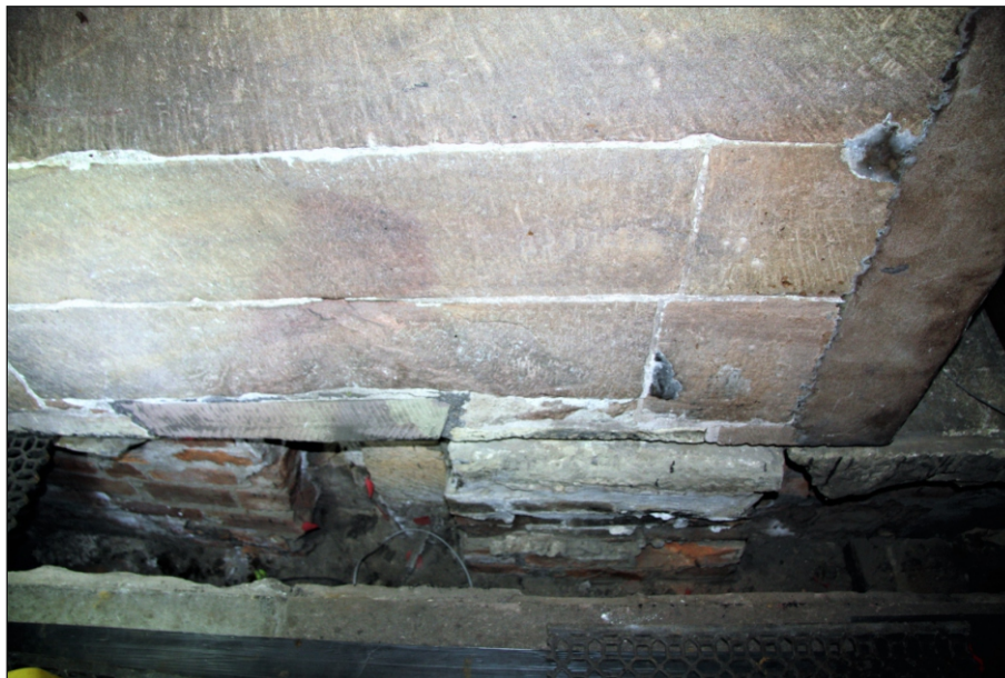
Plate 22 Architectural remains (109) of a possible Saxon doorway under the north-west pier of the crossing/tower
