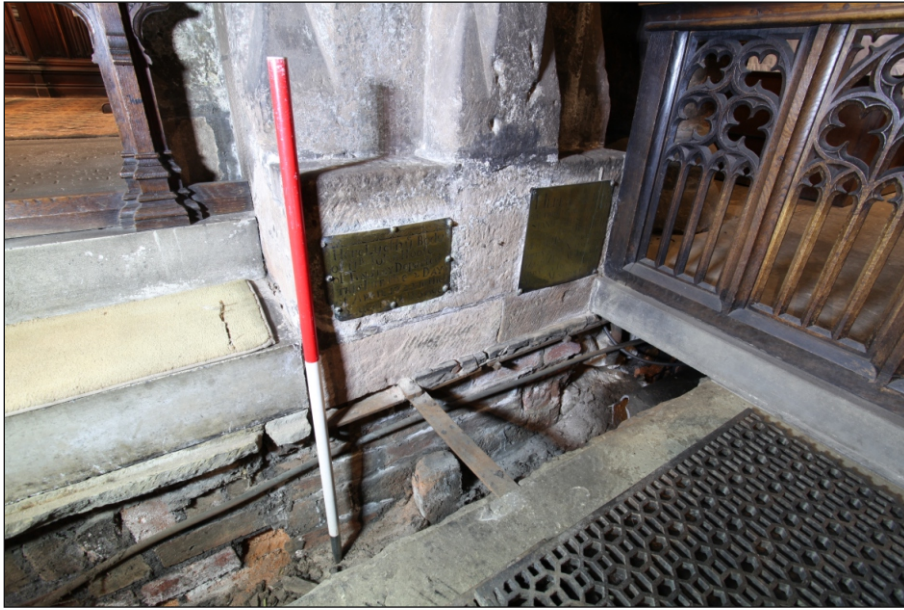
Plate 13: Brickwork of the duct running beneath the south-west pier of the Sanctuary
