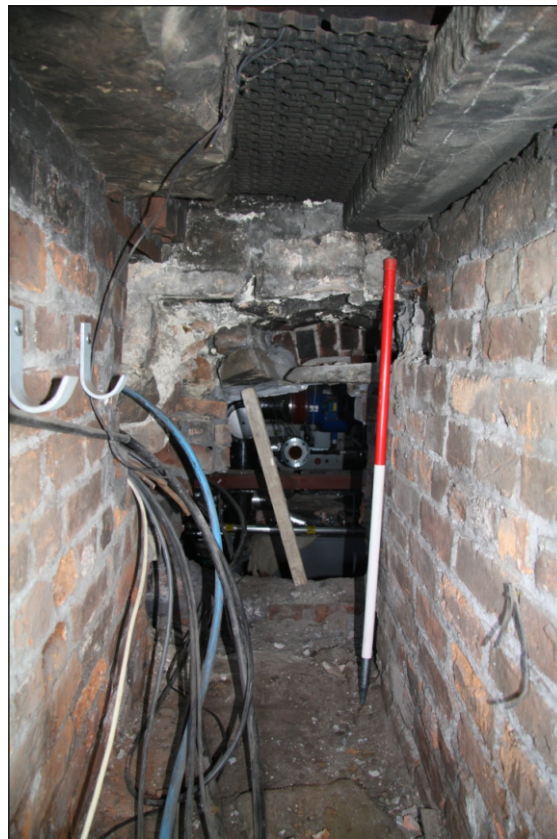
Plate 6: Duct emanating from the boiler house with hole through the inserted wall
