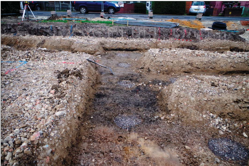
Plate 8: Trench 8 showing foundation trenches and underlying general mixed alluvial deposits and round stone filled piling columns
