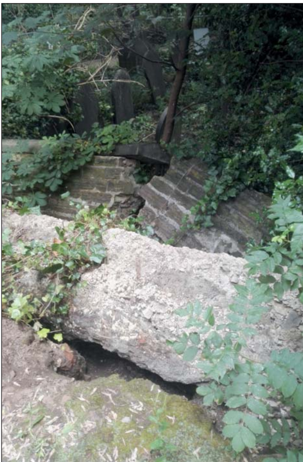
Plate 12: A section of the western retaining wall, within the southwest part of the cemetery, which has collapsed, view from the south
