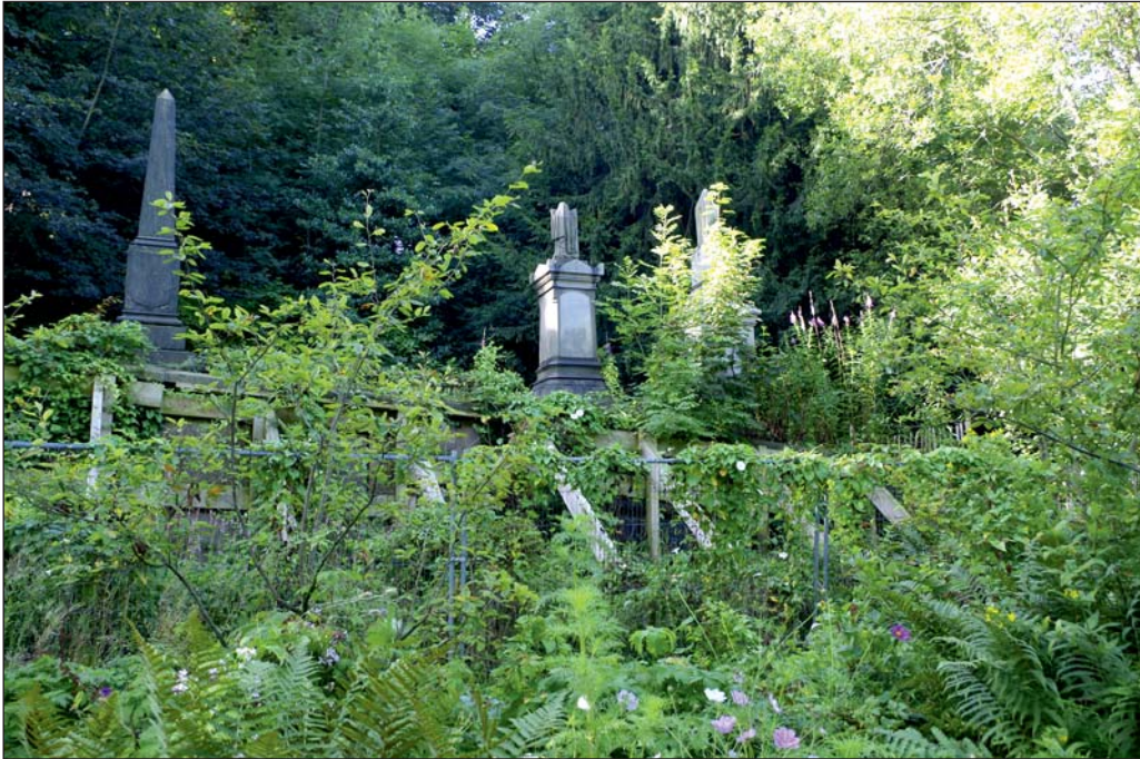
Plate 11: A section of the Grade II listed catacombs which has collapsed, view from the north-west
