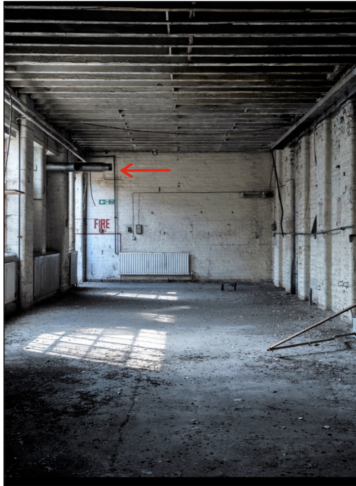
Plate 105: Internal view of Building 17 with a bearing housing wall box within the southern wall (arrow)
