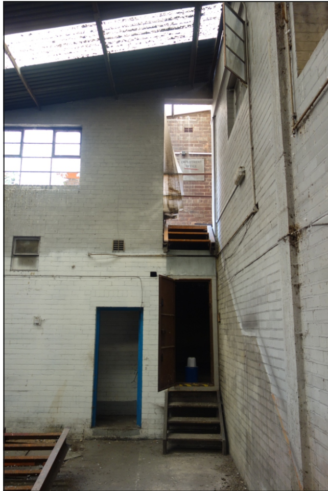
Plate 47: Detail of the south elevation and extension with dismantled staircase to the upper floor
