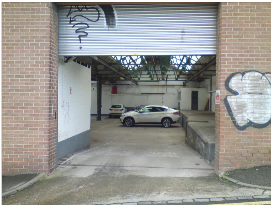
Plate 66: Doorway with roller shutter within the west end of the front elevation of Building 10
