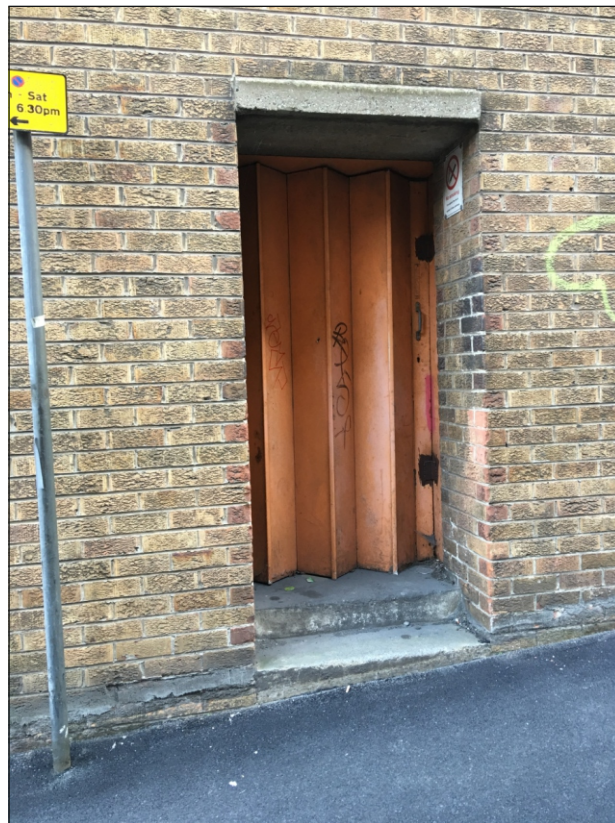
Plate 34: Single concertina doorway to the west of the north elevation of Building 4
