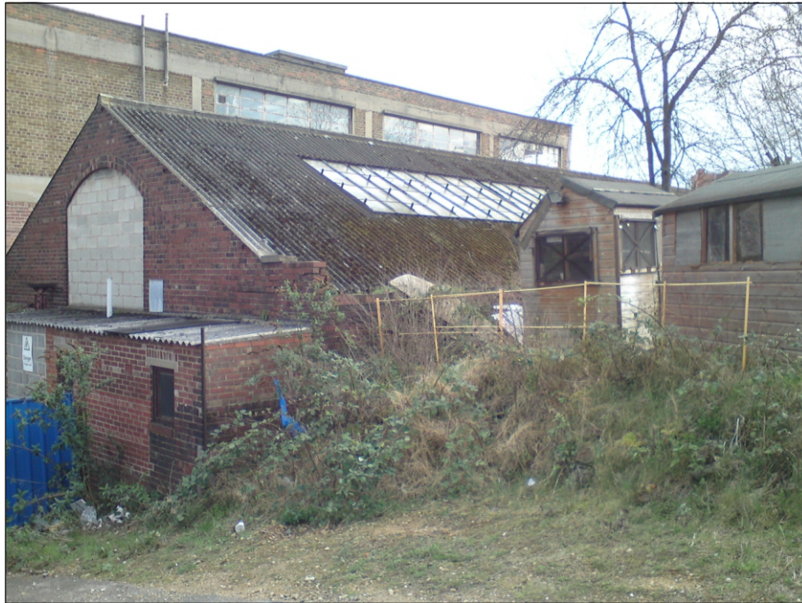
Plate 7: General view of the rear gable elevation of Building 1 facing onto White Croft
