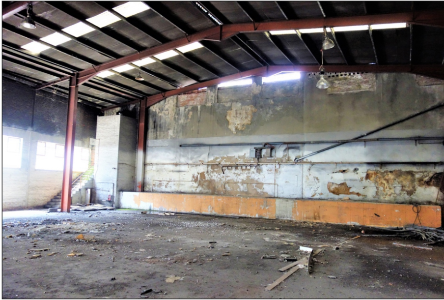
Plate 81: Western wall with blocked-up window openings of a former structure within Building 11 and brick vents towards the northern section of the wall
