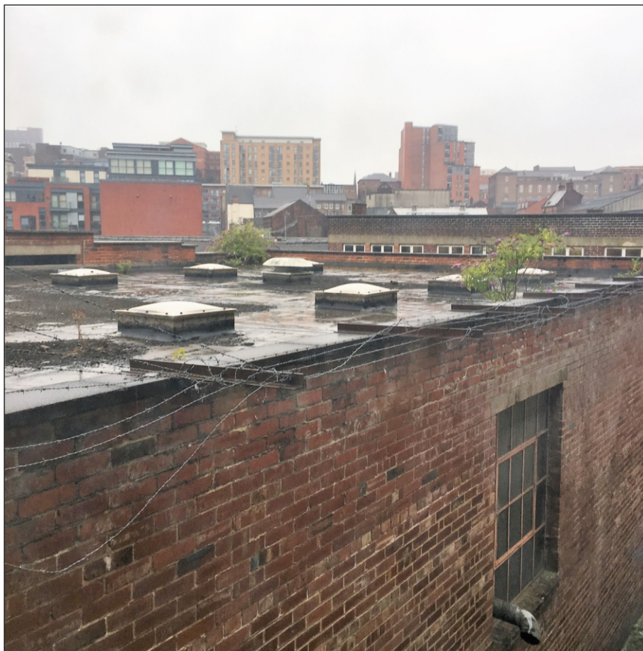
Plate 71: West elevation of Building 11 along an alleyway of the adjacent Croft House
