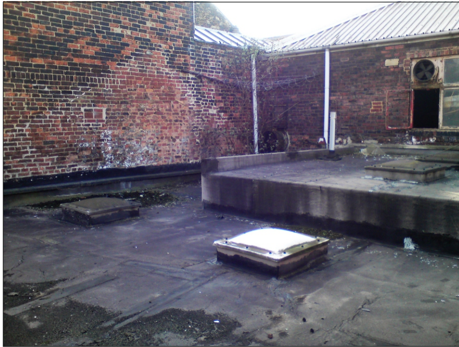
Plate 59: Southern end of the east elevation of Building 8 viewed from the roof of Building 11
