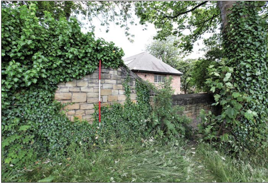
Plate 23: General view of the west face of wall, section E towards section F
