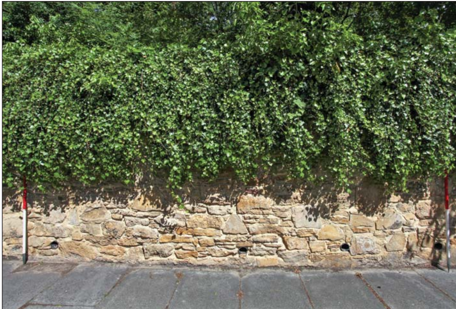
Plate 12: Detailed view of southern boundary wall, showing rebuilt area to the east of section A
