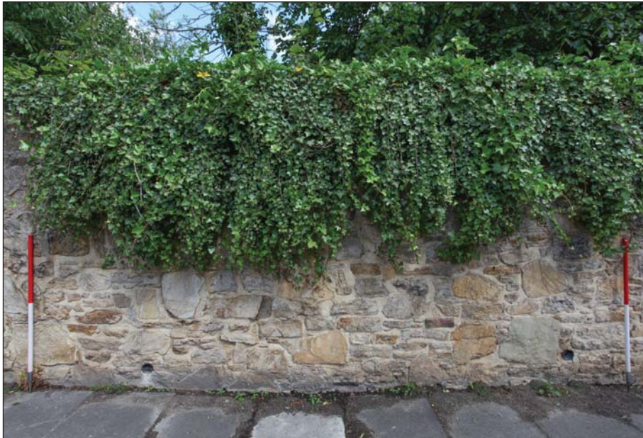
Plate 10: Detailed view of southern boundary wall, showing rebuilt area to the east of section A
