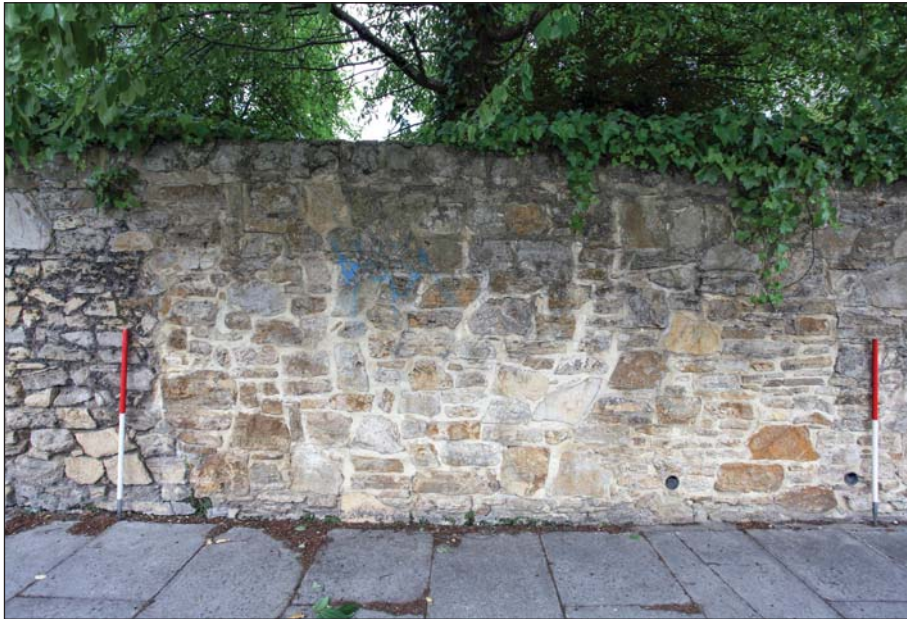
Plate 7: Detailed view of southern boundary wall, showing rebuilt area of section A
