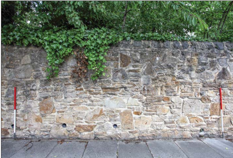
Plate 8: Detailed view of southern boundary wall, showing rebuilt area of section A
