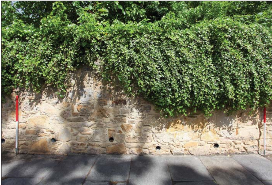
Plate 11: Detailed view of southern boundary wall, showing rebuilt area to the east of section A
