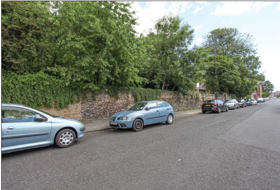
Plate 2: Southern boundary wall along Gray Road to the east of section A
