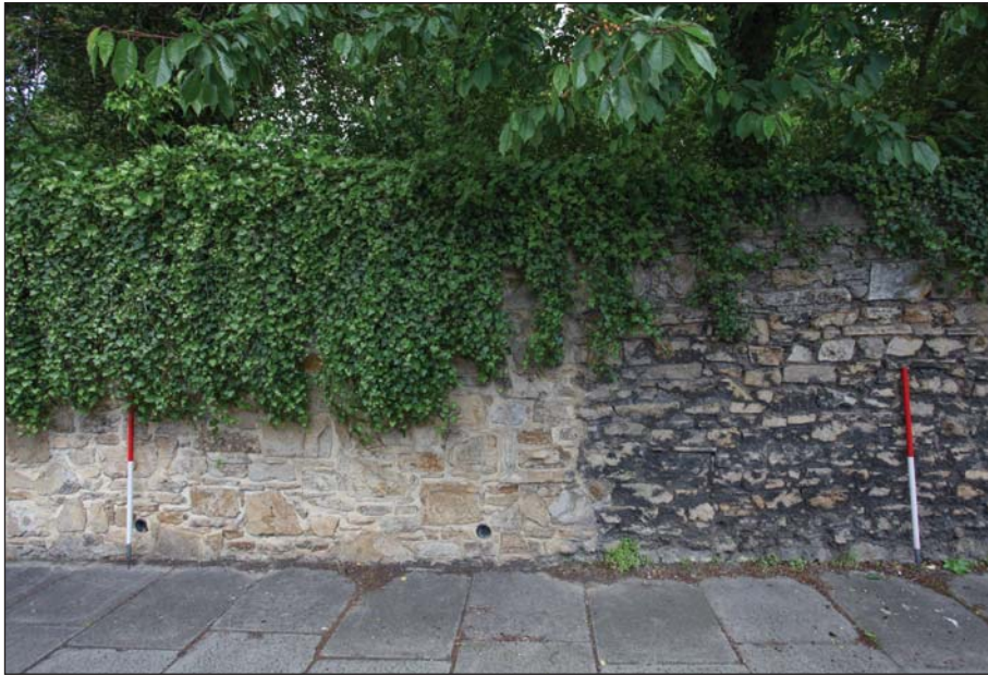
Plate 13: Detailed view of southern boundary wall, showing rebuilt area to the east of section A
