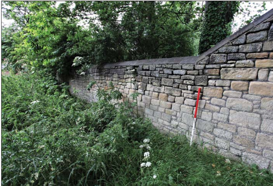
Plate 31: General view of the east face of wall, section E towards section F
