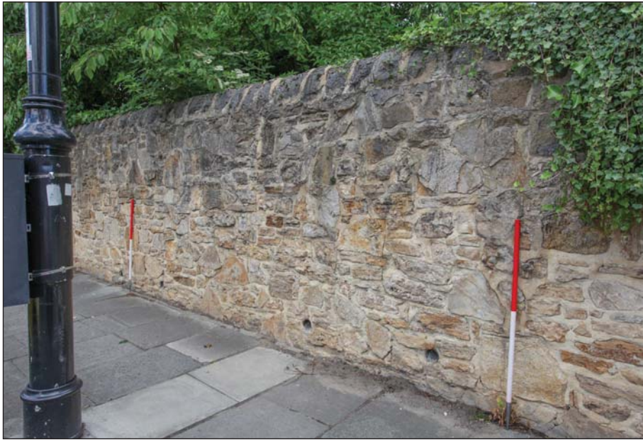
Plate 9: Detailed view of southern boundary wall, showing rebuilt area of section A
