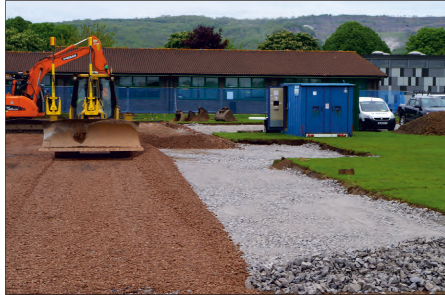
Plate 5: Two types of stone foundation for the pitch, overlying sand/gravel and geotextile
