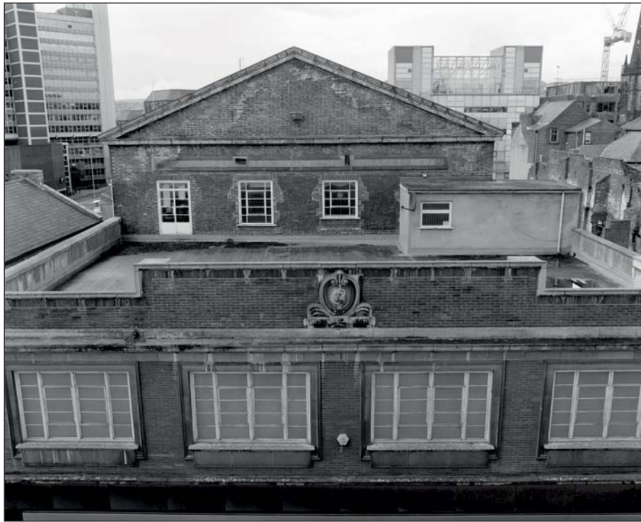
Plate 96: View of parapet and roof space to 'John Lewis', Building 17a from the roof of 'John Lewis', Building 33 (ARCUS 2008)
