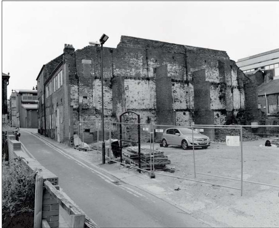
Plate 63: Oblique view of the south facing elevation of the Grade II* Listed Building 'Leahs Yard', Building 13 (ARCUS 2008)
