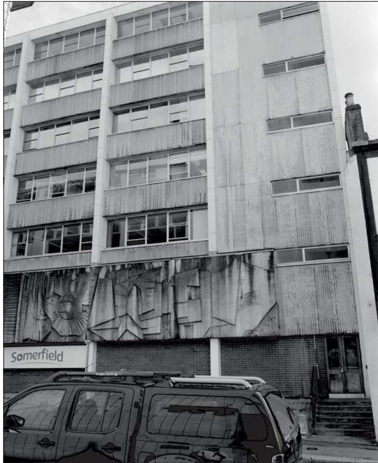
Plate 225: View of the principal west facing elevation of Building 34 at the south end, Burgess Street (ARCUS 2008)
