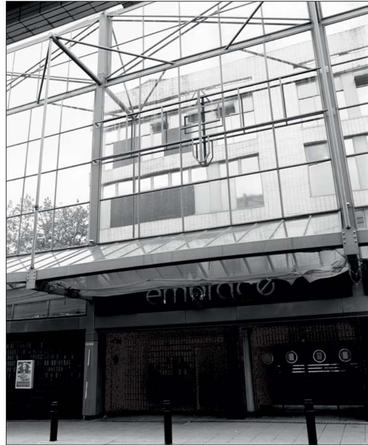
Plate 230: View of the principal west facing elevation of Building 35 at the central section, Burgess Street (ARCUS 2008)
