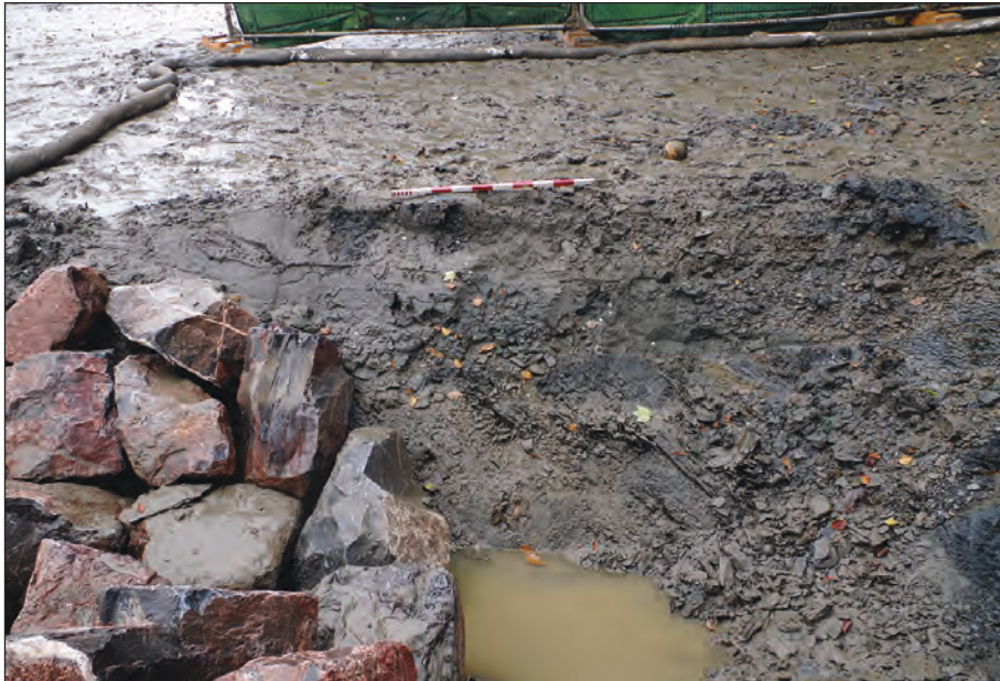
Plate 2: South-east facing view of excavation on the foreshore for construction of the new surface water outfall (scale: 1 x 1 m)
