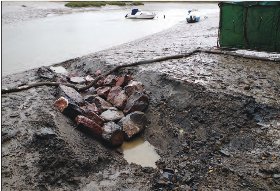
Plate 1: East facing view of excavation on the foreshore for construction of the new surface water outfall (scale: 1 x 1 m)
