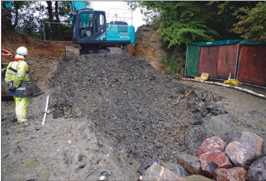
Plate 3: South-east facing view of excavation through bedrock geology / extant trackway within footprint of headwall and inspection chamber
