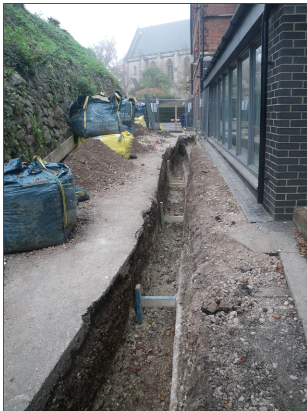
Plate 10: Section of the cable trench at the location of layer 150, view from the south-east
