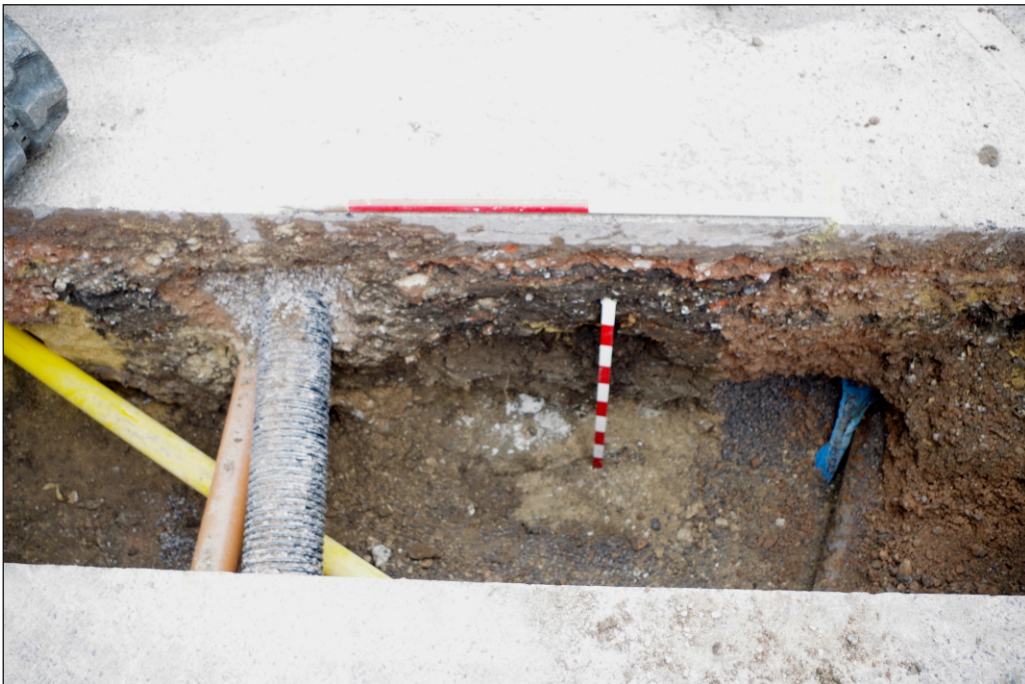
Plate 8: West facing representative section of heavily truncated wall footing 118 (1 x 1 m, 1 x 2 m)
