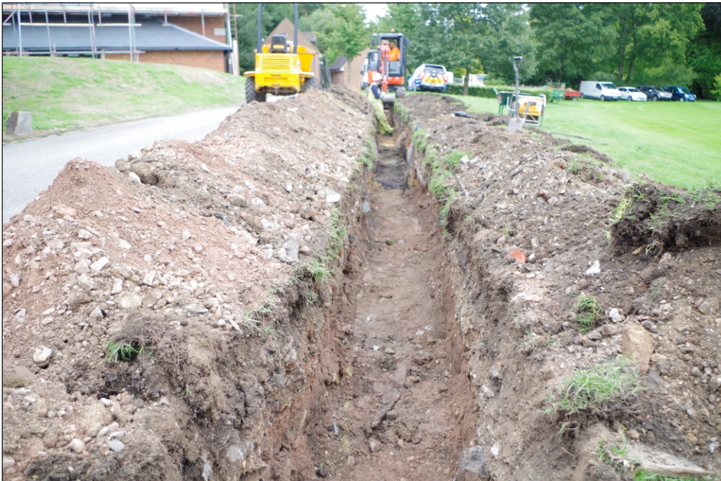
Plate 3: Section of the cable trench located south of language centre, view from the west
