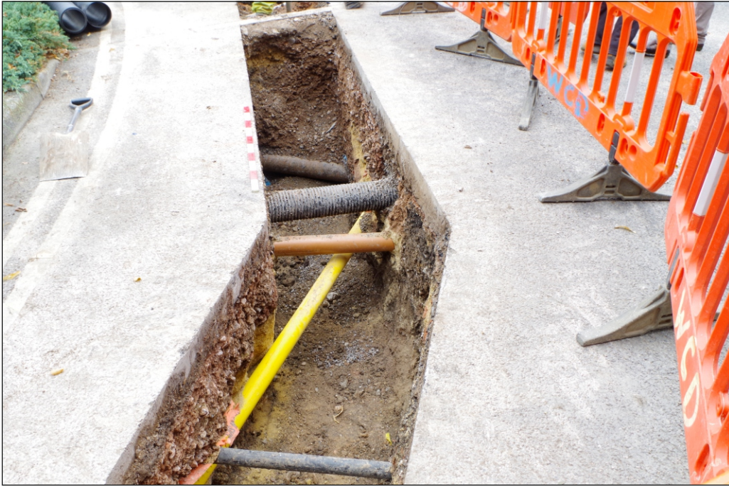
Plate 1: Section of the cable trench in tarmac area, located west of Heywood Block, view from the north
