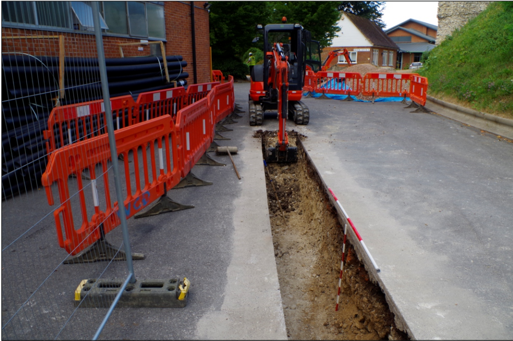
Plate 5: North facing section of cable trench with location of wall footing 105 (1 x 1 m, 1 x 2 m)
