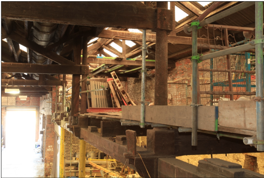
Plate 78: General view of FF6 above the east aisle of G6, showing king post roof trusses, looking north-east (Film 2.05)
