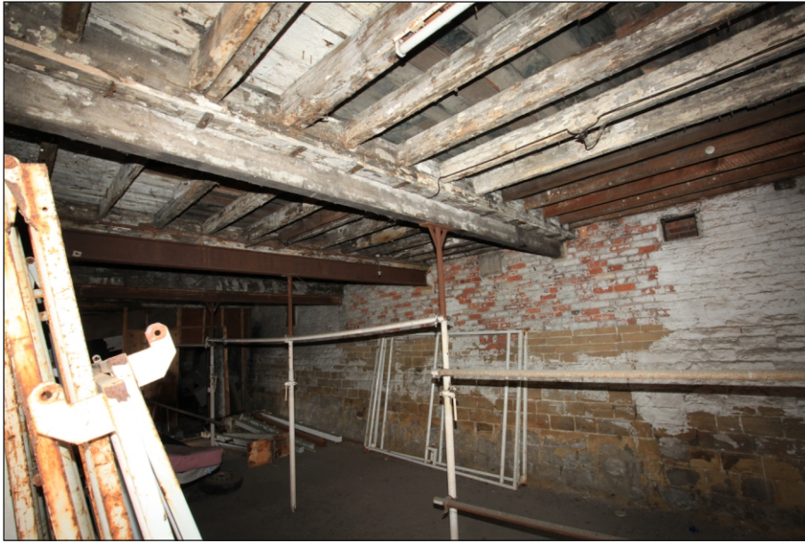
Plate 19: General view of G19 showing wall box and timber ceiling beams, looking south-west (Film 2.18)
