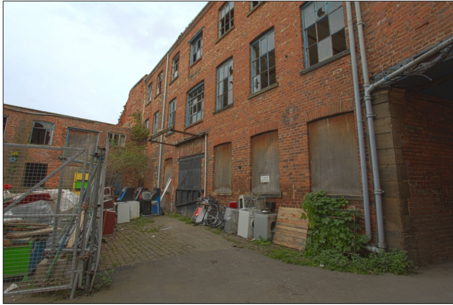
Plate 3: Oblique view of the south elevation of the north-east range of Low Hall Mills and the east range of the Site at the north end (Film 3.02)
