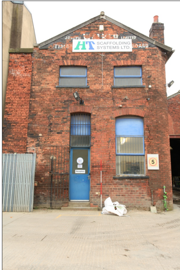
Plate 29: View of the north elevation of the central range showing historic signage (Film 4.01)
