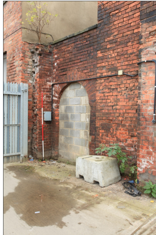
Plate 28: View of blocked doorway to the inaccessible gap between the central and east ranges, showing chimney stack and truncated wall (Film 2.07)
