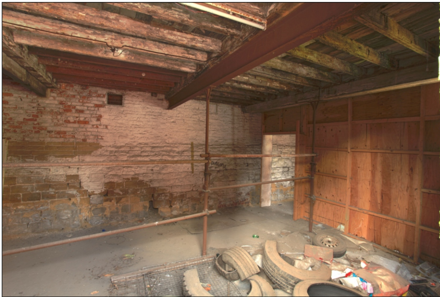
Plate 20: General view of G19 showing wall boxes, stud partition and timber ceiling beams, looking north-west (Film 2.19)
