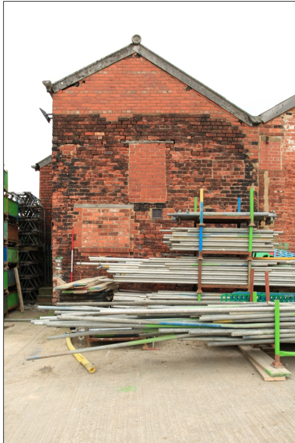
Plate 35: Detail of the west elevation of the west ranges at the north end, showing blockings (Film 1.29)
