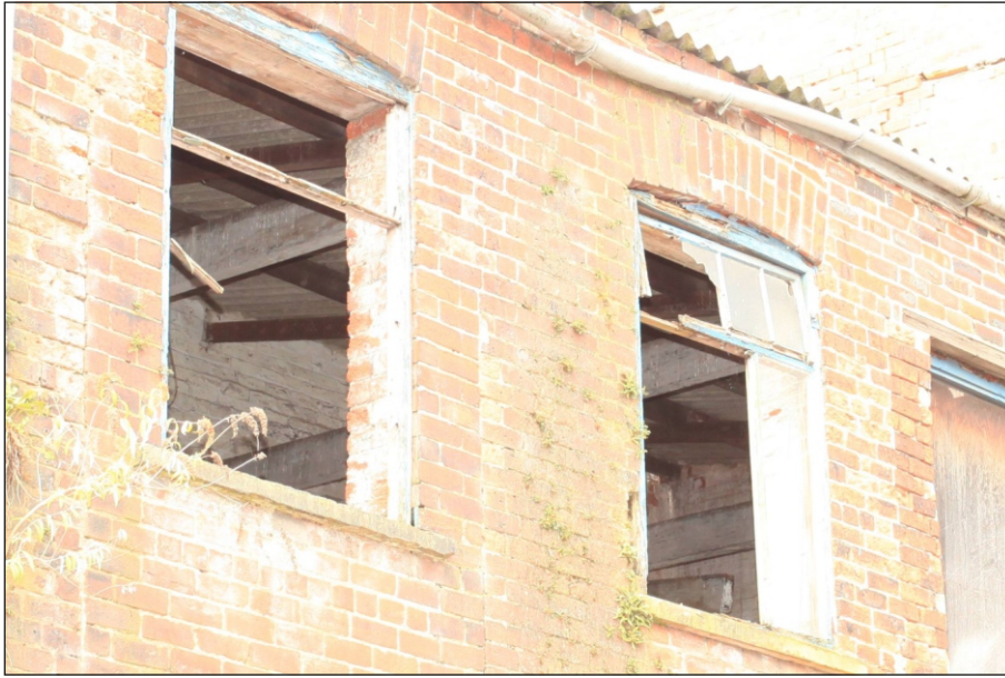
Plate 23: View of the first floor level through windows showing timber beams and modern roof structure, looking north-west (Film 2.12)
