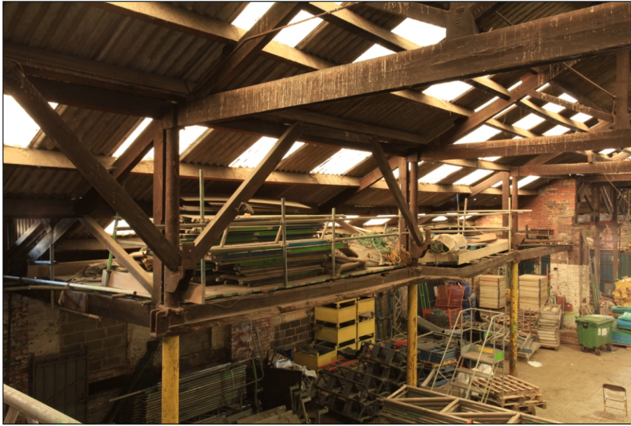
Plate 77: General view of FF5 above the west aisle of G6 showing cast-iron columns and bolting faces, looking north-west (Film 2.04)
