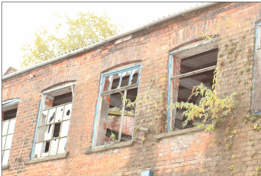
Plate 22: View of the first floor level through windows showing timber beams and modern roof structure, looking south-west (Film 2.11)
