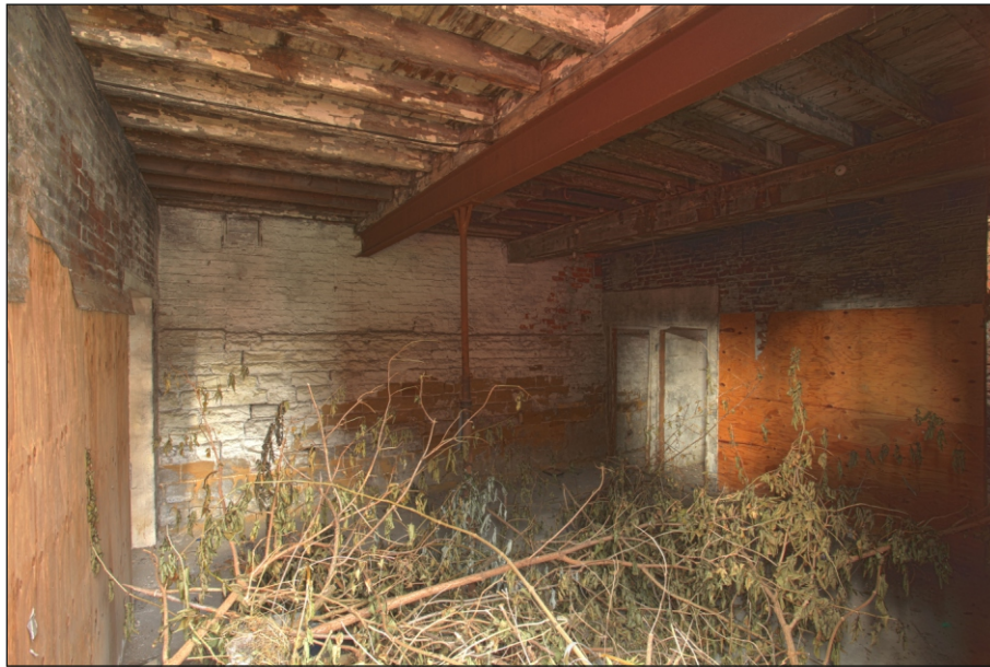
Plate 21: General view of G18 looking north-west showing wall box, cupboards and timber ceiling beams, with a staircase in the north-east corner leading to the first floor (Film 2.20-21)
