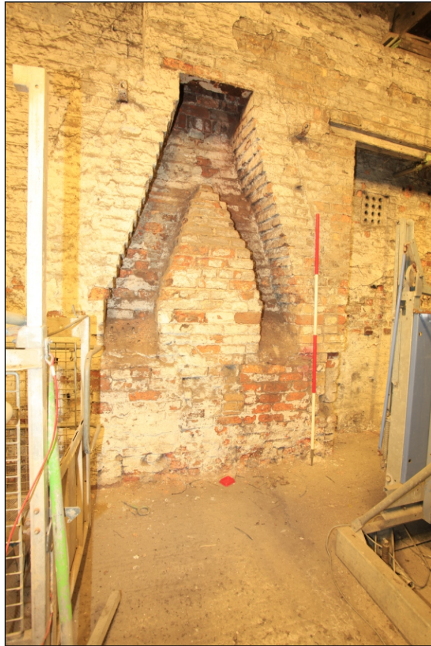
Plate 72: Detail of a typical flue in the east wall of G6 (Film 2.27)
