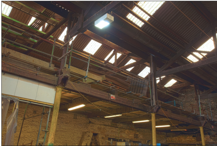
Plate 79: General view of FF6 above the east aisle of G6, showing king post roof trusses and sky lights, looking south-east (Film 2.24)
