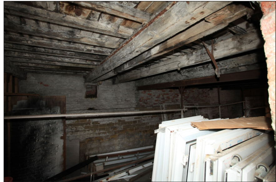
Plate 18: General view of G19 showing wall box and timber ceiling beams, looking north-west (Film 2.17)
