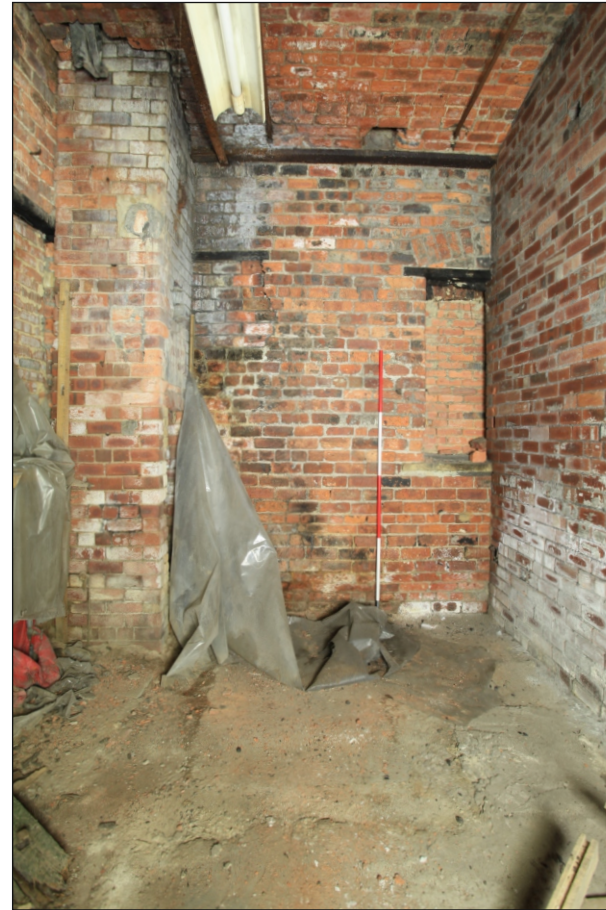
Plate 8: General view of G23, looking south, showing blocked windows and chimney stack (Film 1.32)
