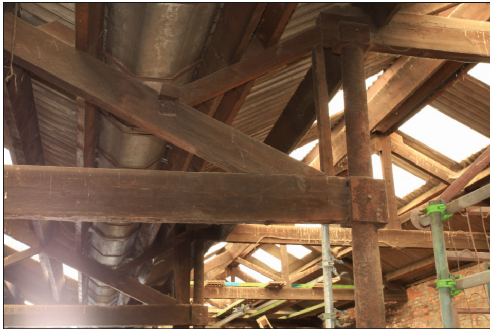
Plate 83: Detail of junction of roof trusses from central aisle of G6 to FF6 (Film 2.01)
