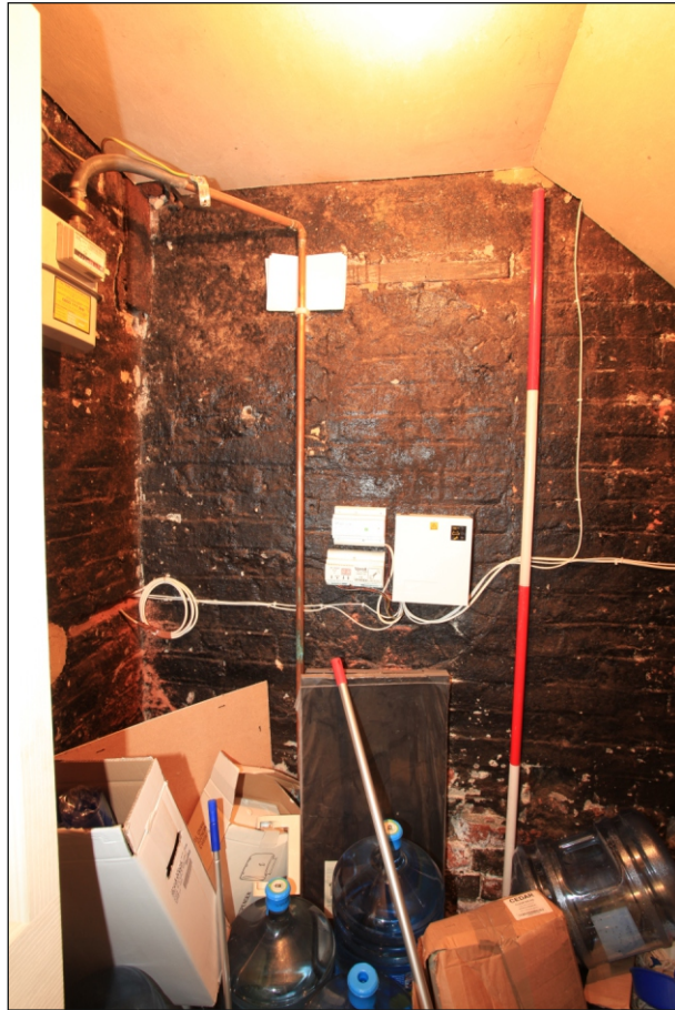
Plate 85: General view of under stairs cupboard G10 looking east, showing blocked window (Film 1.05)
