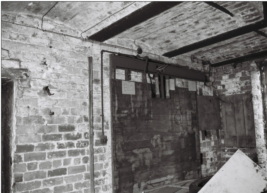
Plate 12: General view G21, looking north-east (Film 3.08)
