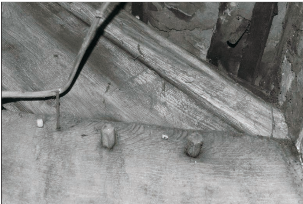
Plate 66: View of the timber truss, showing joint of tie beam and principal rafter with construction marks, F1, Building 1 (Film 03.16)
