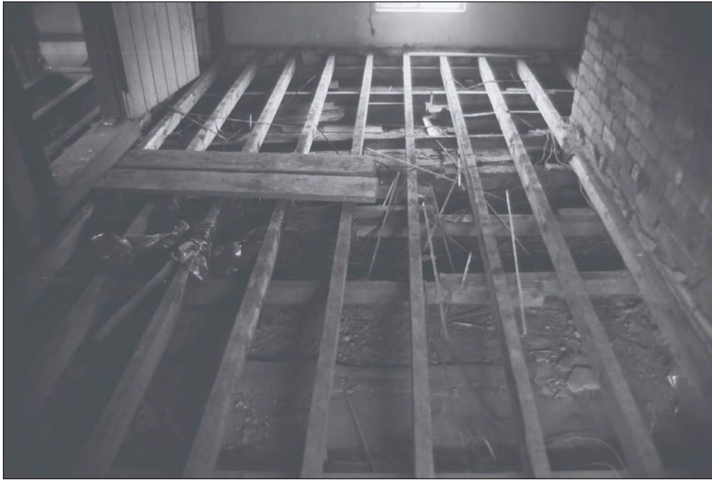
Plate 229: General view of lifted floor boards, F1, Building 2 showing limeash floor beneath (Film 40.05)
