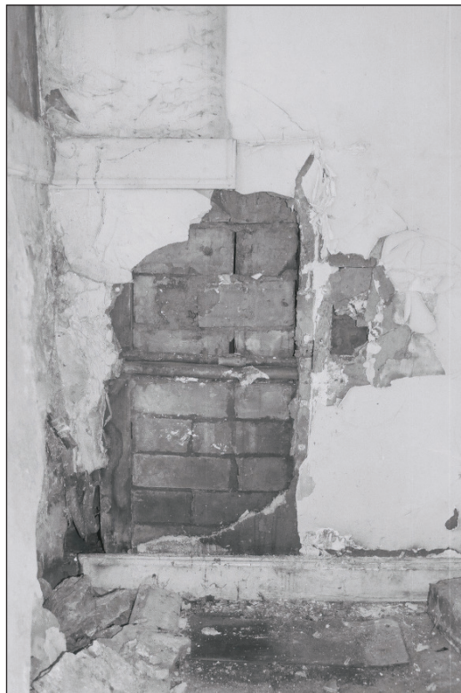
Plate 147: Detail of exposed timber and brick partition between G1 and G4, Building 2 (Film 12.27)
