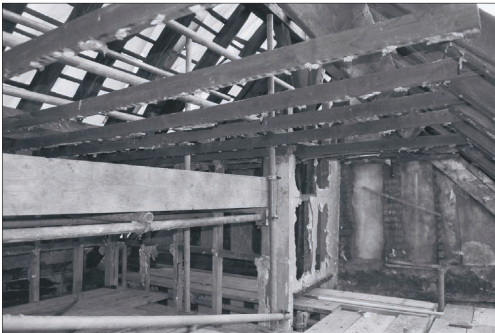
Plate 218: General view of ceiling and roof structure during watching brief, F3, Building 2 (Film 41.09)
