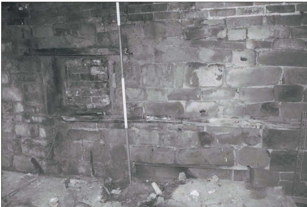
Plate 50: Detail of blocked window and inserted RSJ lintel, east wall of F1, Building 1 (Film 18.36)
