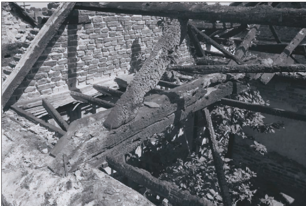
Plate 321: Detail of ceiling joists and tie beam, south end of Building 4 (Film 25.23)
