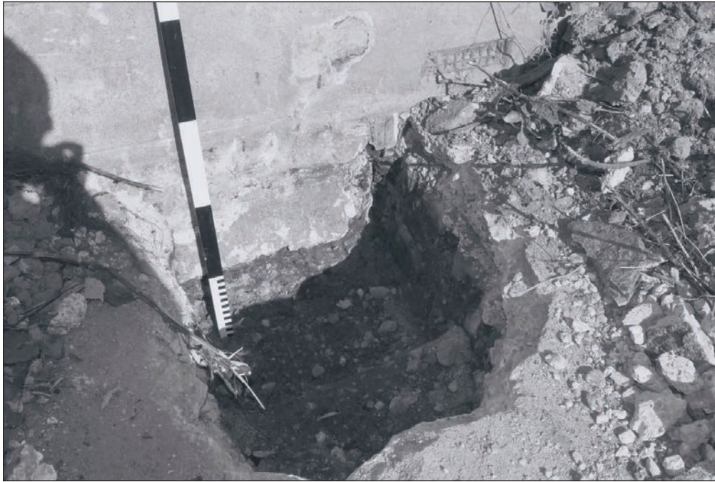
Plate 120: General view of Test Pit 9, against the south elevation of Building 2 (Film 35.24)
