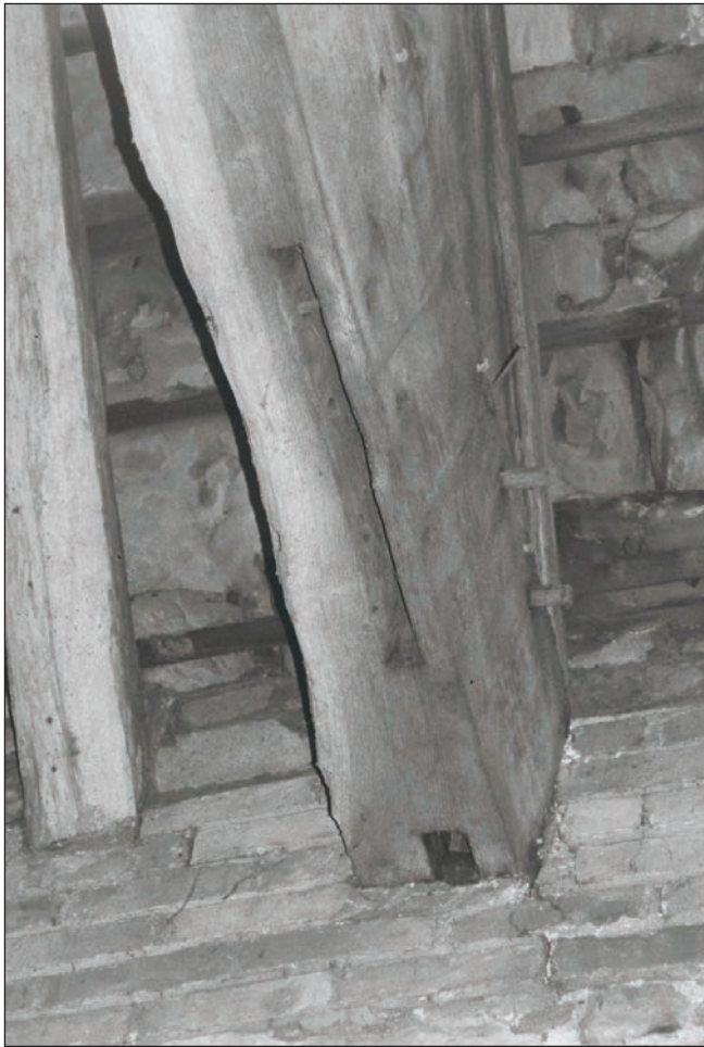
Plate 61: Detail of timber truss tie beam, with empty mortice joints and junction with wall, F1, Building 1 (Film 24.15)
