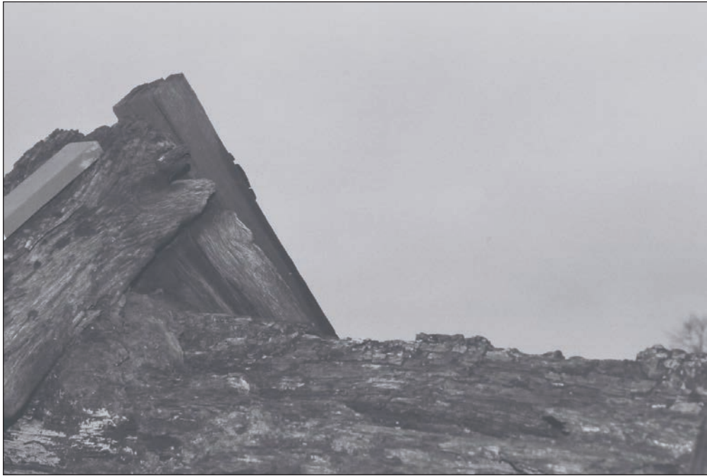
Plate 91: Detail of the ridge of the roof, Building 1, during the watching brief (Film 39.28)
