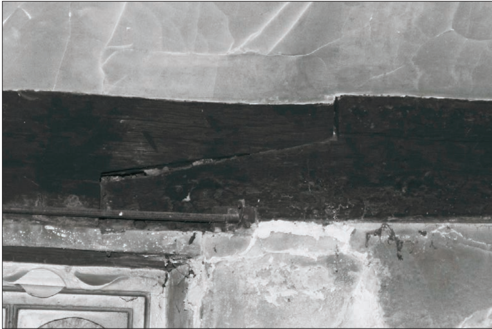
Plate 213: Detail of scarf joint within wall plate of south wall, F3, Building 2 (Film 05.14)
