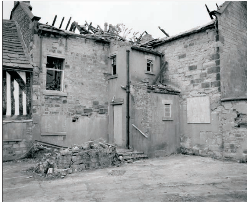
Plate 247: General view of the east elevation of Building 4 and north elevation of Building 3 (Film 08.10)
