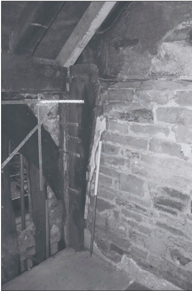
Plate 199: Detail of the northeast corner of F1 showing the exposed original timber post and join with the wall plate and arched brace, Building 2 (Film 43.26)
