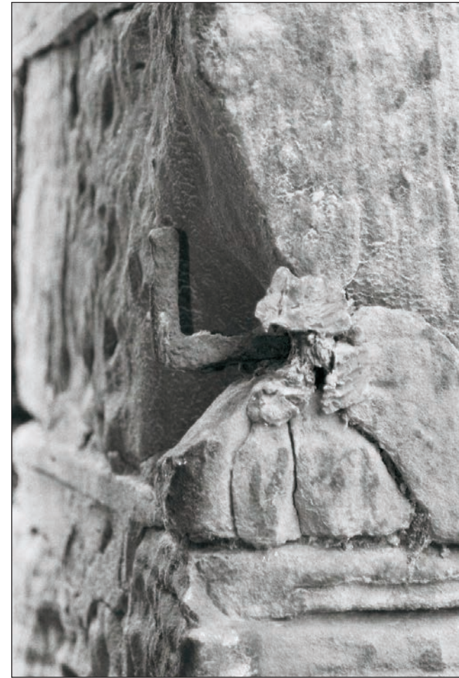
Plate 105: Detail of iron hook within south corner of east elevation of Building 2 (Film 04.32)
