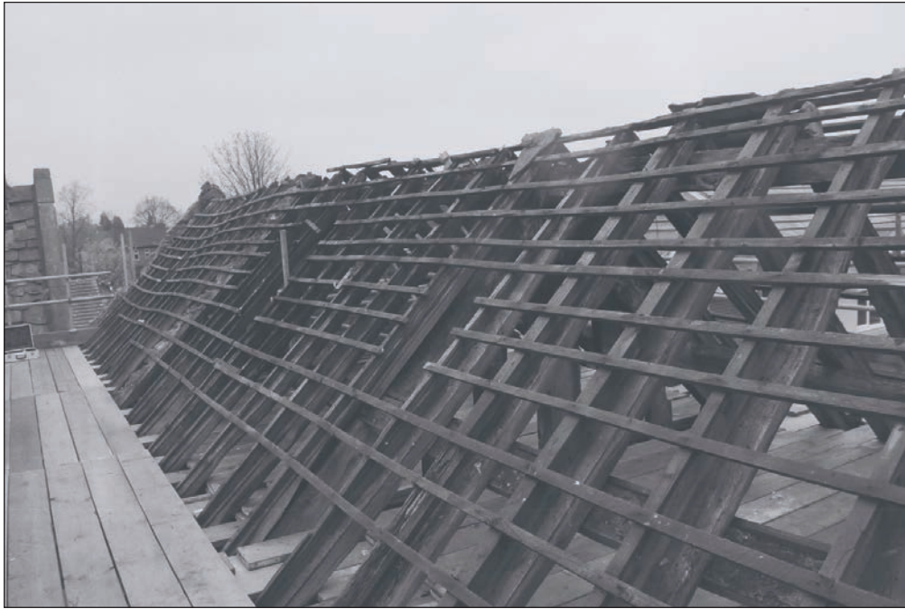
Plate 87: General view of the roof structure of Building 1 during the watching brief (Film 39.16)
