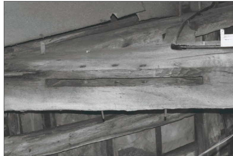
Plate 62: Detail of timber truss tie beam, with empty mortice joints on underside, F1, Building 1 (Film 24.17)
