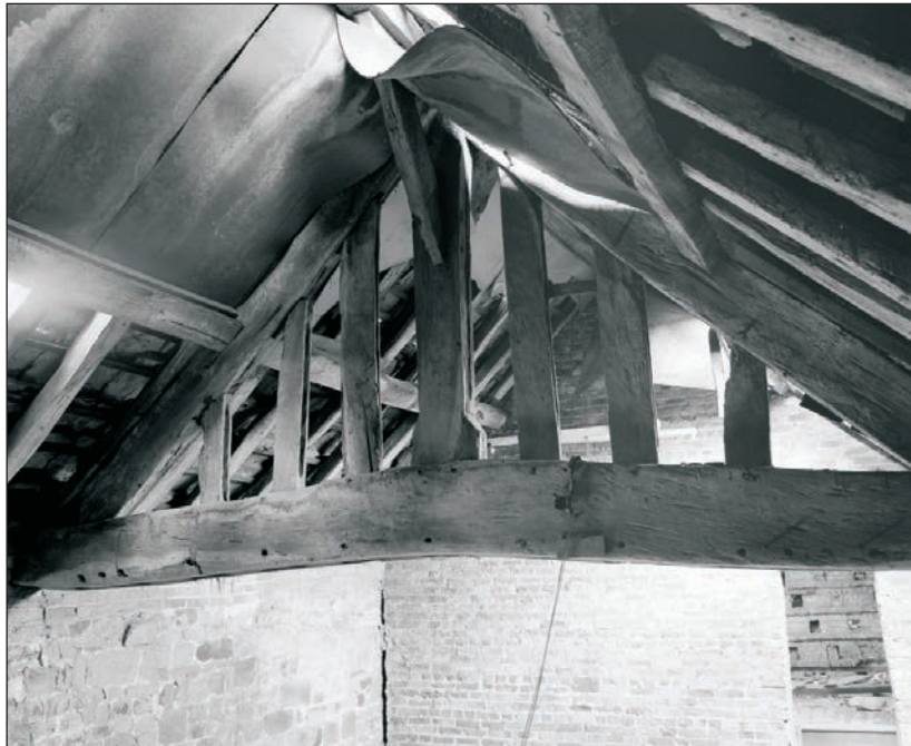
Plate 56: View of the timber truss, showing the lower face, F1, Building 1 (Film 19.10)
