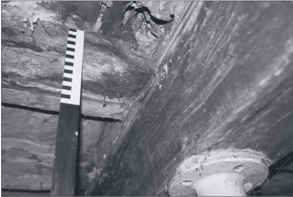
Plate 144: Detail of join of exposed joists with timber beam, G1, Building 2 (Film 35.37)
