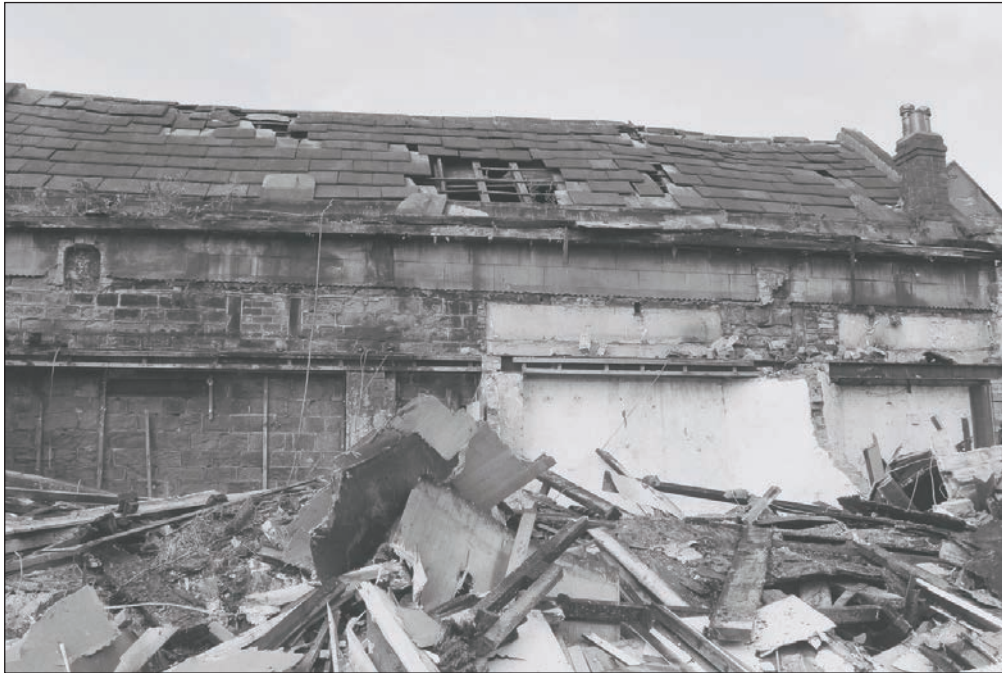
Plate 24: General view of the east elevation of the barn, Building 1 after the demolition of the modern extension (Film 18.12)
