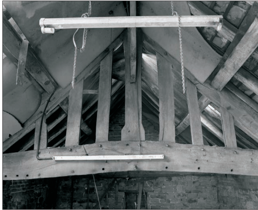
Plate 55: View of the timber truss, showing the fair or upper face, F1, Building 1 (Film 19.08)
