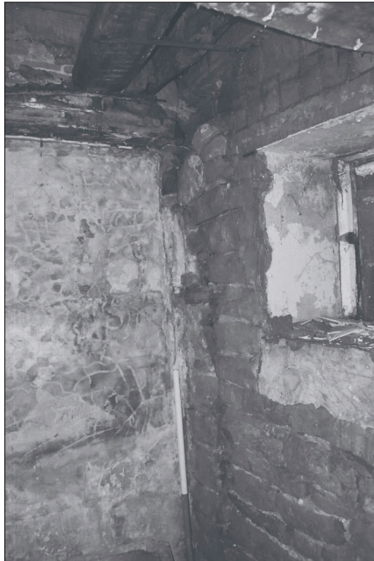
Plate 176: Detail of exposed southeast corner of G1 showing removed timber post, replaced with stone, Building 2 (Film 42.27)
