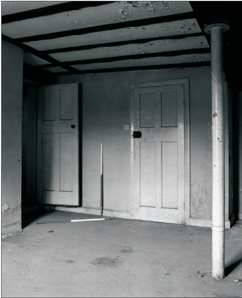
Plate 124: General view of G1, Building 2, showing cast iron column and doorways to G2 and G3 (Film 13.10)
