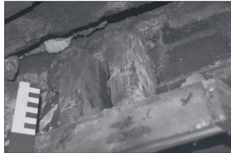
Plate 159: Detail of mortice for cross beam at the top of the exposed south post, G4, Building 2 (Film 30.08)
