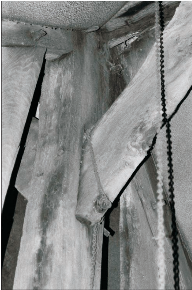
Plate 67: Detail of timber truss, showing joint of ridge brace with King-Post, F1, Building 1 (Film 03.18)
