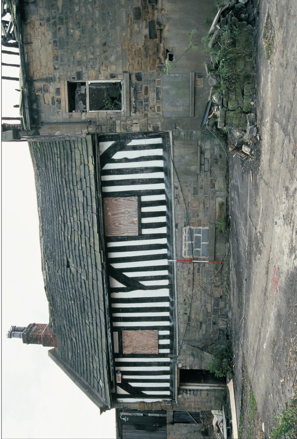
Plate 7: General view of the northern timber framed facade of Hanson House (Building 2) (Colour Slide 02)
