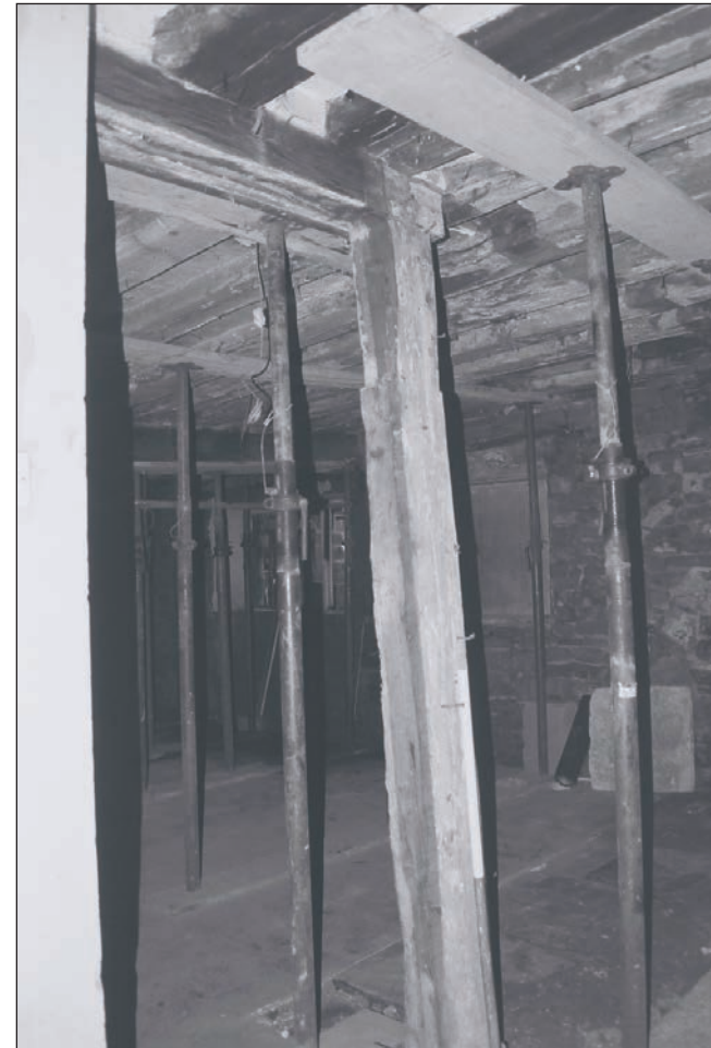
Plate 165: View of exposed timber framing of doorway between G3 and G1, and position of former removed partition between G4 and G1, Building 2 (Film 42.06)
