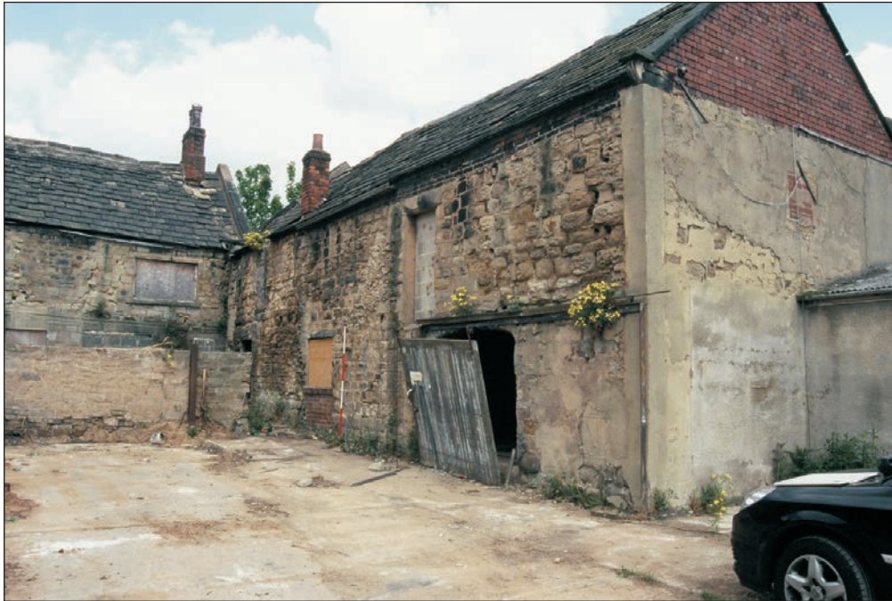
Plate 3: General view of the western facade of the barn (Building 1) (Colour Slide 05)
