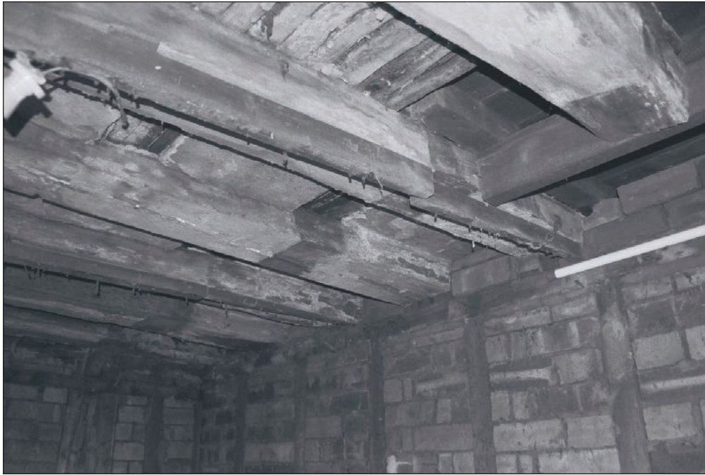
Plate 162: View of scar within exposed ceiling delineating position of former partition between exposed timber posts, G4, Building 2 (Film 30.18)
