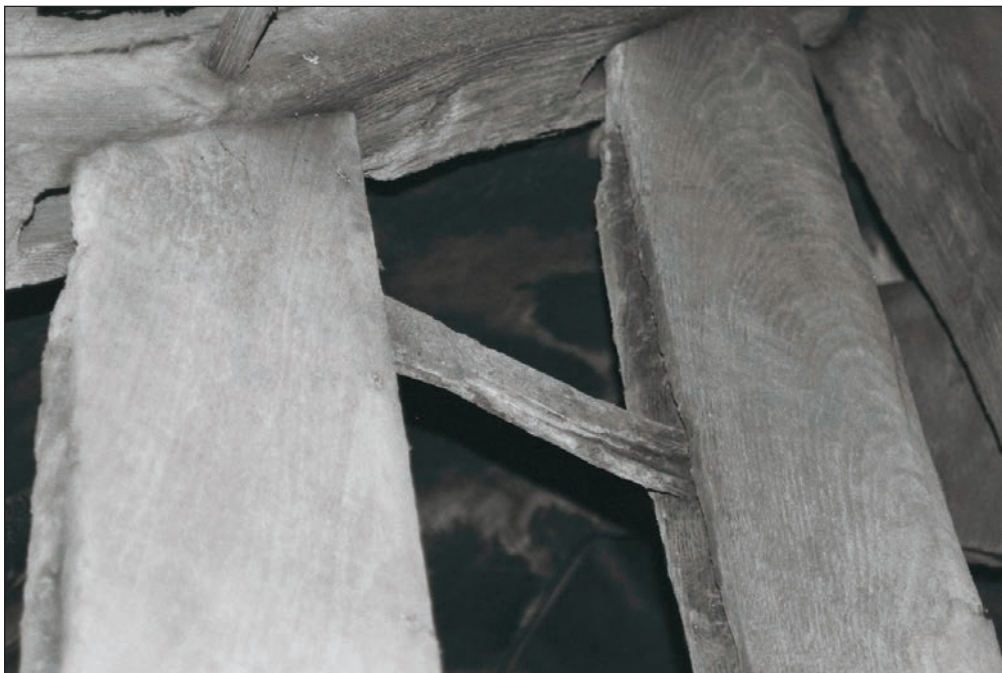
Plate 70: View of the timber truss, showing original lath infill and grooves within uprights for removed laths, F1, Building 1 (Film 06.14)
