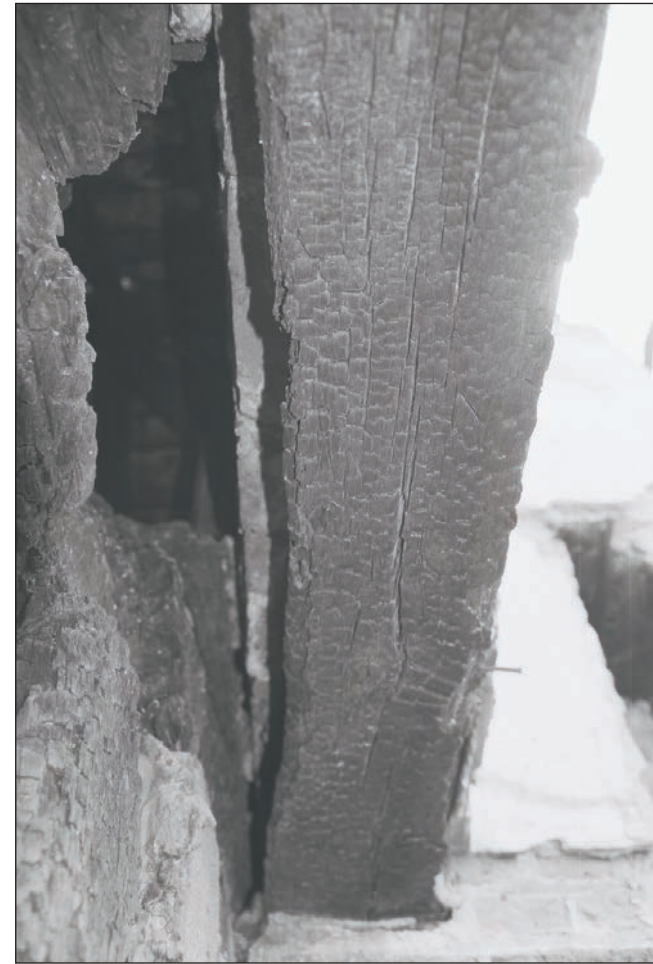
Plate 303: View of timber beam and join between Buildings 2 and 3 from F7, Building 3 (Film 12.02)
