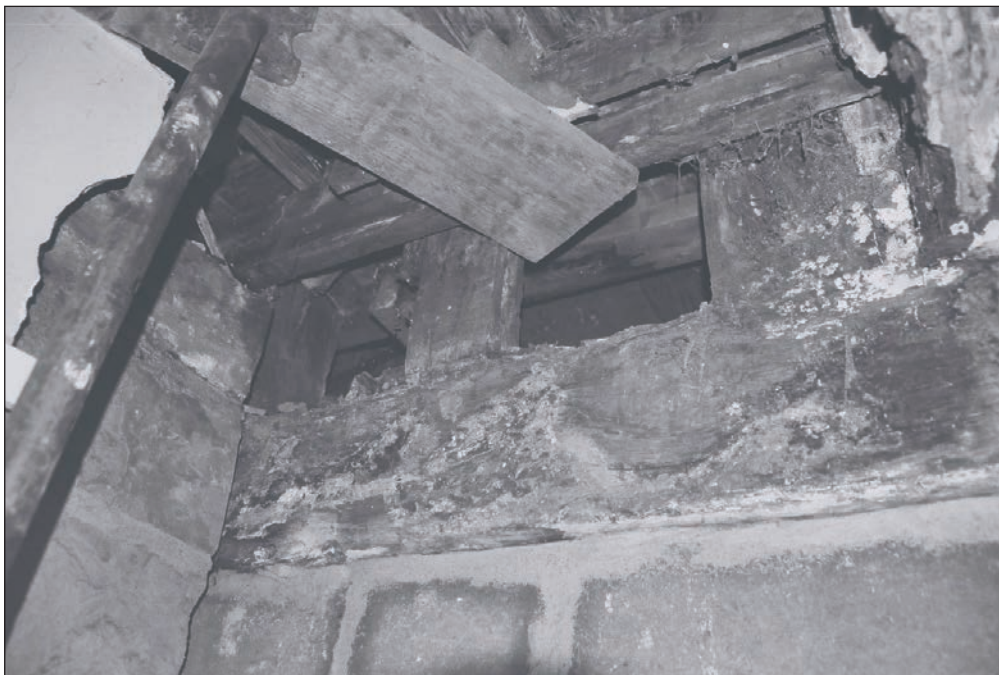
Plate 173: Detail of exposed timber framing above tie beam across G1 and join with the original north central timber post, G2/G1, Building 2 (Film 42.18)
