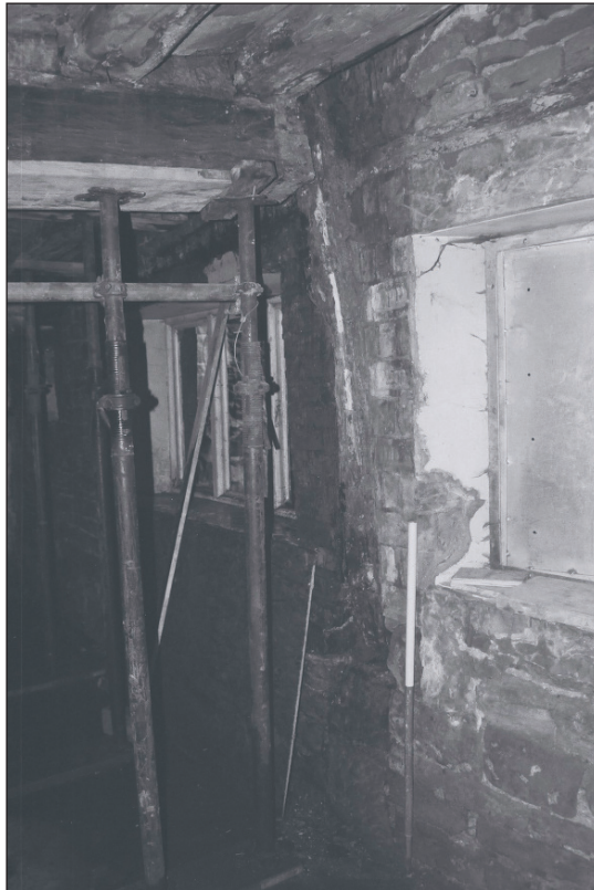
Plate 175: Detail of exposed original southern central timber post, showing stone plinth/pad, G1, Building 2 (Film 42.23)
