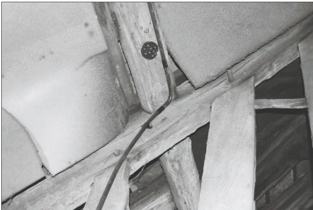
Plate 64: View of the timber truss, showing joints of principal rafters and purlins, F1, Building 1 (Film 03.06)
