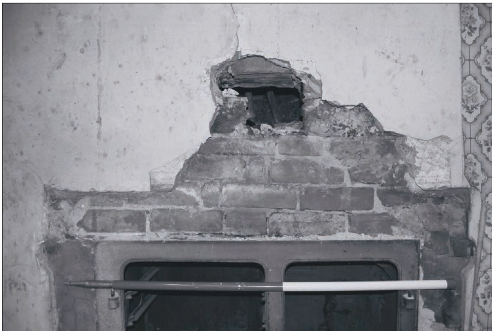
Plate 297: Detail of range and chimney breast, room G7, Building 3, showing range to be later insertion (Film 30.35)
