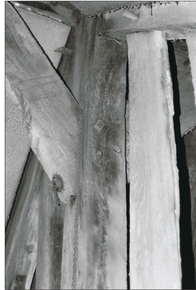
Plate 68: Detail of timber truss, showing joint of ridge brace with King-Post, F1, Building 1 (Film 03.19)
