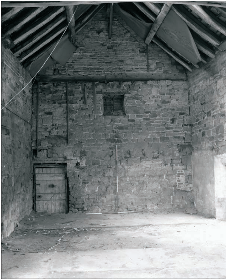
Plate 29: General internal view of G1 and F1 after the removal of modern shelving, Building 1 (Film 22.09)
