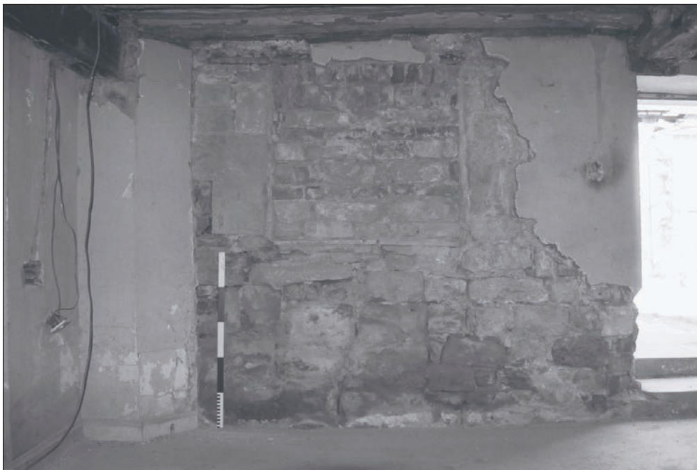
Plate 133: Detail of exposed blocked window within the north wall of G1, Building 2, during watching brief (Film 35.31)
