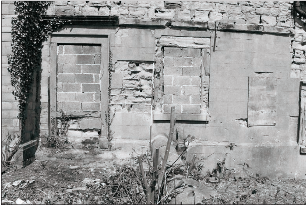
Plate 236: General view of the south elevation of Building 3, showing windows and former doorway (Film 01.23)
