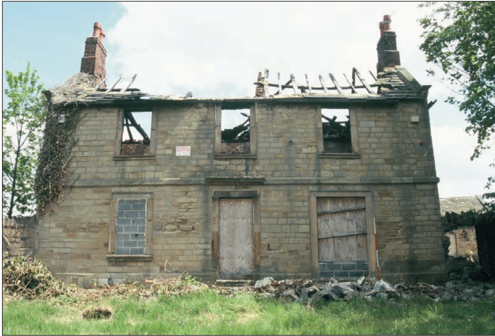
Plate 1: General view of the Georgian western facade of Hanson House (Building 4) (Colour Slide 04)
