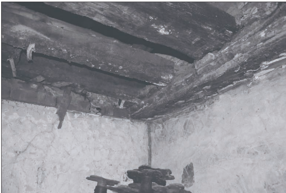
Plate 177: Detail of exposed timber beam at east end of G1, Building 2 (Film 42.25)
