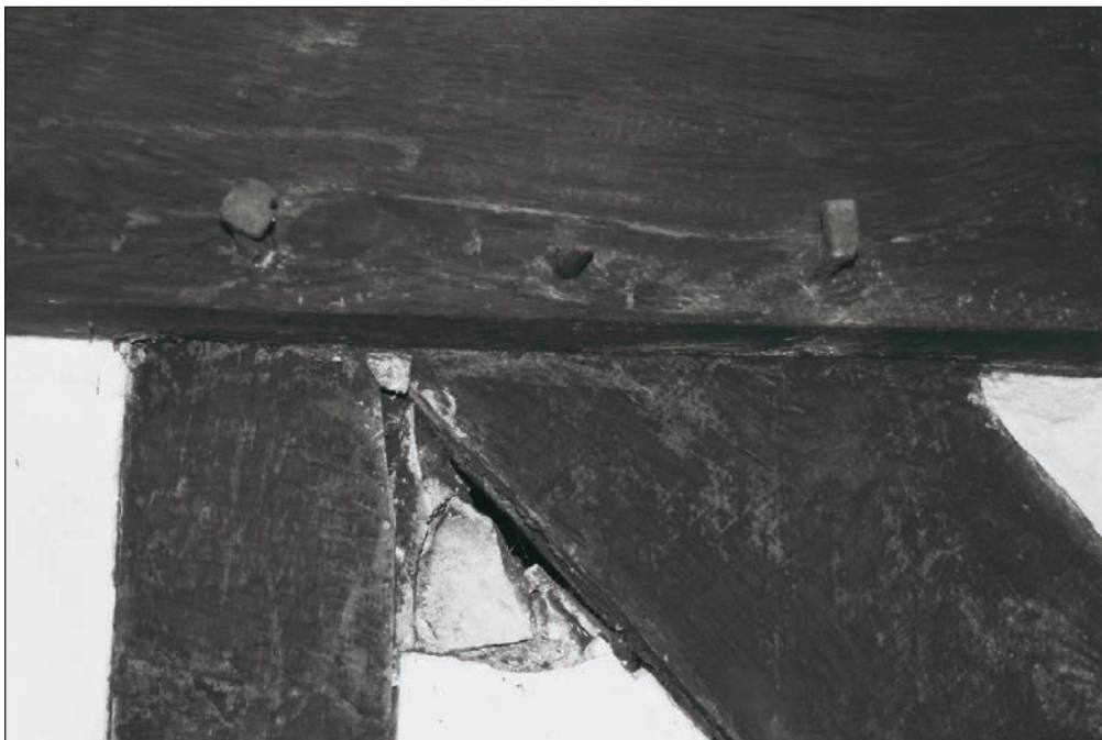
Plate 190: Detail of join between tie beam, arch brace and close stud, north end of timber partition, F1, Building 2 (Film 05.32)
