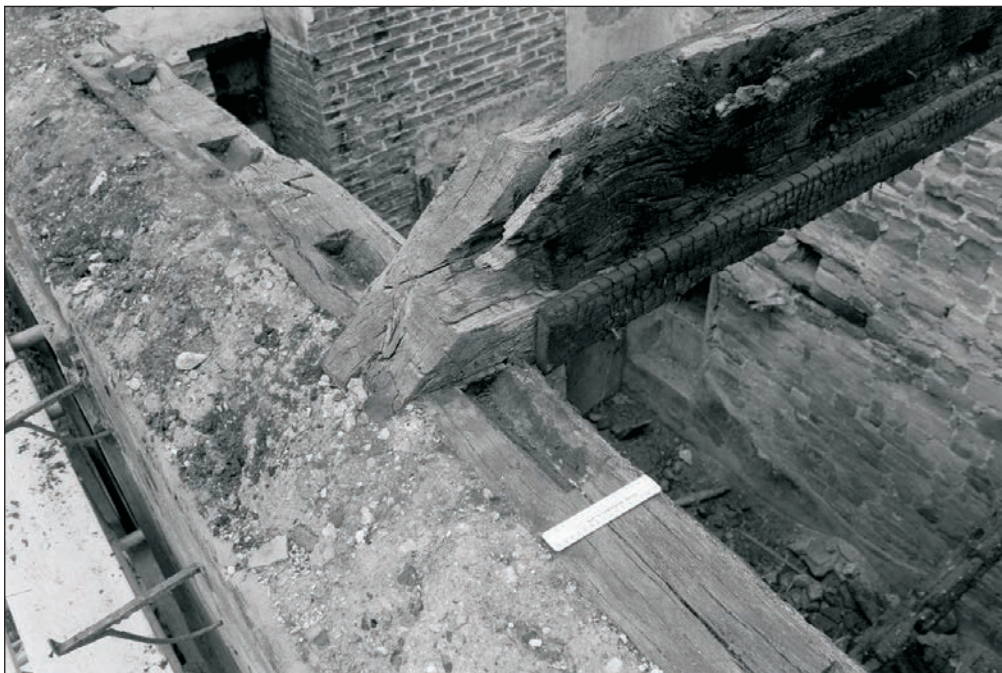
Plate 353: Detail of joint of tie beam and wall plate, west wall, Building 4 (Film 27.31)
