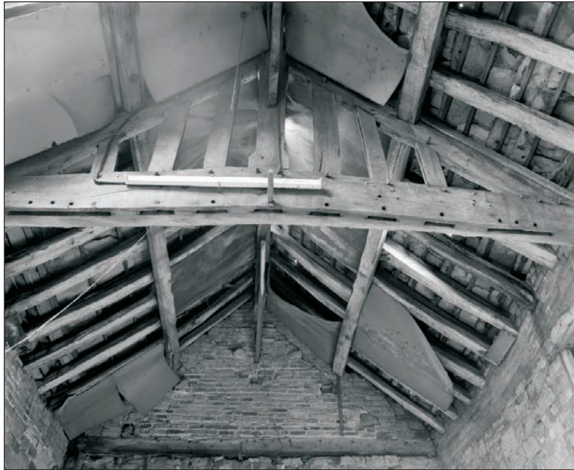
Plate 57: View of the timber truss, showing empty mortice joints on underside of tie beam, F1, Building 1 (Film 23.09)
