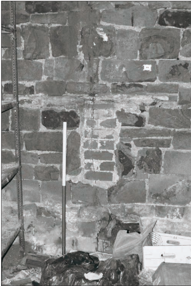
Plate 35: Detail of blocked breather slit, east wall of G1, Building 1 (Film 03.22)
