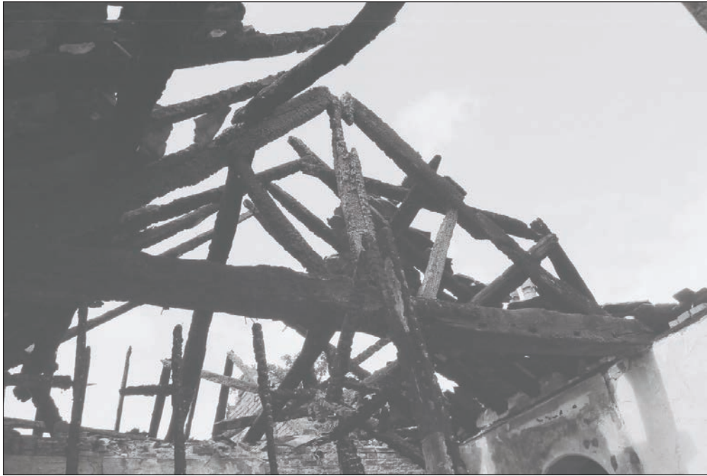
Plate 308: View of timber King-Post roof trusses of Building 3, from F3, Building 2 (Film 12.21)
