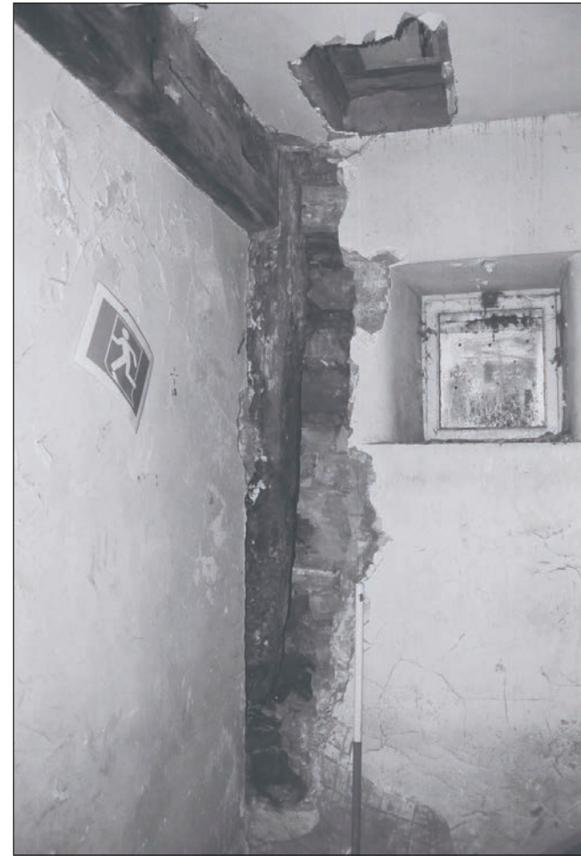
Plate 169: Detail of exposed north-west timber post of original framing, G3, Building 2 (Film 43.32)
