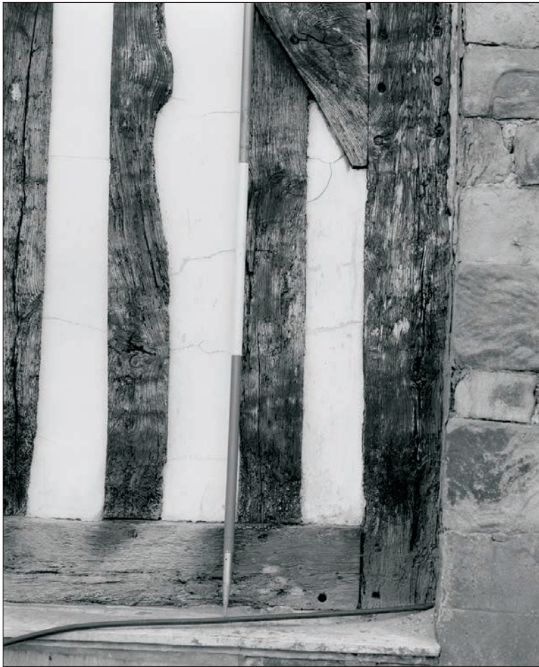
Plate 116: Detail of western post showing join with the mid-rail and arched brace, north elevation, Building 2 (note empty peg holes at bottom of post and mid-rail for former doorway, and those within post for a former arched brace to the west) (Film 09.05)
