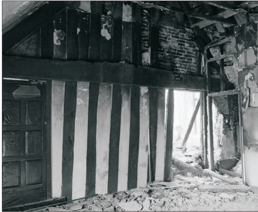
Plate 201: General view of F3, Building 2, showing close stud partition and inserted doorways to Building 3 (Film 15.05)
