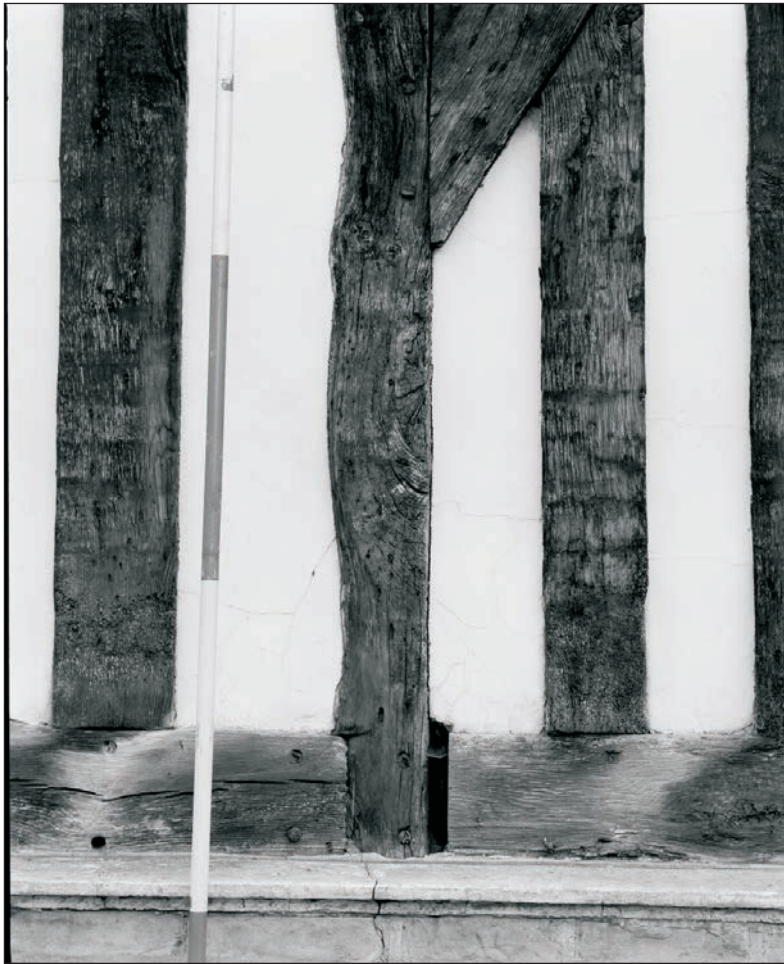
Plate 114: Detail of central post with arched brace and join with two phase mid-rail, north elevation, Building 2 (Film 09.08)
