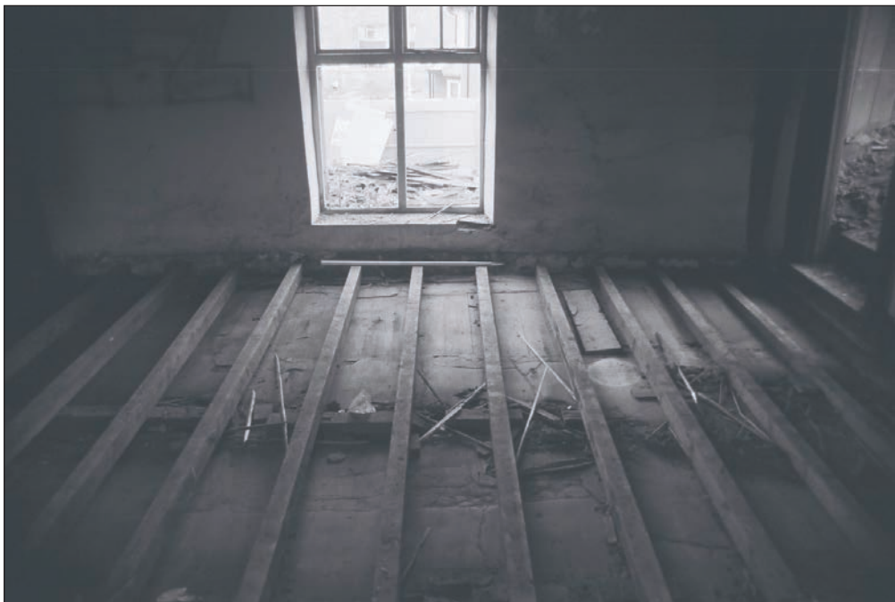
Plate 228: General view of lifted floor boards, F3, Building 2, showing limeash floor beneath and boarded area of original stair opening in floor (Film 40.03)
