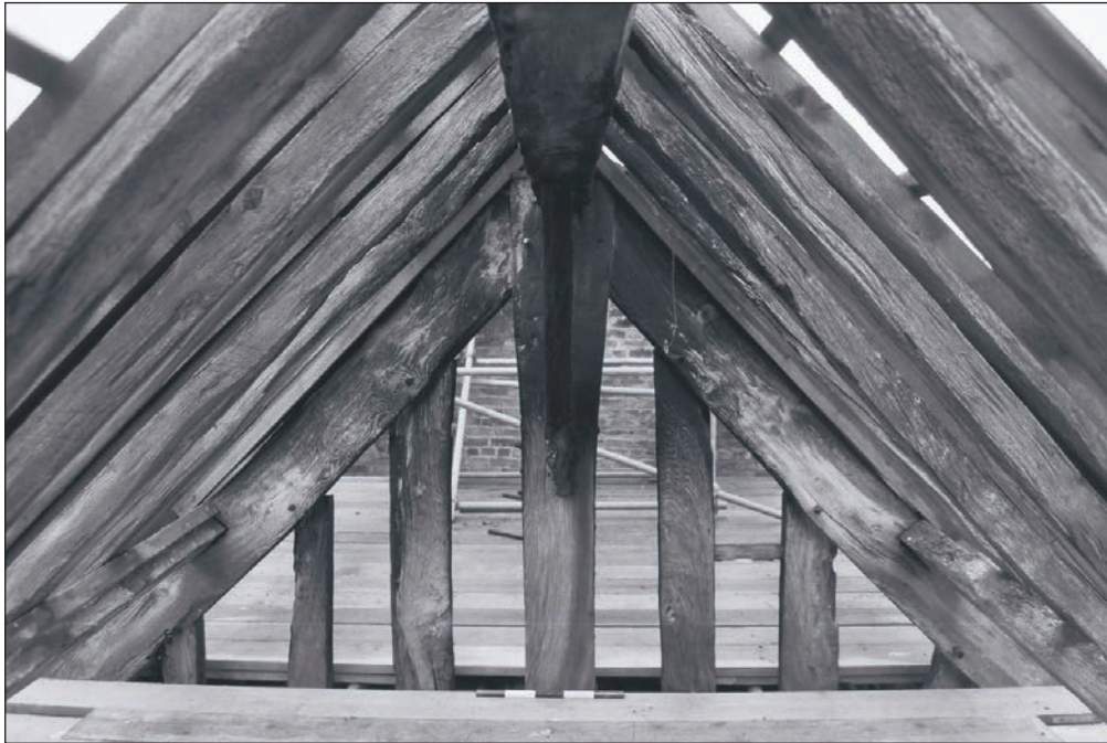
Plate 71: Detail of timber truss during the watching brief, showing the lower face, Building 1 (Film 39.23)
