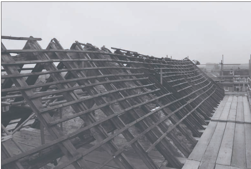
Plate 88: General view of the roof structure of Building 1 during the watching brief (Film 39.24)
