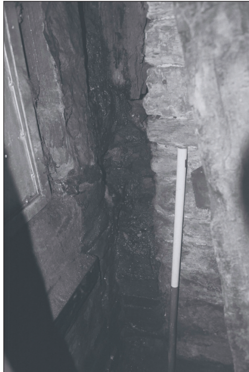
Plate 172: Detail of exposed south-west timber post, G4, Building 2, showing decayed base of timber and inserted brick plinth/pad (Film 42.10)
