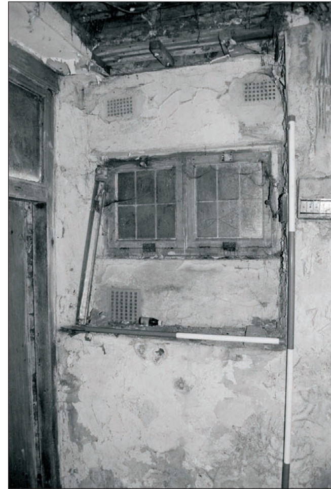
Plate 256b: Detail of window, north wall of cellar head G8, Building 3 (Film 28.16)
