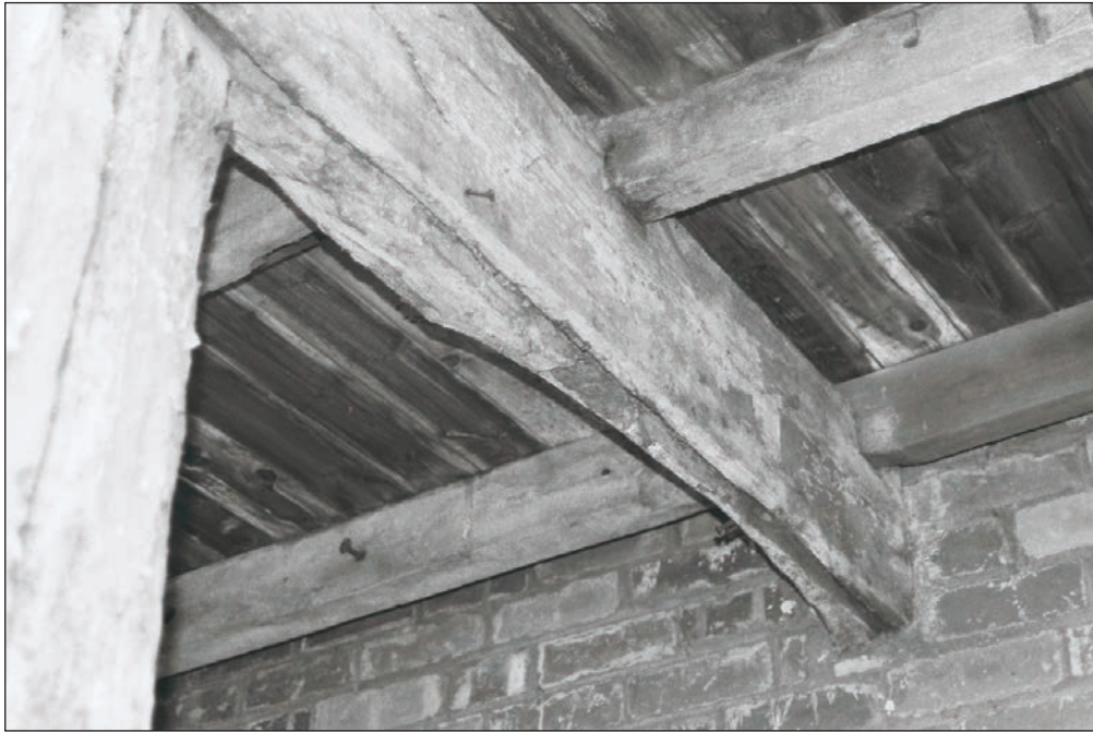
Plate 43: View of timber joists and beams of floor above G3, Building 1 (Film 03.27)
