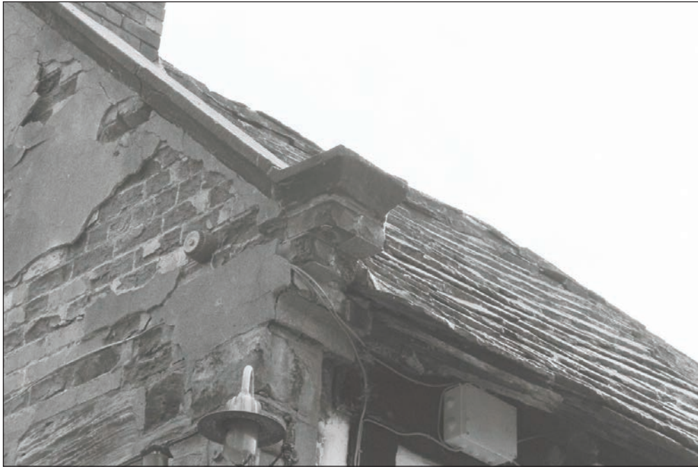
Plate 106: Detail of brick kneeler with stone coping, east gable and north elevation, Building 2 (Film 05.08)
