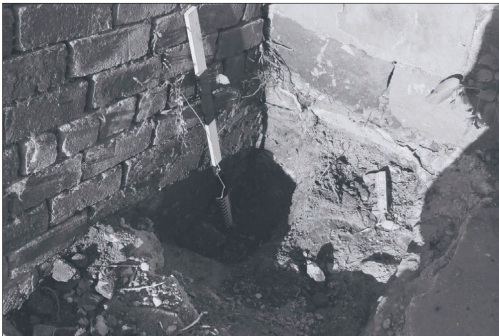
Plate 119: General view of Test Pit 8, against the south elevation of Building 2 (Film 35.23)
