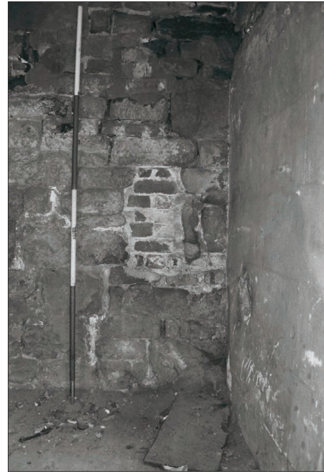
Plate 36: Detail of blocked breather slit, south wall of G1, Building 1 (Film 24.05)
