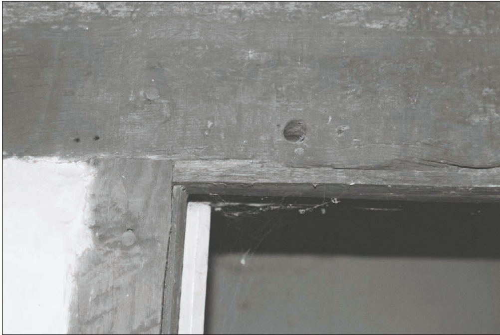
Plate 181: Detail of inserted doorway between F2 and F1 within close studding, Building 2 (Film 04.04)
