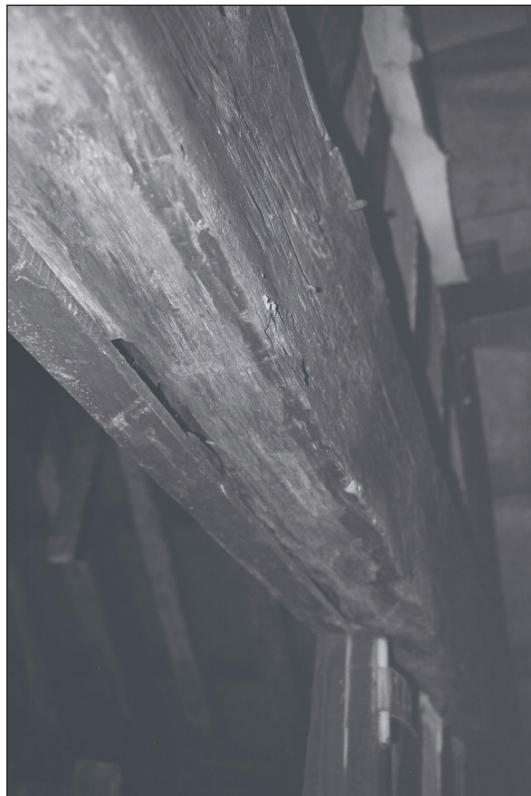
Plate 194: Detail of empty mortice holes in underside of tie beam of the central close stud partition, Building 2 (Film 43.10)
