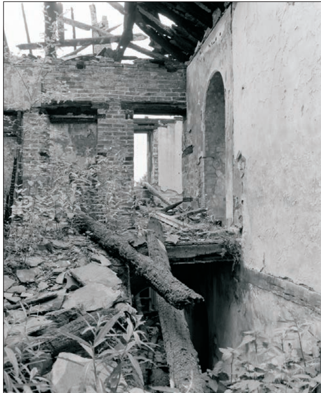
Plate 301: General view of rooms F5 and F7, Building 3, from F3, Building 2 (Film 16.03)
