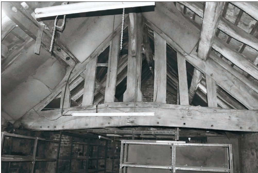
Plate 54: View of the timber truss, showing the fair or upper face, F1, Building 1 (Film 03.20)
