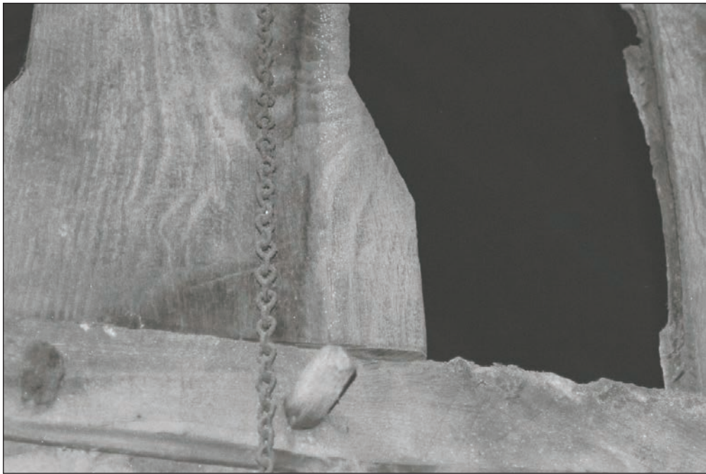
Plate 65: Detail of timber truss, F1, Building 1, showing the pegged King-Post and tie beam, and carpenters construction marks (Film 03.14)
