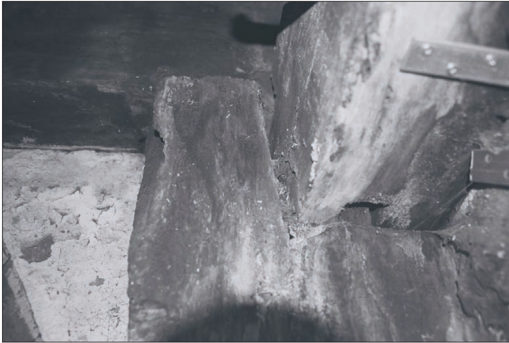
Plate 197: Detail of the central northern post joint with wall plate and tie beam, F1, Building 2 (Film 43.17)
