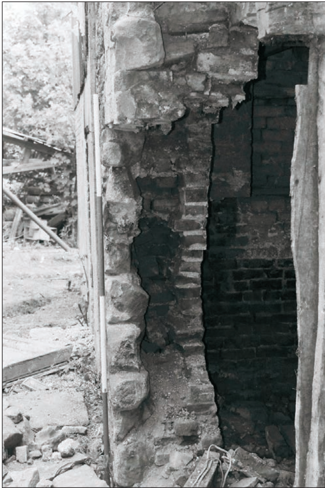
Plate 41: Detail of fabric of the north wall of G3, Building 1 showing inserted inner brick (Film 02.01)
