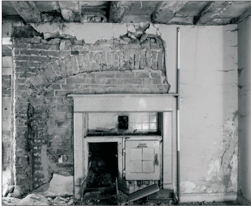
Plate 130: Detail of fireplace and exposed chimney breast during watching brief, G1, Building 2 (Film 31.01)
