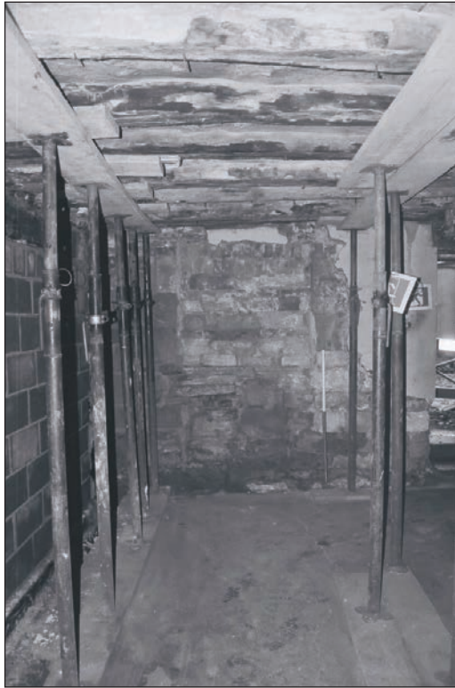
Plate 134: Detail of exposed blocked window within the north wall of G1, Building 2, during watching brief (Film 42.34)
