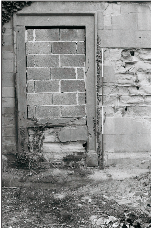
Plate 237: Detail of former doorway, altered to window, south elevation of Building 3 (Film 05.05)
