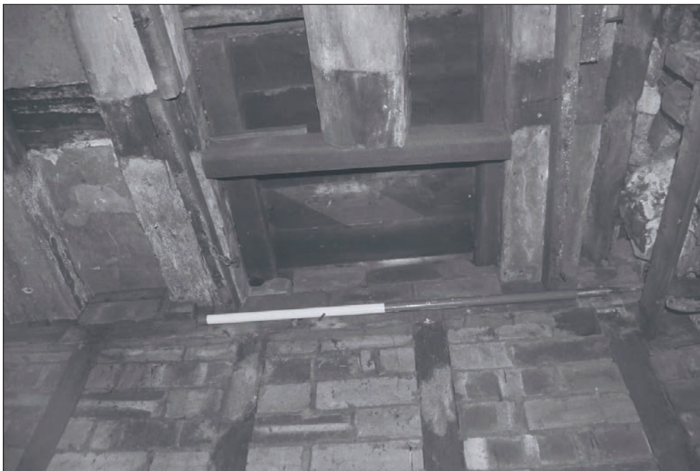
Plate 155: View of exposed former stair opening within the ceiling of G4, Building 2 (Film 30.20)
