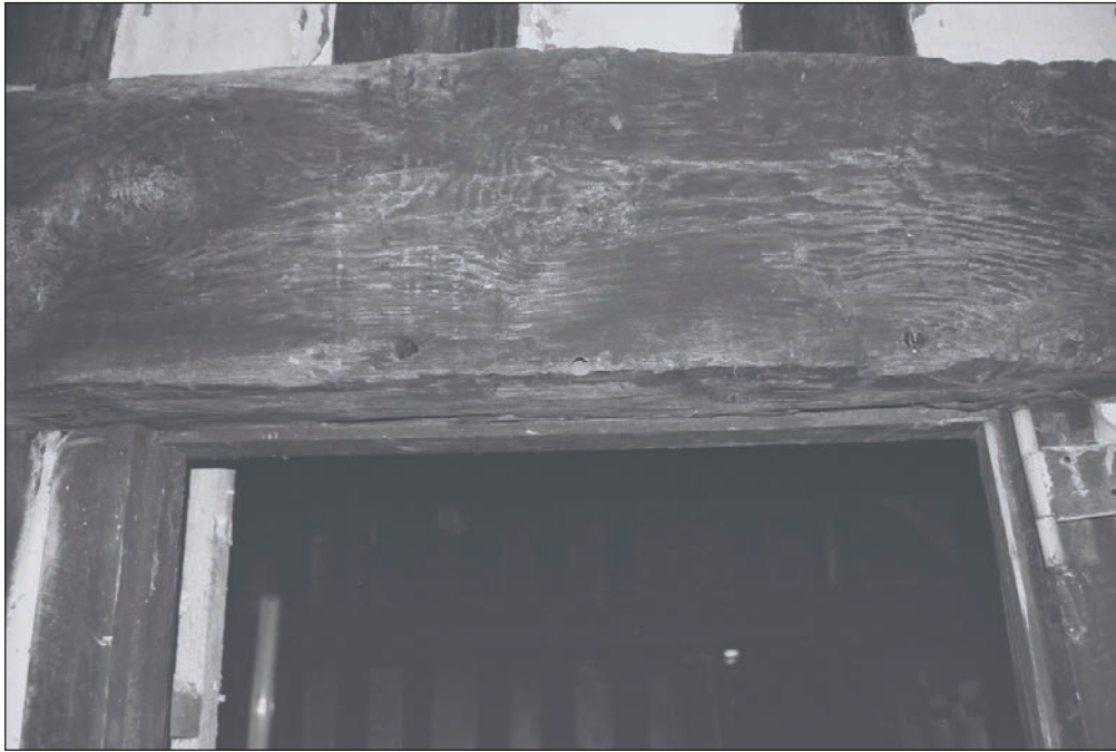
Plate 193: Detail of inserted doorway within the close stud partition between F1 and F2/3, showing empty peg and mortice holes, Building 2 (Film 43.12)
