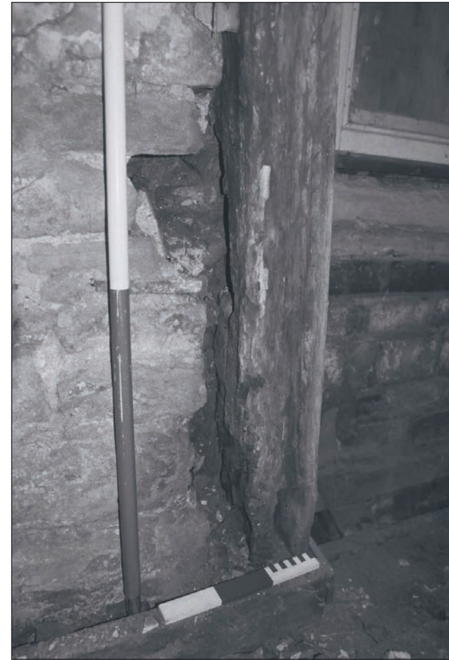
Plate 157: View of exposed original timber post, G4, Building 2 (Film 30.11)
