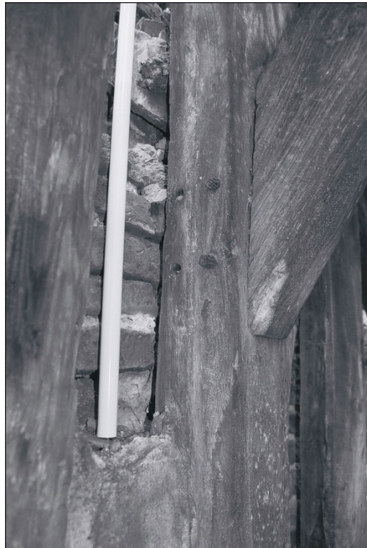
Plate 220: Detail of King-Post and ridge brace, showing empty peg holes to the west, F3, Building 2 (Film 41.13)
