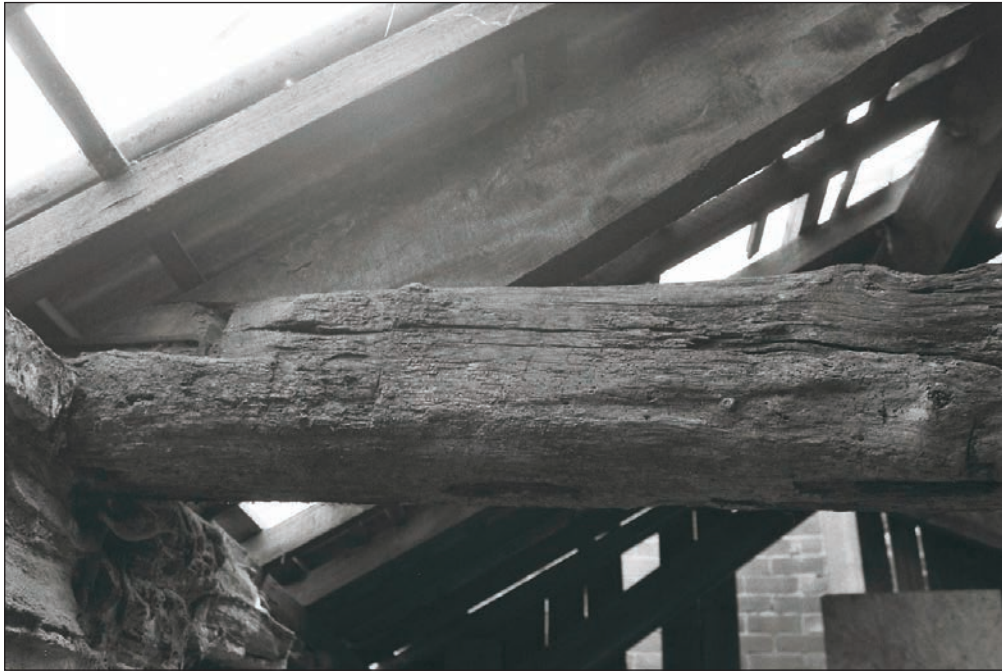
Plate 366: Detail of the joint between the tie beam and principal rafter with wall head, Building 5 (Film 02.22)
