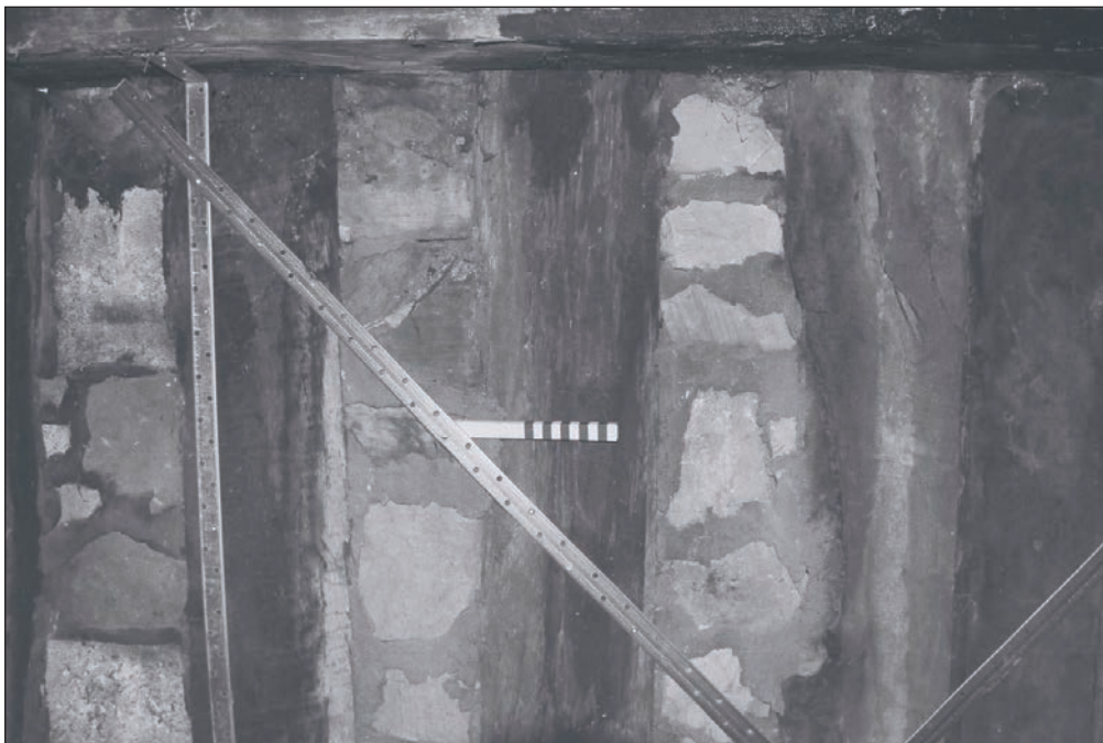
Plate 198: Detail of the original stone infills of the timber close studding of the first floor north wall, F1, Building 2 (Film 43.20)
