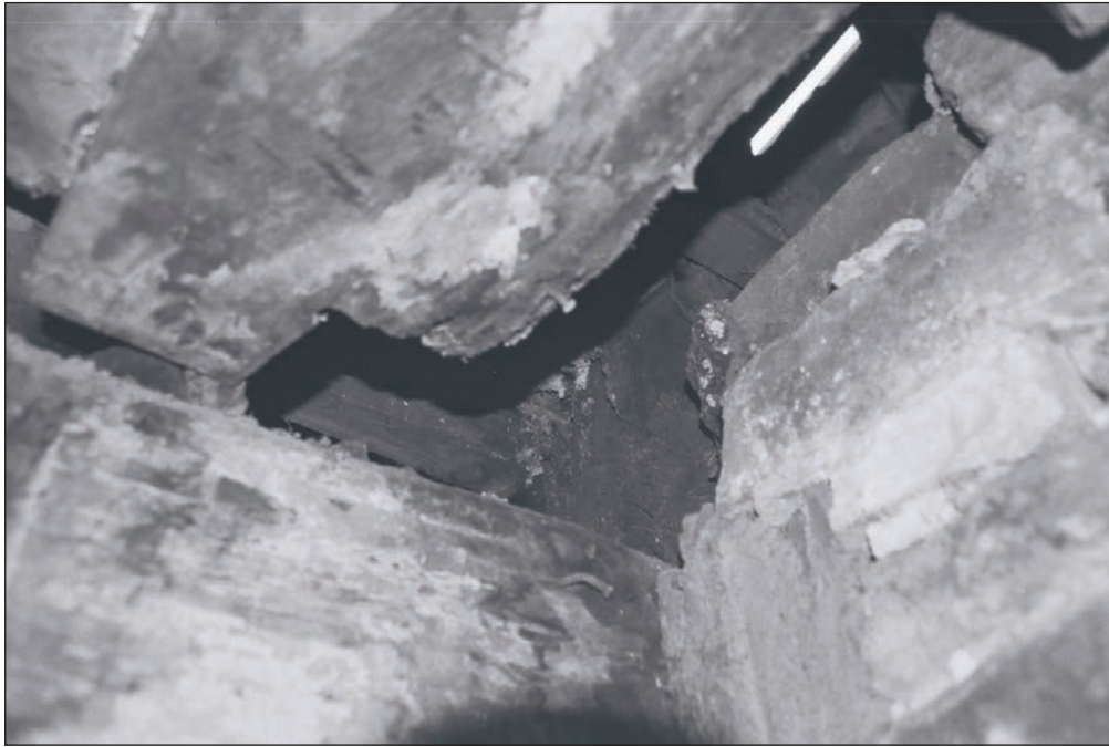
Plate 174: Detail of exposed timber framing above tie beam across G1 and join with the original north central timber post, G1, Building 2 (Film 42.32)
