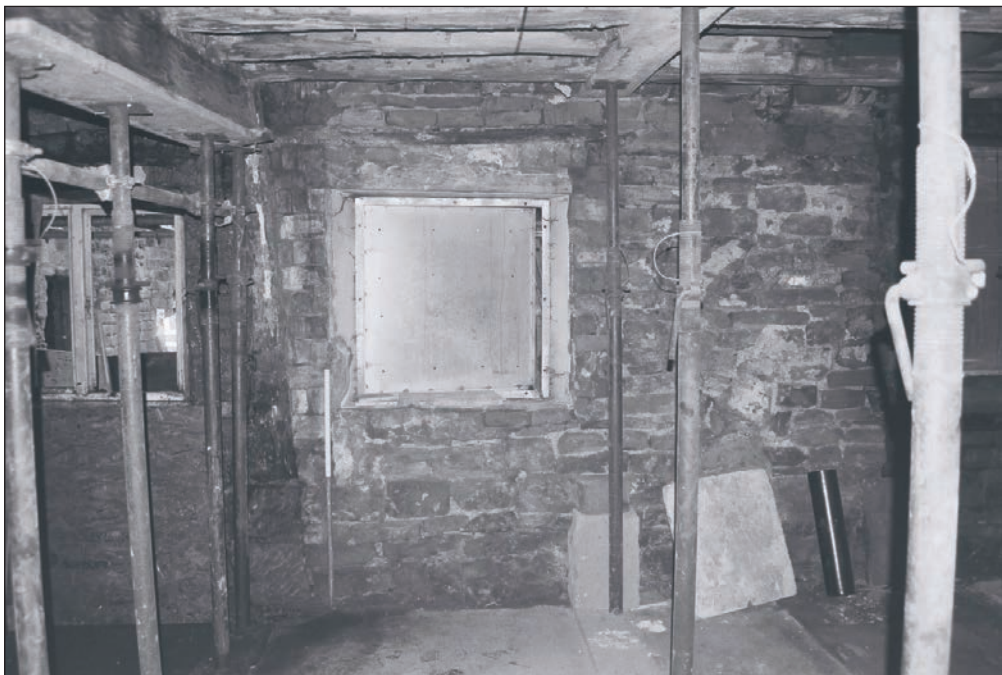
Plate 137: General view of exposed fabric of the south wall of G1 during watching brief (Film 42.21)
