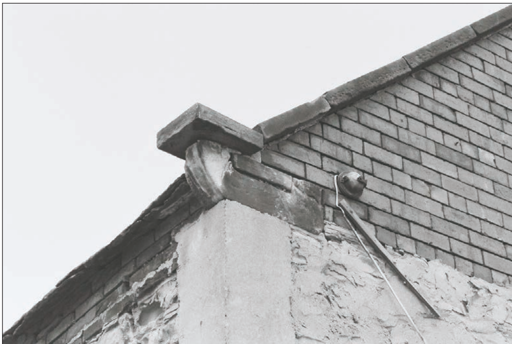
Plate 19: Detail of stone kneeler, south end of the west elevation of the barn, Building 1 (Film 02.08)
