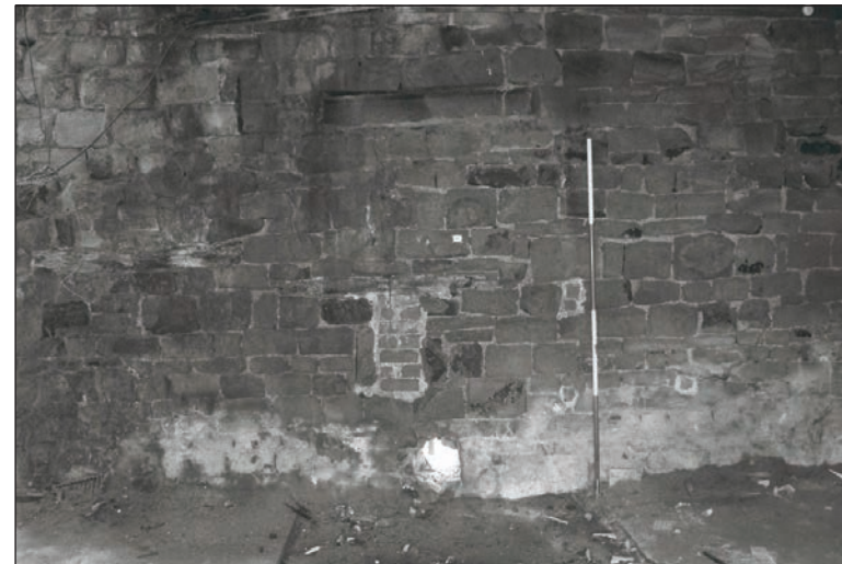
Plate 38: Detail of blocked breather slit, east wall of G1, Building 1 (Film 24.09)
