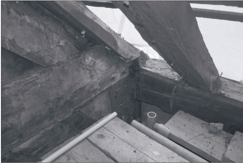
Plate 217: Detail of tie beam, wall plate, and post joint, northwest corner of F1, Building 2 (Film 41.18)
