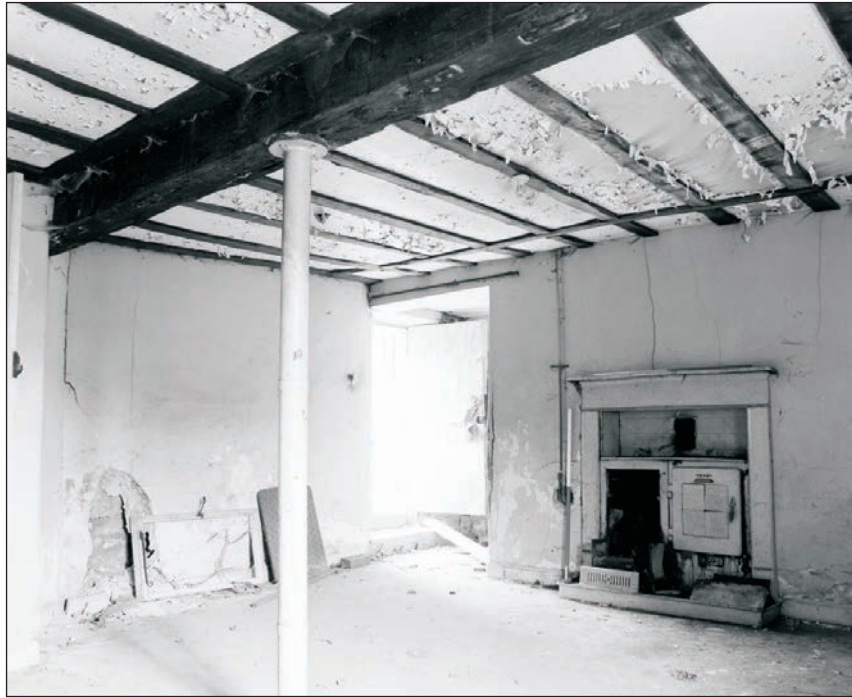
Plate 122: General view of G1, Building 2, showing cast iron column, fireplace and inserted doorway (Film 13.07)
