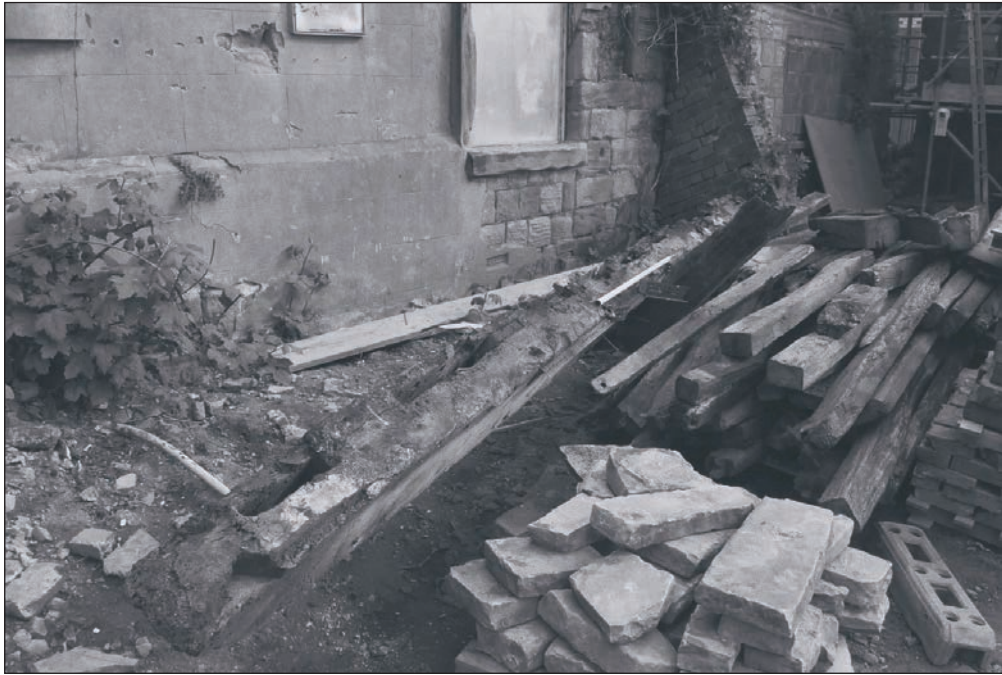
Plate 93: General view of removed tie beam from Building 1, during the watching brief (Film 39. 05)
