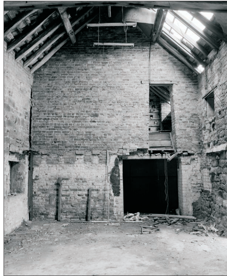
Plate 30: General internal view of G1 and F1, after the removal of modern shelving, Building 1 (Film 23.03)
