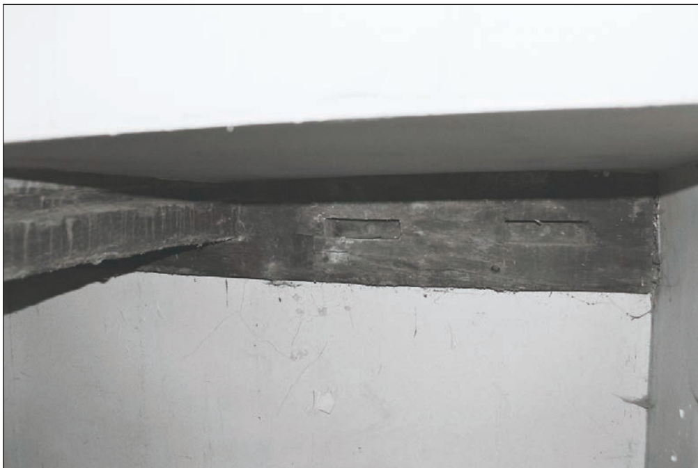
Plate 149: Detail of mortice holes from removed joists for the insertion of the staircase, G3, Building 2 (Film 06.05)
