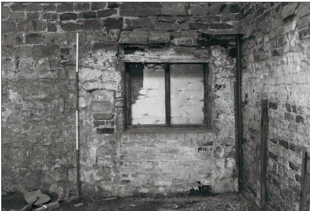
Plate 34: Internal detail of altered door to window and blocked breather slit, west wall of G1, Building 1 (Film 24.03)
