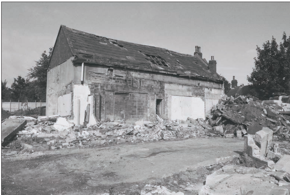
Plate 23: General view of the barn, Building 1 after the demolition of the modern extensions (Film 18.27)
