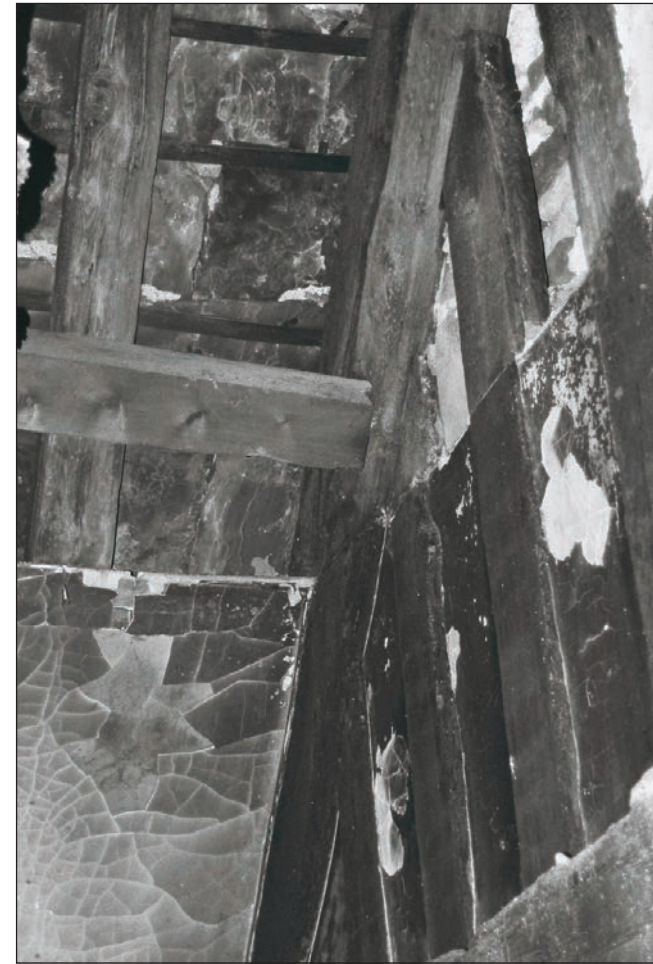
Plate 210: View of roof structure showing position of former ceiling, F3, Building 2 (Film 05.18)
