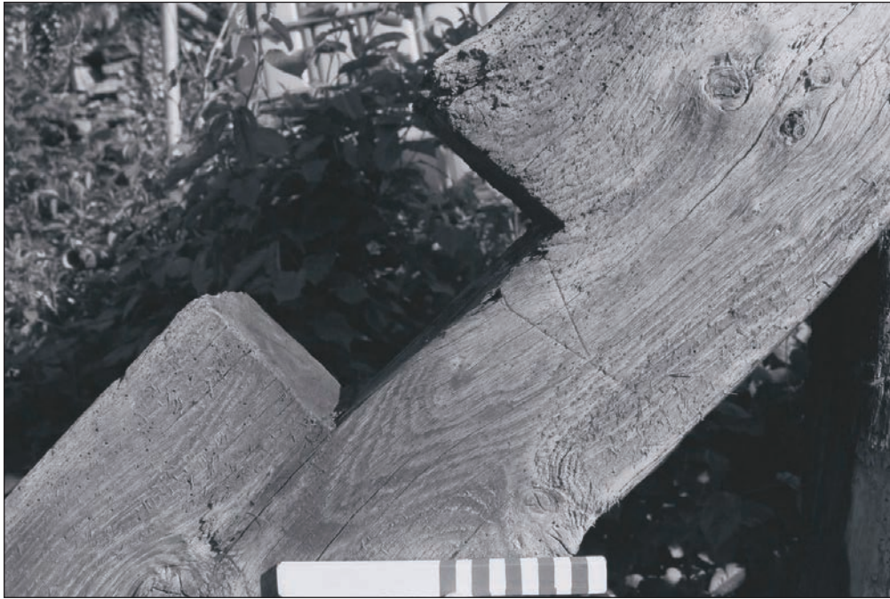
Plate 77: Detail of trench for purlin within the principal rafter of the truss removed from Building 1 during the watching brief (Film 39.10)
