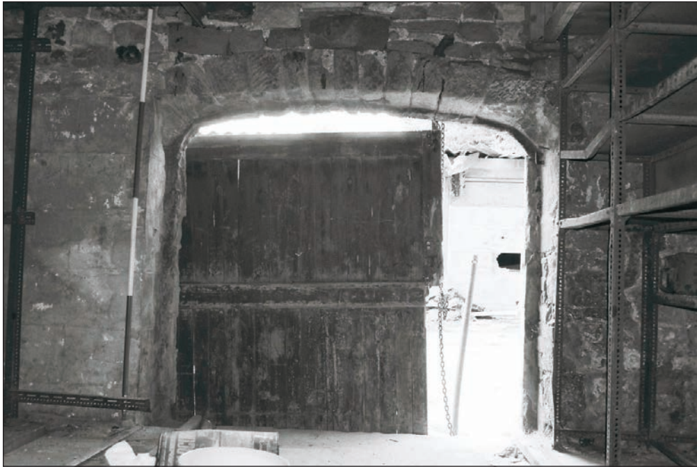
Plate 33: Internal view of the cart entrance, west wall of G1, Building 1 (Film 03.24)
