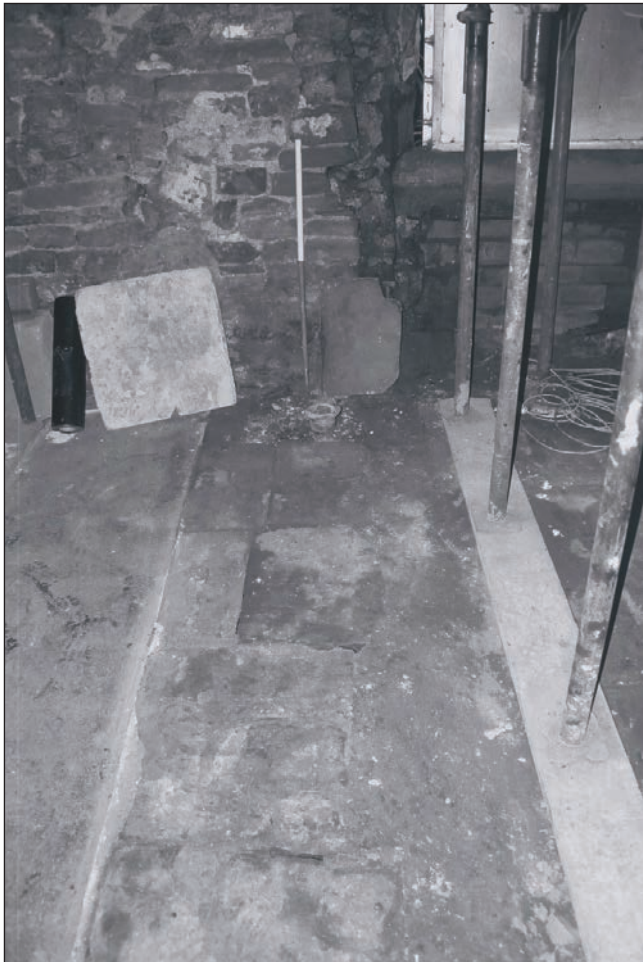
Plate 164: Detail of exposed stone flagged floor of former room G4/G1, showing the position of the primary timber partition since removed, watching brief, Building 2 (Film 42.13)
