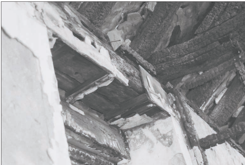
Plate 309: View of joint of window lintel, wall plate, tie beam and principal rafter above room F6, Building 3, from F3, Building 2 (Film 12.23)
