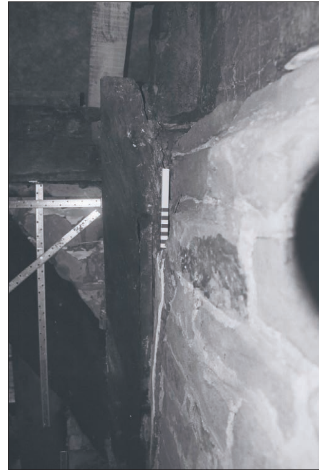
Plate 200: Detail of the northeast corner of F1 showing the exposed timber post with empty mortice hole, Building 2 (Film 43.24)
