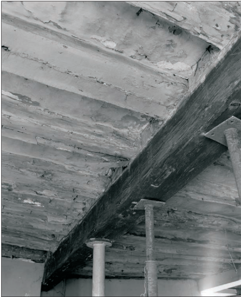
Plate 142: View of the exposed ceiling and join of joists with beam, G1, Building 2 (Film 31.05)
