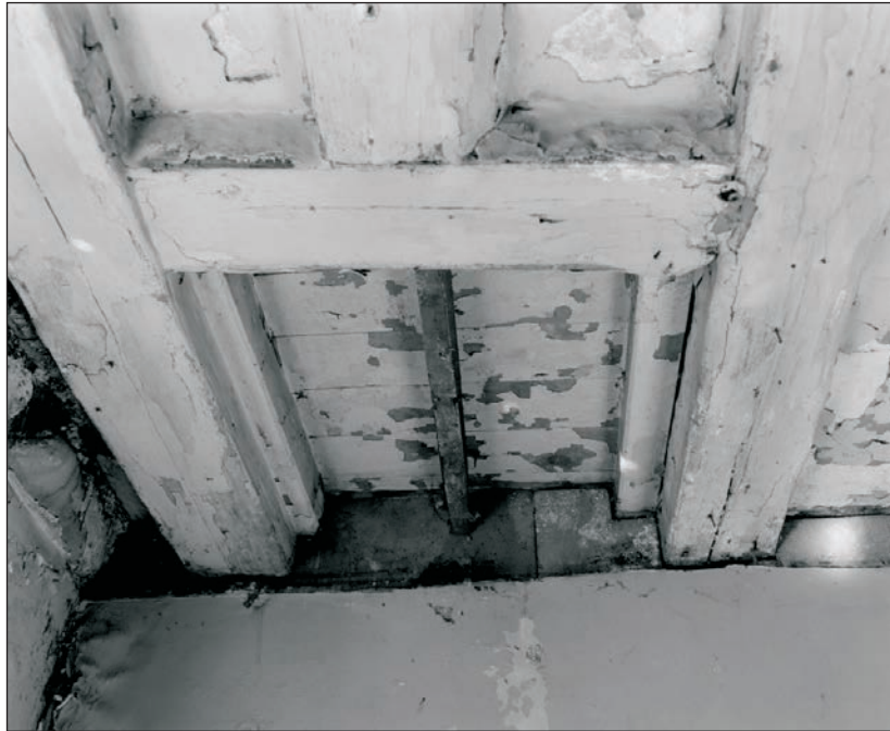
Plate 146: Detail of exposed former stair opening within the ceiling of G1, Building 2 (Film 31.03)
