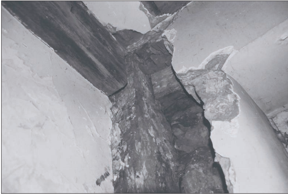
Plate 170: Detail of the exposed north-west post showing the joints with the mid-rail and tie beam, G3, Building 2 (Film 43.30)
