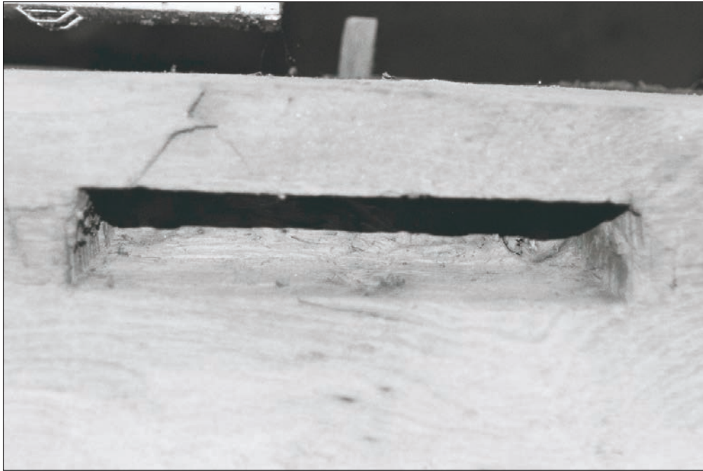
Plate 69: Detail of an empty mortise within the timber truss, F1, Building 1 (Film 06.13)
