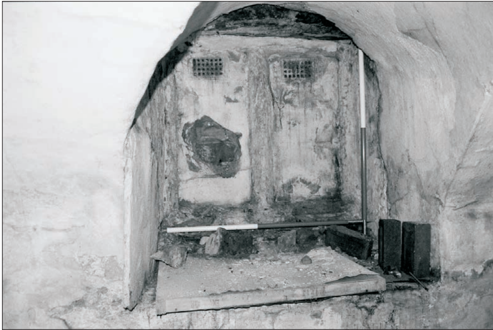
Plate 262: Detail of blocked window in west wall of room C2, Building 4 (Film 28.33)
