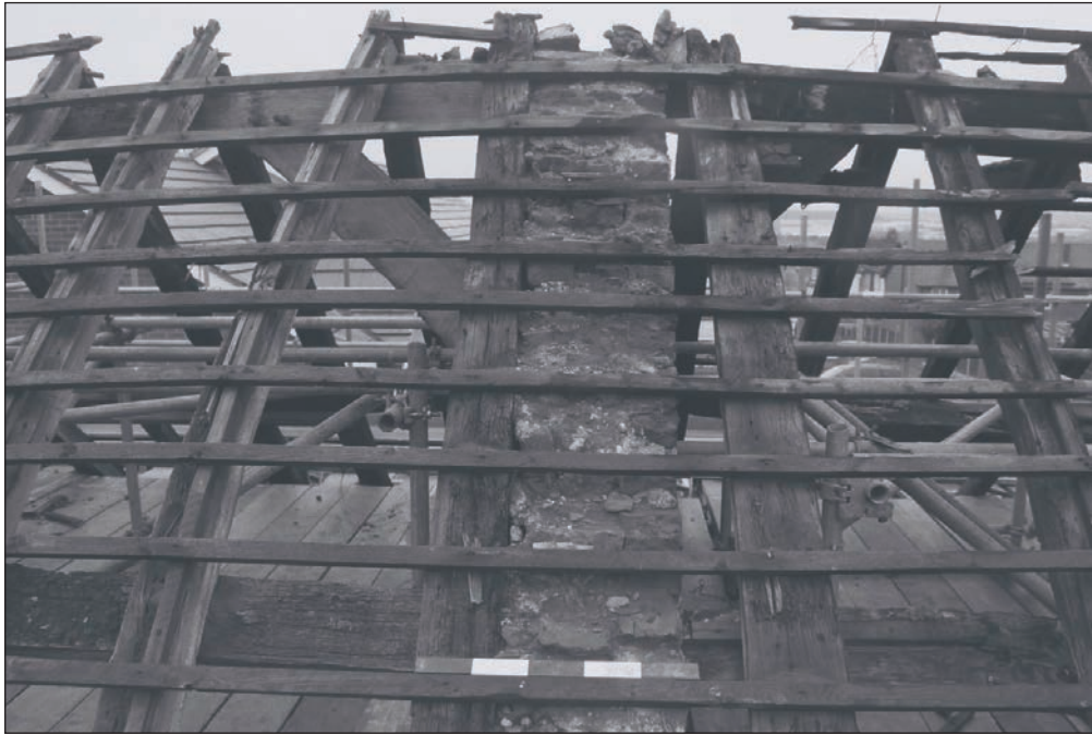
Plate 89: View of the inserted brick infill of the truss and south wall of the dovecote during the watching brief, Building 1 (Film 39.25)
