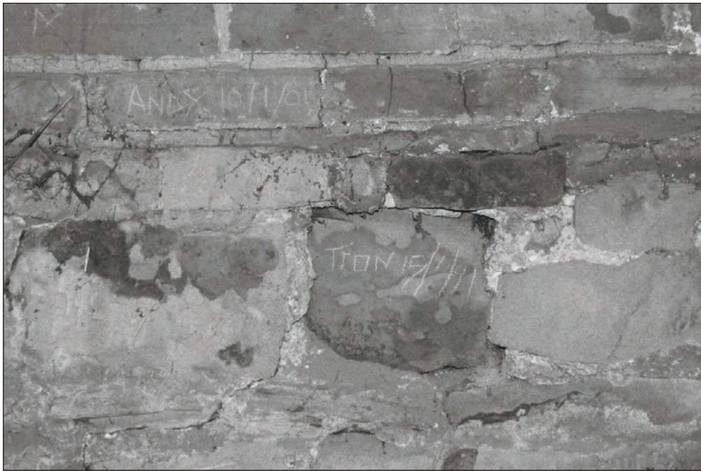
Plate 49: Detail of graffiti, west wall of F1, Building 1 (Film 06.16)
