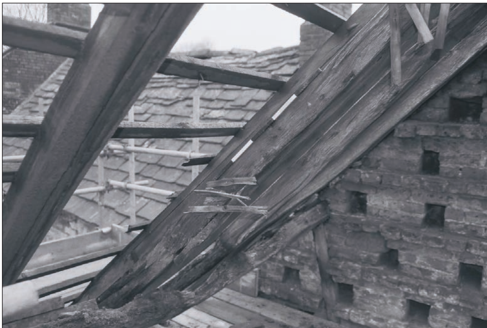
Plate 90: Detail of the common rafters of Building 1 during the watching brief (Film 39.30)
