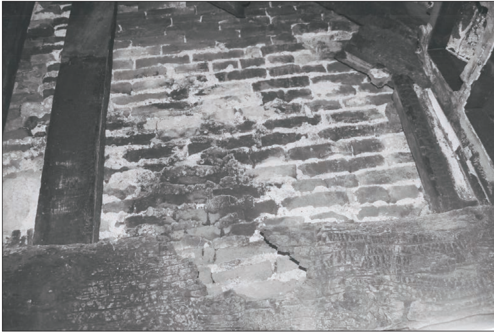
Plate 205: Detail of damaged timber partition/roof and brick gable of Building 3 built abut, west wall of F3, Building 2 (Film 12.01)
