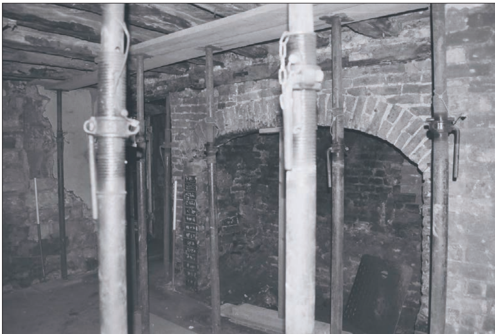
Plate 131: Detail of exposed fireplace and chimney breast during watching brief, G1, Building 2 (Film 42.35)
