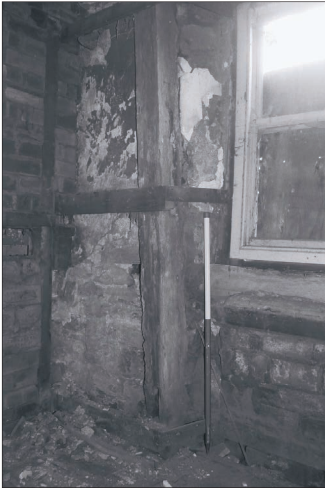
Plate 156: View of exposed original timber post, G4, Building 2 (Film 30.15)
