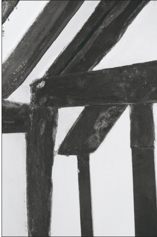
Plate 189: Detail of truncated arch brace, south end of timber partition, F1, Building 2 (Film 05.34)
