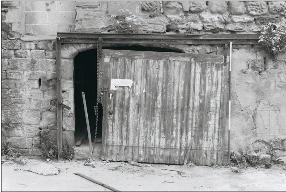
Plate 12: Detail of the cart opening, west elevation of the barn, Building 1 (Film 02.18)
