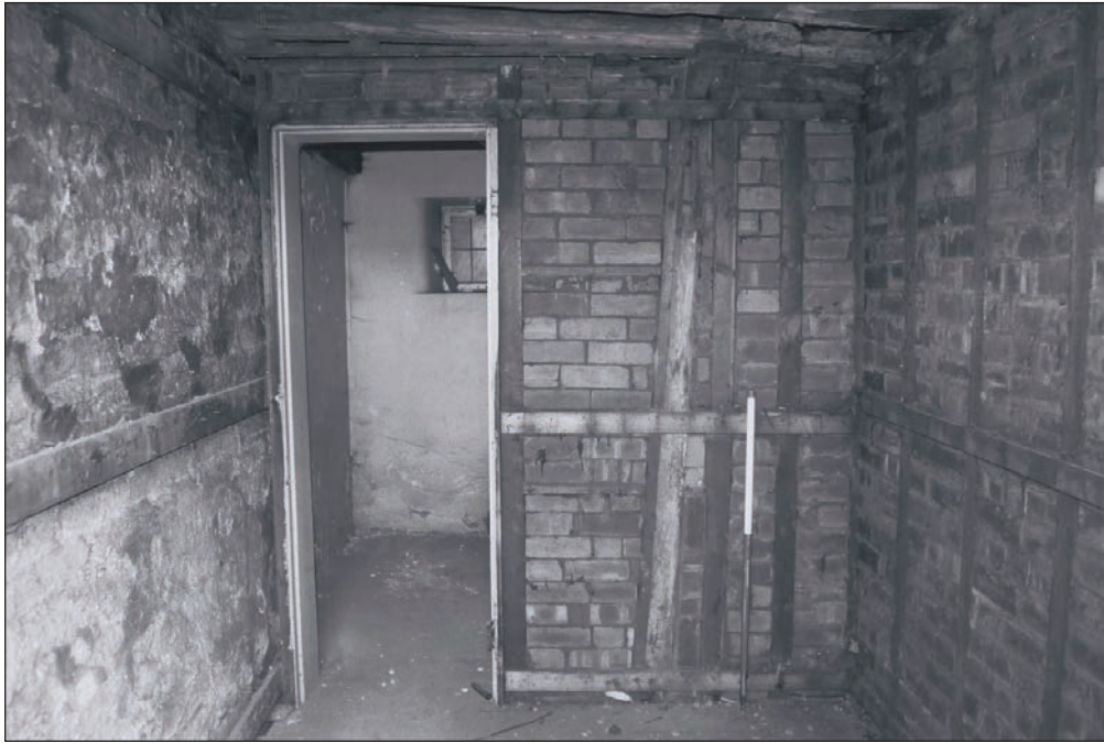
Plate 160: View of G4 after soft strip exposing original timber post to the north, Building 2 (Film 30.24)
