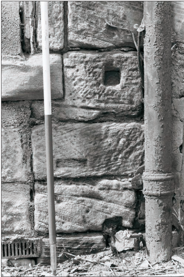
Plate 100: Detail of vertical joint of former doorway, south elevation of Building 2 (Film 05.07)
