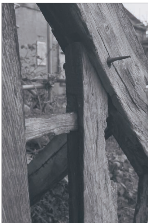
Plate 75: Detail of former lath infill of the timber truss from Building 1, during the watching brief (Film 39.06)
