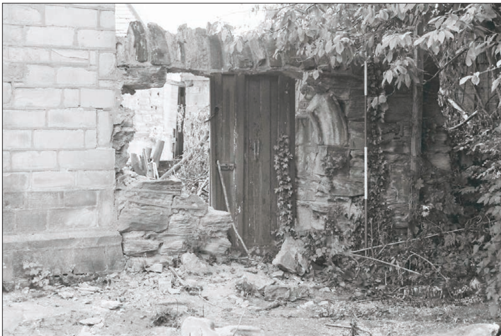
Plate 243: General view of garden wall attached to the south of the west elevation of Building 4 (Film 01.19)
