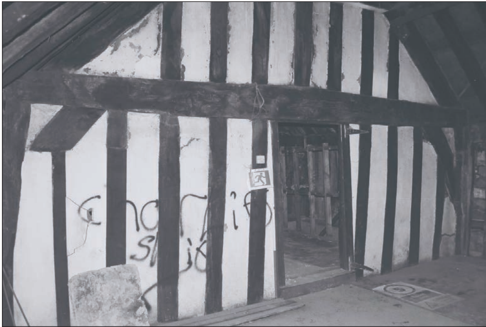
Plate 192: General view of F1 during the watching brief showing the central close stud partition, Building 2 (Film 43.14)
