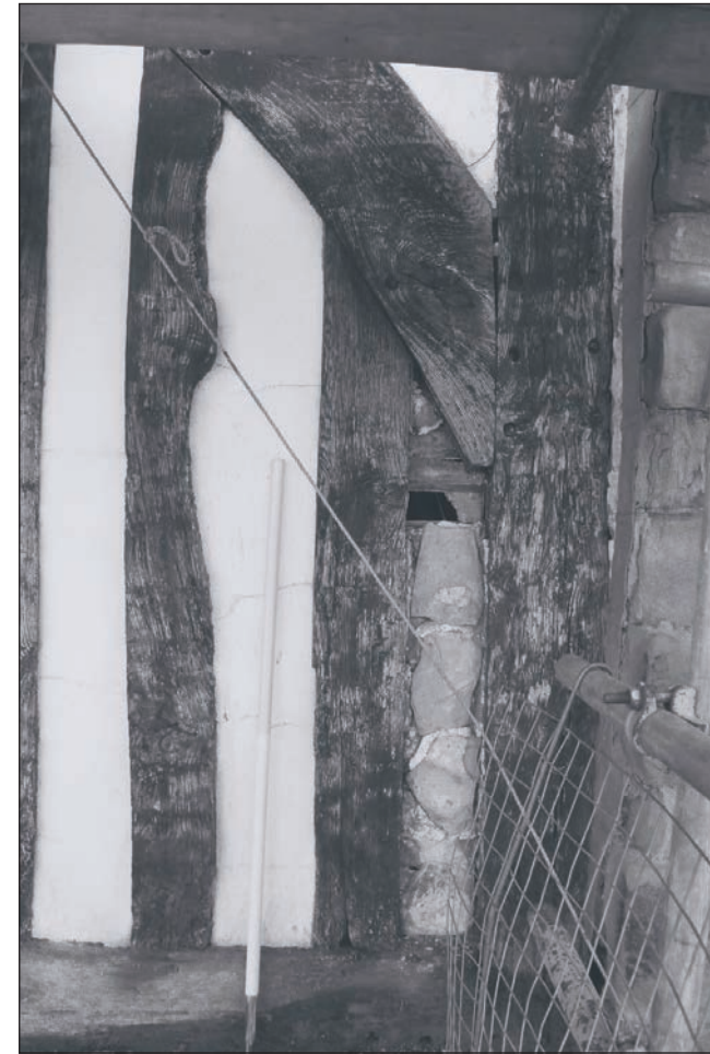
Plate 117: Detail of western post and arched brace, showing original stone infill, north elevation, Building 2 (Film 41.23)
