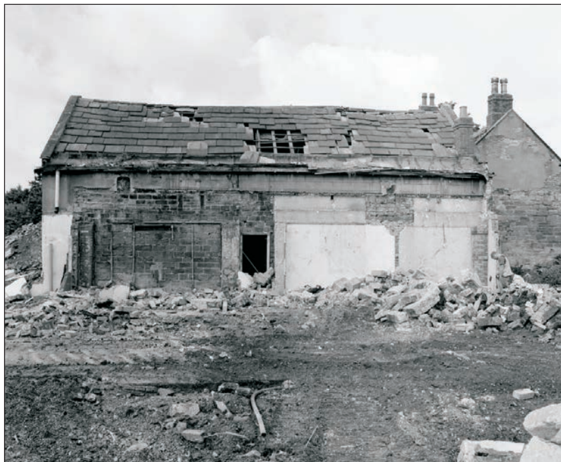
Plate 25: General view of the east elevation of the barn, Building 1 after the demolition of the modern extensions (Film 20.05)
