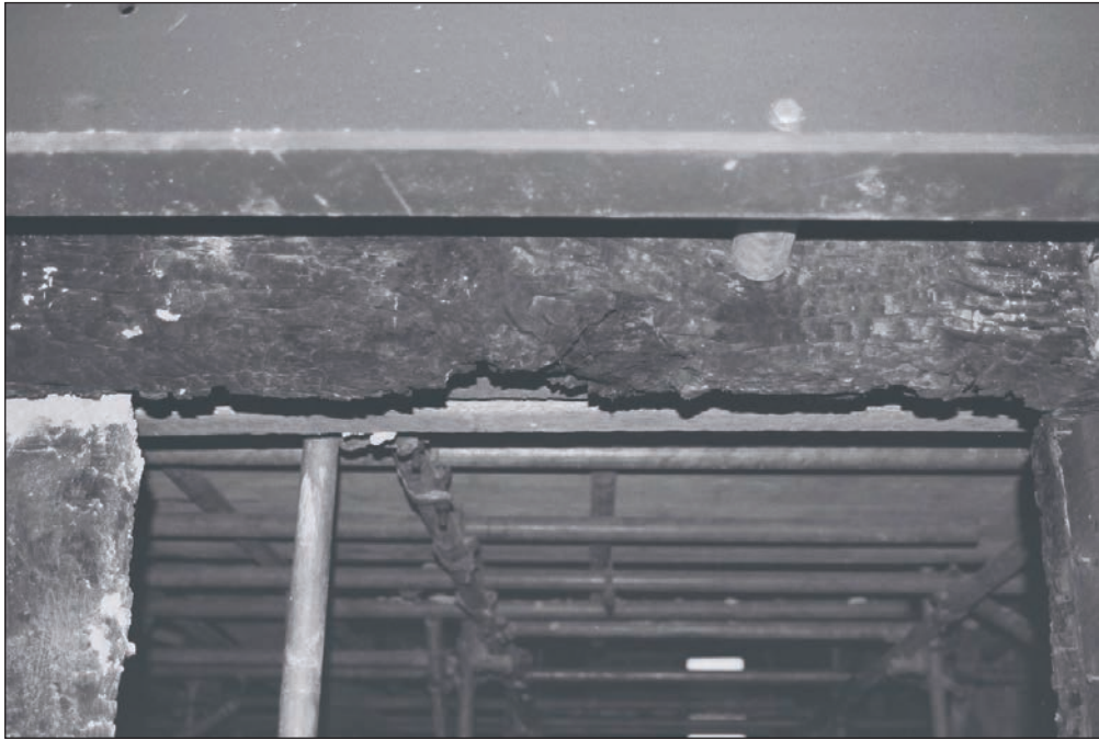
Plate 207: Detail of damaged empty peg holes within inserted doorway of close stud partition, F3, Building 2 (Film 43.05)
