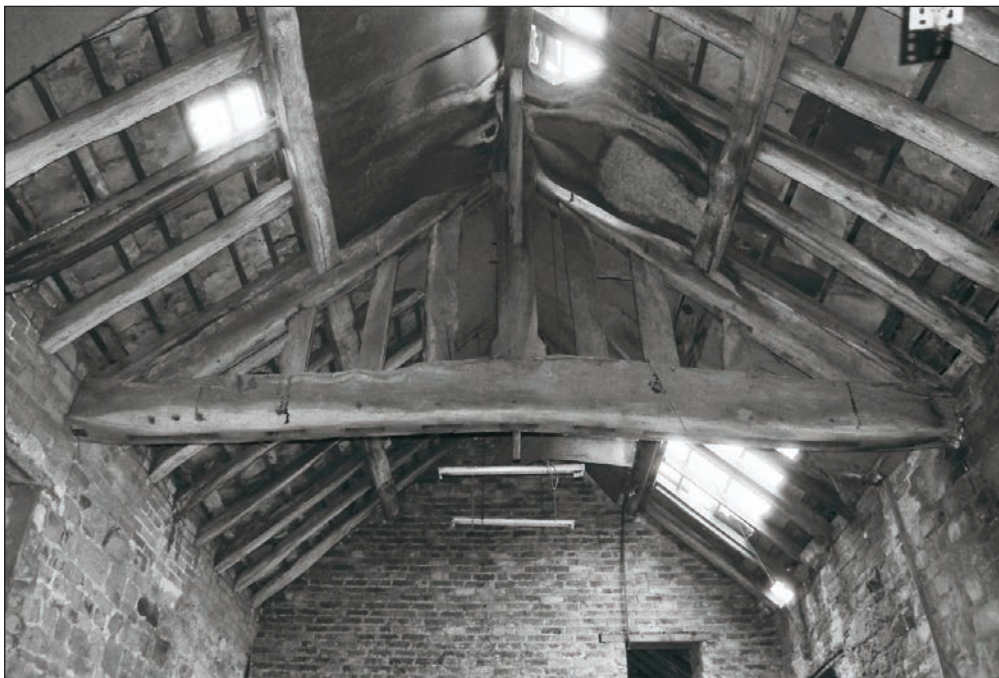
Plate 58: View of the timber truss, showing empty mortice joints on underside of tie beam, F1, Building 1 (Film 24.19)
