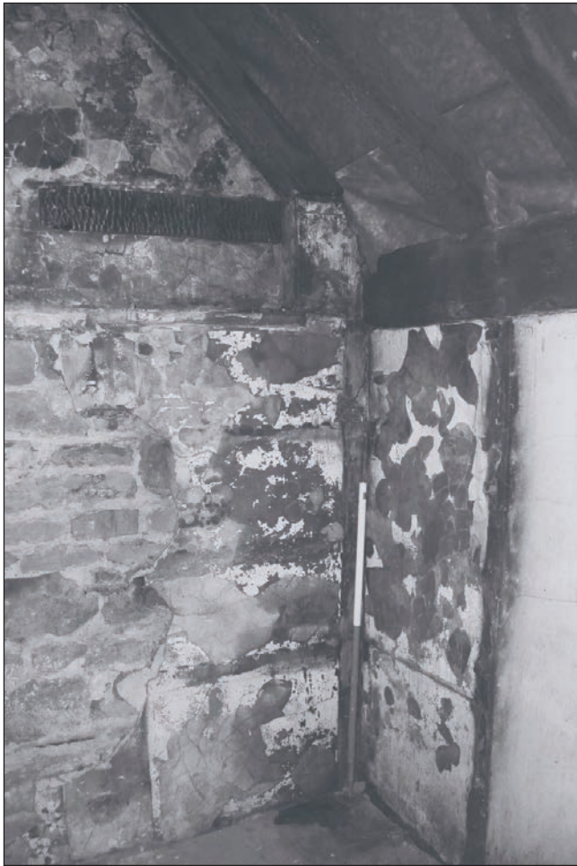
Plate 195: Detail of the southeast corner of room F1, Building 2, showing removed timber post and truncated tie beam and rafter (Film 43.08)
