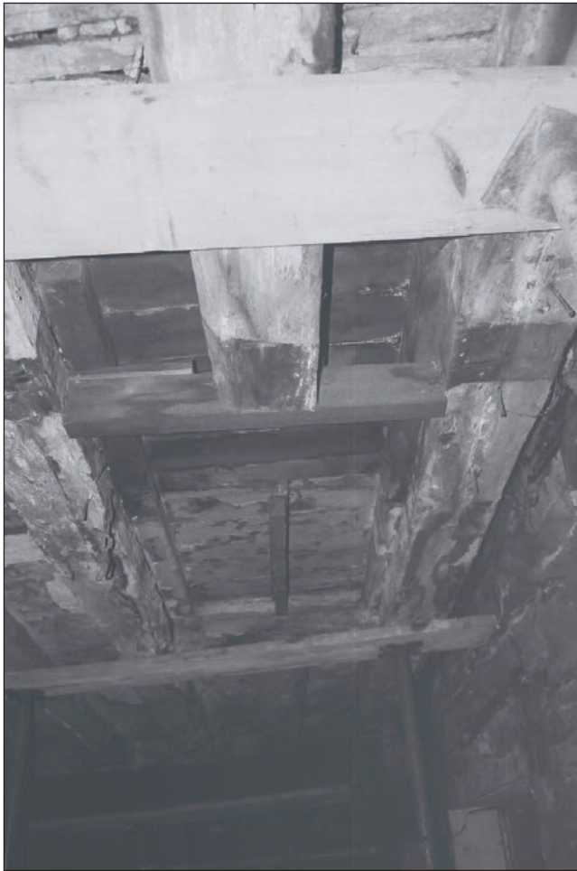
Plate 168: Detail of fully exposed former staircase opening in the ceiling of G1 and G4, Building 2 (Film 43.34)
