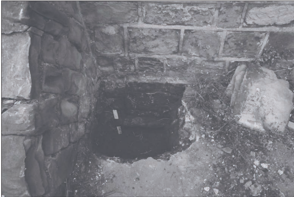
Plate 118: General view of Test Pit 3 against the north elevation of Building 2 (Film 36.06)
