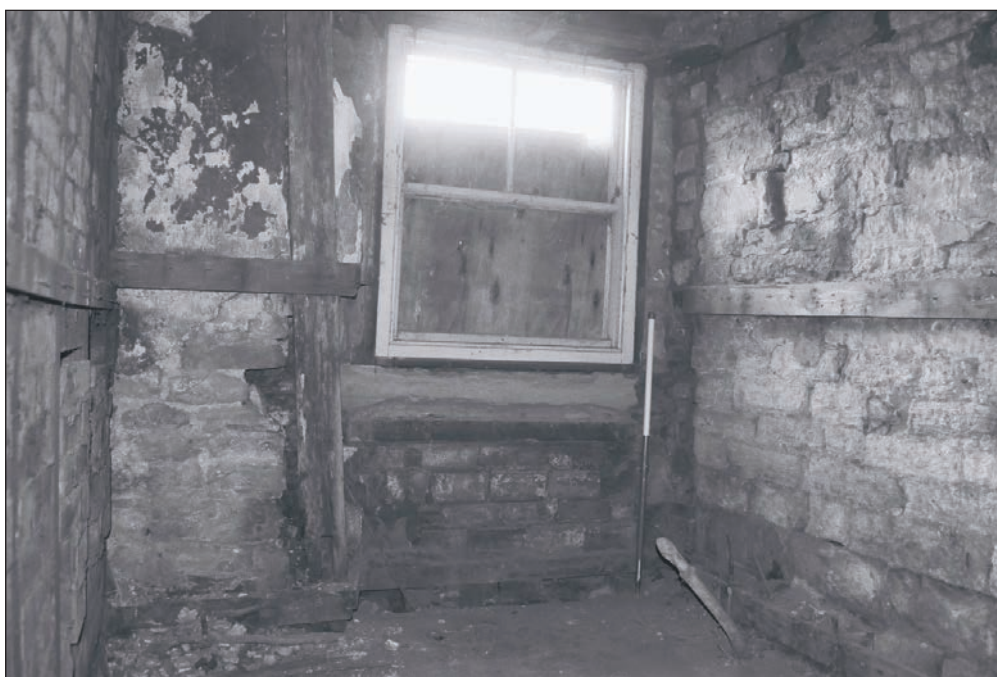
Plate 153: General view of G4 after soft strip during watching brief, Building 2, showing altered door to window, and adjacent timber framing (Film 30.16)
