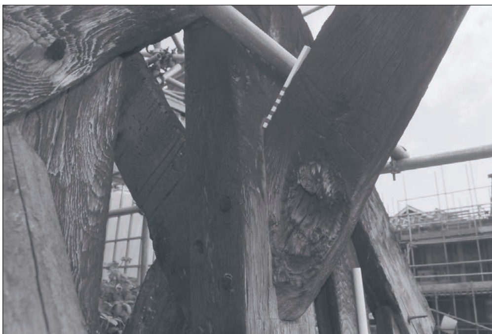
Plate 76: Detail of timber ridge braces and King-Post, removed truss from Building 1 (Film 39.08)
