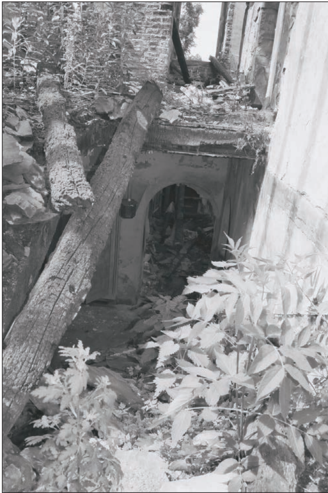
Plate 302: View down staircase from F7 to G6, Building 3, from F3 Building 2 (Film 12.09)
