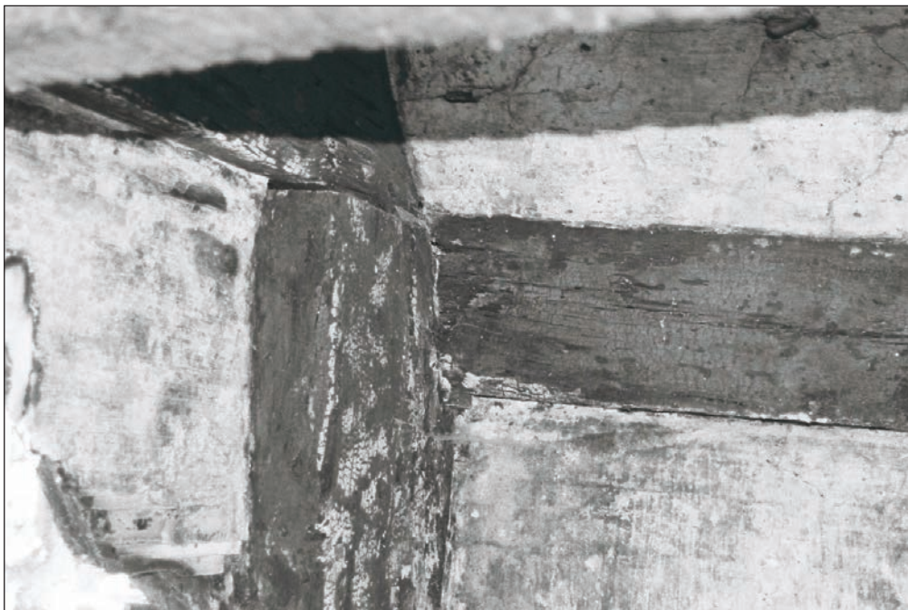
Plate 206: Detail of joint of tie beam, post and wall plate, northwest corner of F3, Building 2 (Film 05.21)
