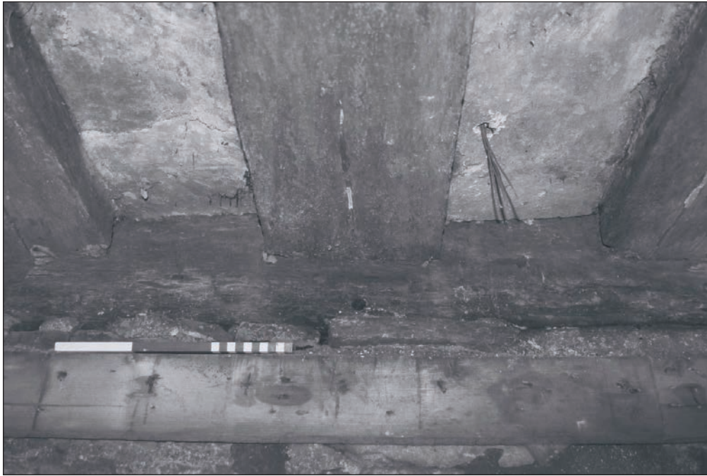
Plate 154: Detail of exposed ceiling and joists, with timber beam within west wall of G4, Building 2 (Film 30.07)
