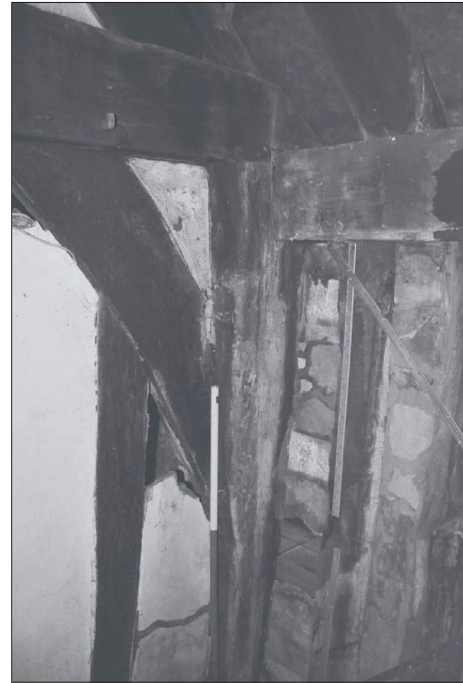
Plate 196: Detail of the central northern timber post and joints with the close stud central partition, F1, Building 2 (Film 43.16)
