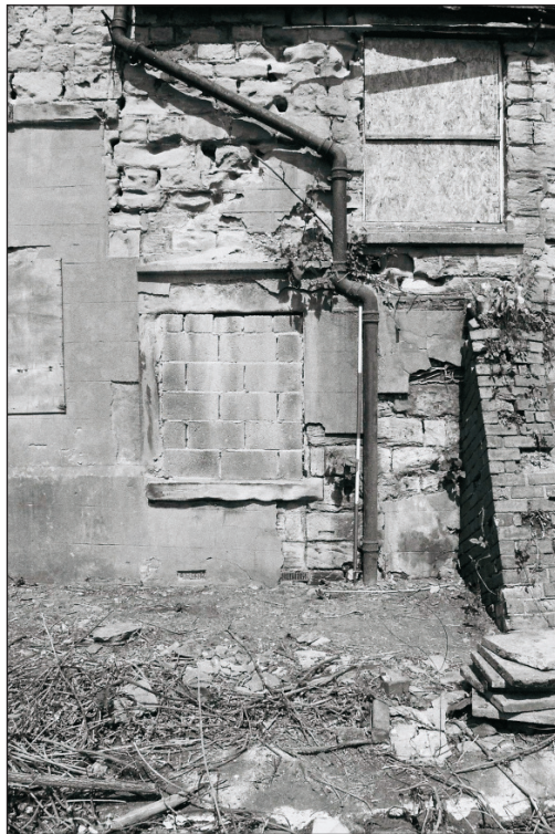
Plate 99: View of the west end of the south elevation of Building 2, showing the former doorway, and vertical joint with Building 3 (Film 01.24)
