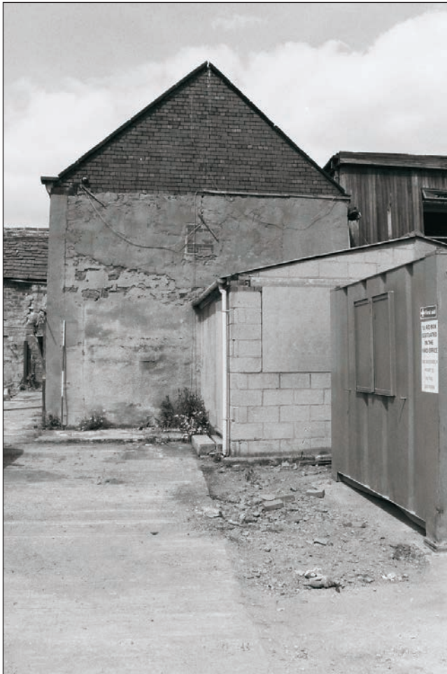
Plate 26: General view of the south elevation of the barn, Building 1, with extensions (Film 02.34)
