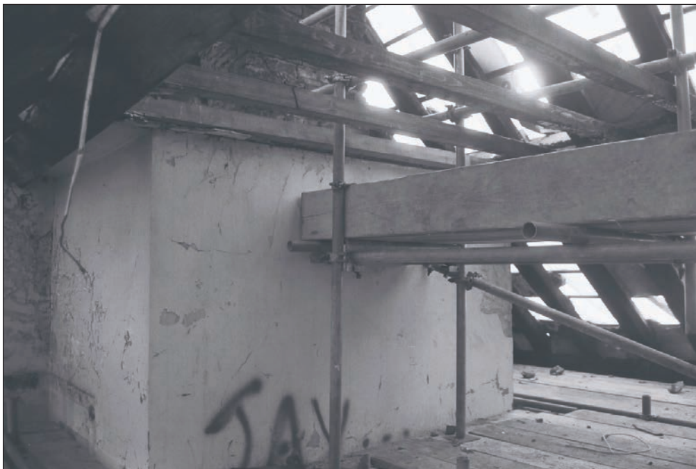
Plate 214: General view of ceiling and roof structure during watching brief, F1, Building 2 (Film 41.02)
