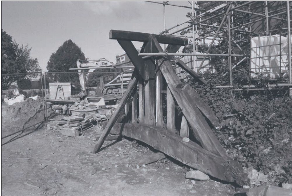
Plate 73: Detail of timber truss during the watching brief once removed from Building 1 (Film 39.13)
