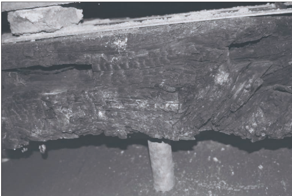
Plate 208: Detail of empty mortice holes in underside of tie beam of close stud partition for inserted door, F3, Building 2 (Film 43.03)
