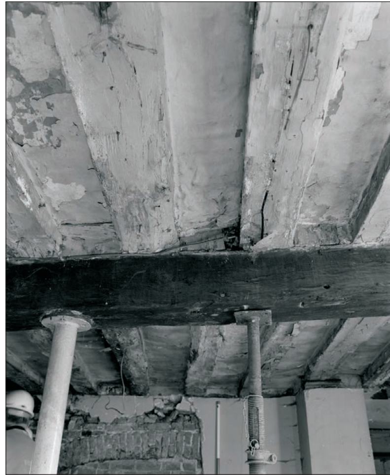
Plate 143: Detail of exposed ceiling and joists, showing joint with timber beam, G1, Building 2 (Film 31.07)
