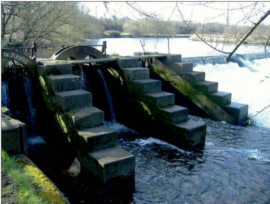
Plate 8: General view of the sluices from downstream prior to works (Client Digital 8)
