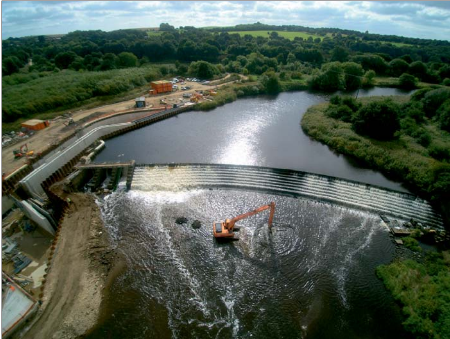
Plate 21: Aerial view of weir, sluices and new hydropower station site during works on 1st September 2016 following movement of central pier (Client Digital 21)
