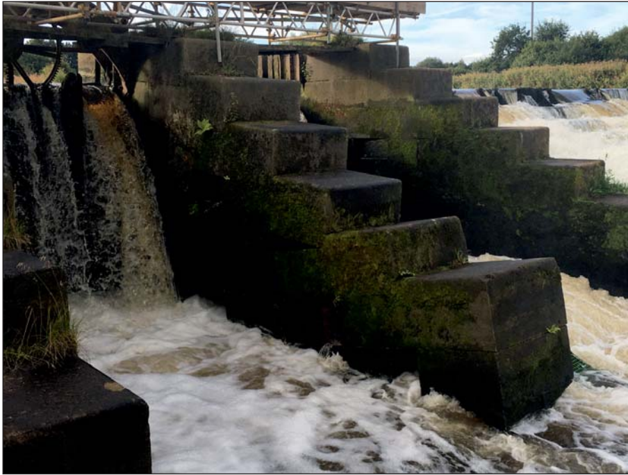
Plate 29: Downstream detail of sluice piers following subsidence of central pier (Client Digital 29)
