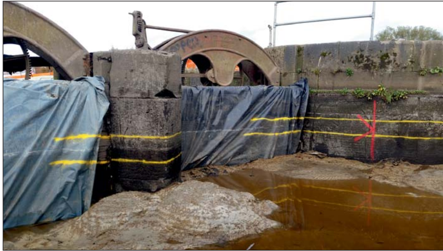
Plate 43: Detail of easternmost sluice from upstream post-piling, showing levels for new concrete slab (Client Digital 43)
