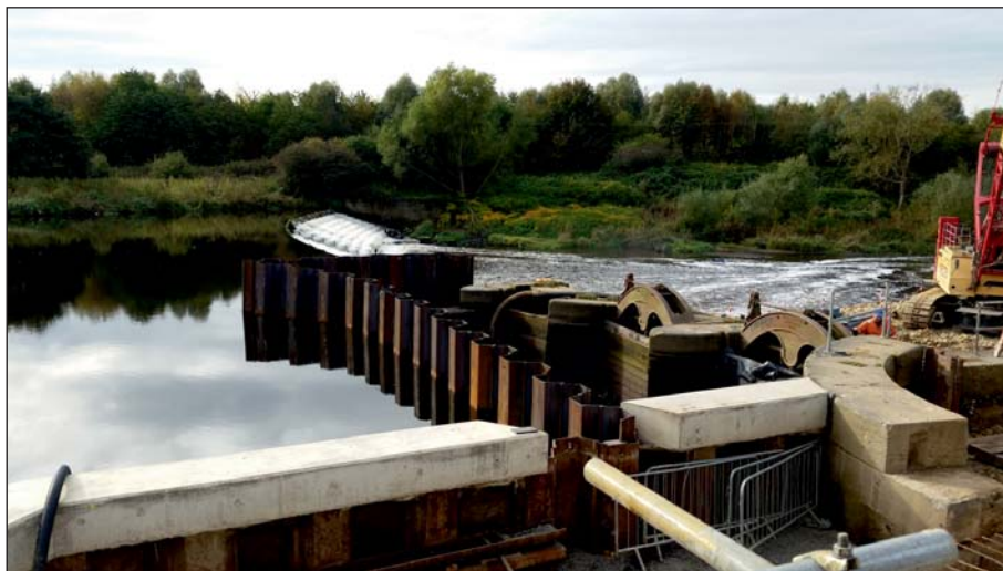
Plate 36: General view of the sluices and weir from the hydropower site, post-piling (Client Digital 36)
