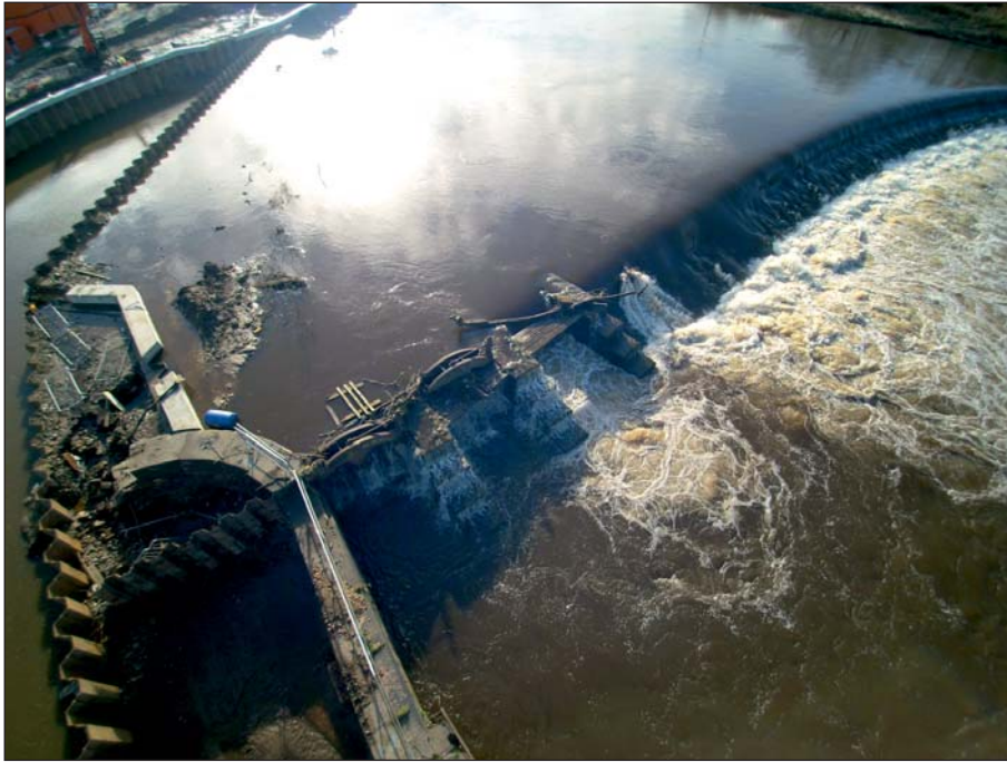
Plate 15: Aerial view of sluices and weir during high river waters during works (Client Digital 15)
