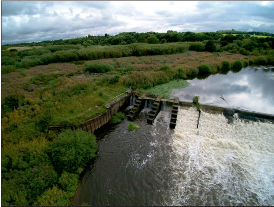
Plate 1: Aerial view of Kirkthorpe Weir showing the sluices and east wingwall prior to works (Client Digital 1)
