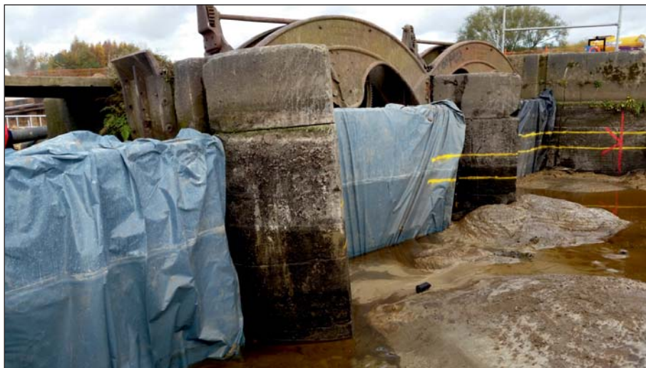
Plate 44: View of the sluices from upstream post-piling, showing levels for new concrete slab (Client Digital 44)
