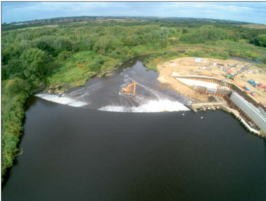
Plate 20: Aerial view of weir, sluices and new hydropower station site during works on 1st September 2016 following movement of central pier (Client Digital 20)
