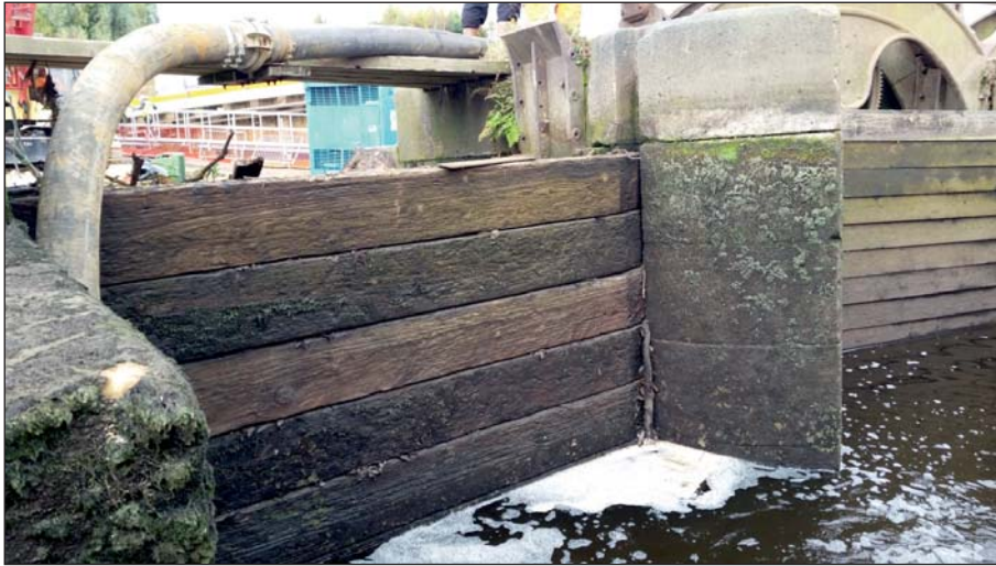
Plate 39: View of the timber boards of westernmost sluices from upstream post-piling (Client Digital 39)
