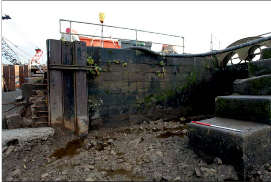
Plate 57: General view of the downstream easternmost sluice pier and wingwall (Digital IMG_0230)
