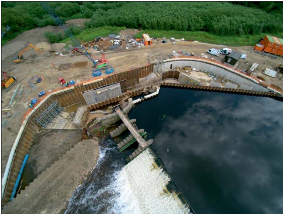
Plate 18: Aerial view of weir, sluices and new hydropower station site during works (Client Digital 18)
