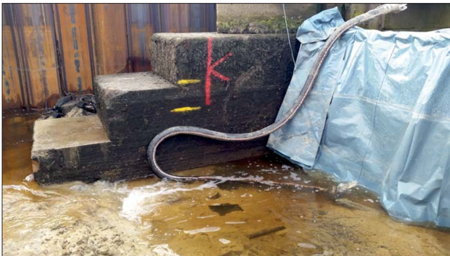
Plate 46: Detail of westernmost pier with stepped upstream side showing levels for new concrete slab (Client Digital 46)
