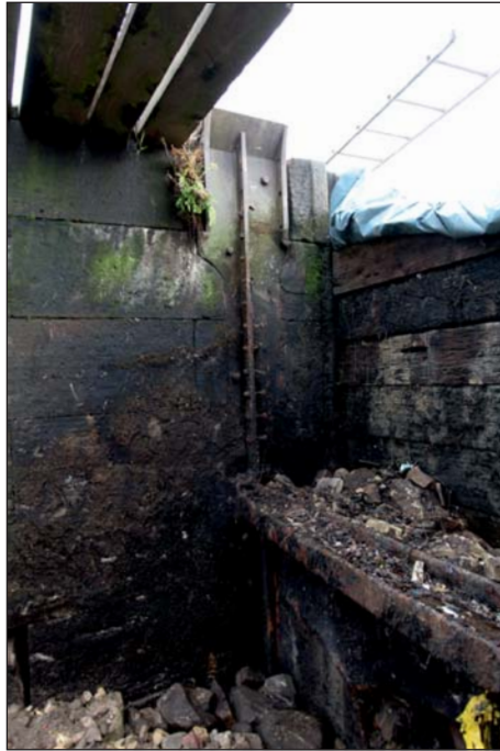
Plate 69: Detail of cast iron sluice fixings to the central pier of the westernmost sluice from downstream (Digital IMG_0244)
