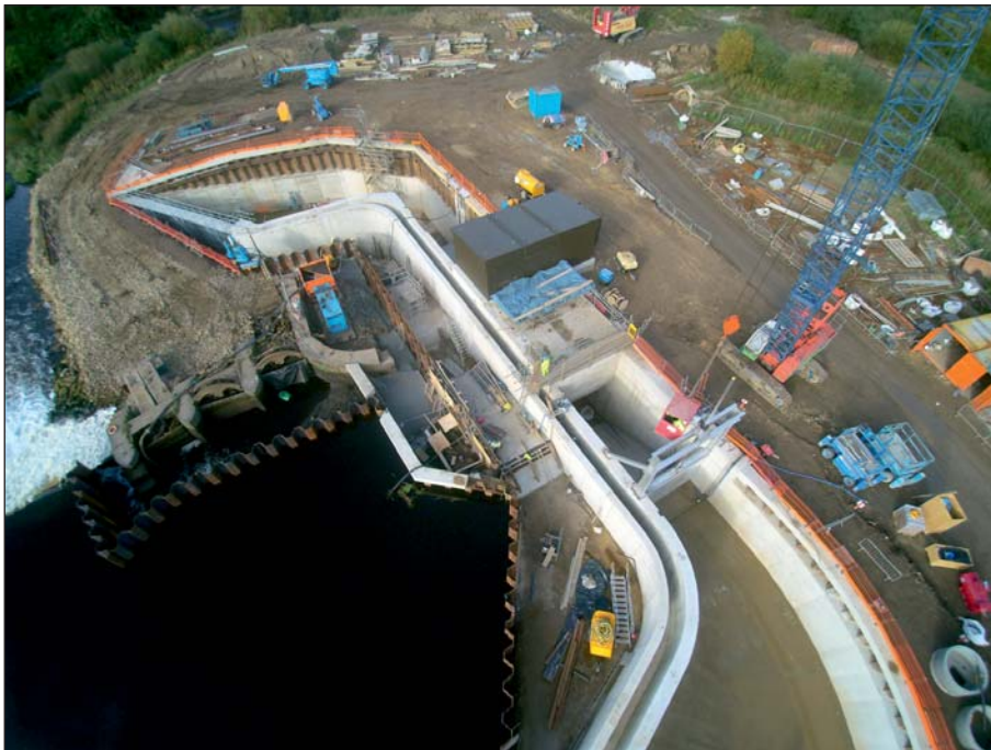
Plate 30: Aerial view of new hydropower site and adjacent wingwall and sluices post-piling (Client Digital 30)
