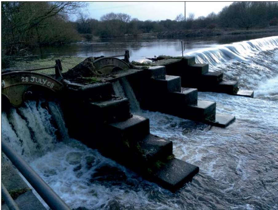
Plate 2: General view of the sluices and weir beyond prior to works (Client Digital 2)
