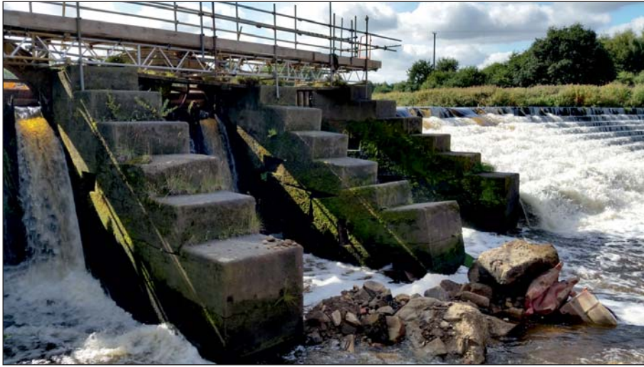
Plate 27: Downstream detail of sluice piers following subsidence of central pier (Client Digital 27)
