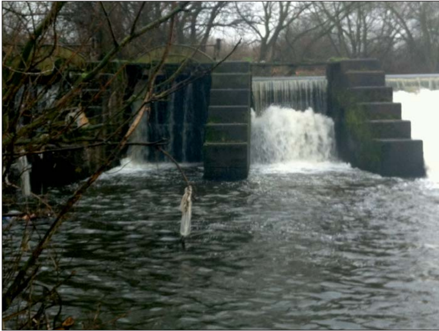
Plate 9: General view of the sluices from downstream prior to works (Client Digital 9)
