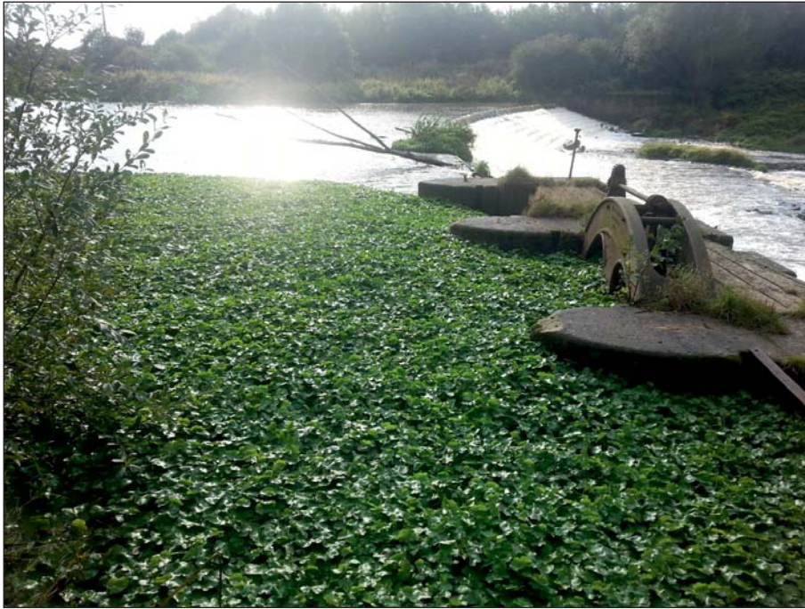
Plate 3: General view of the upstream side of the sluices with weir beyond, looking across the River Calder prior to works (Client Digital 3)
