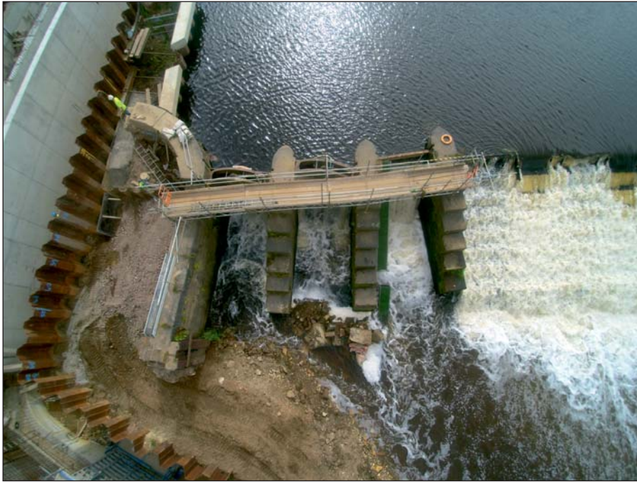
Plate 25: Aerial view of weir and sluices during works on 1st September 2016 following movement of central pier (Client Digital 25)
