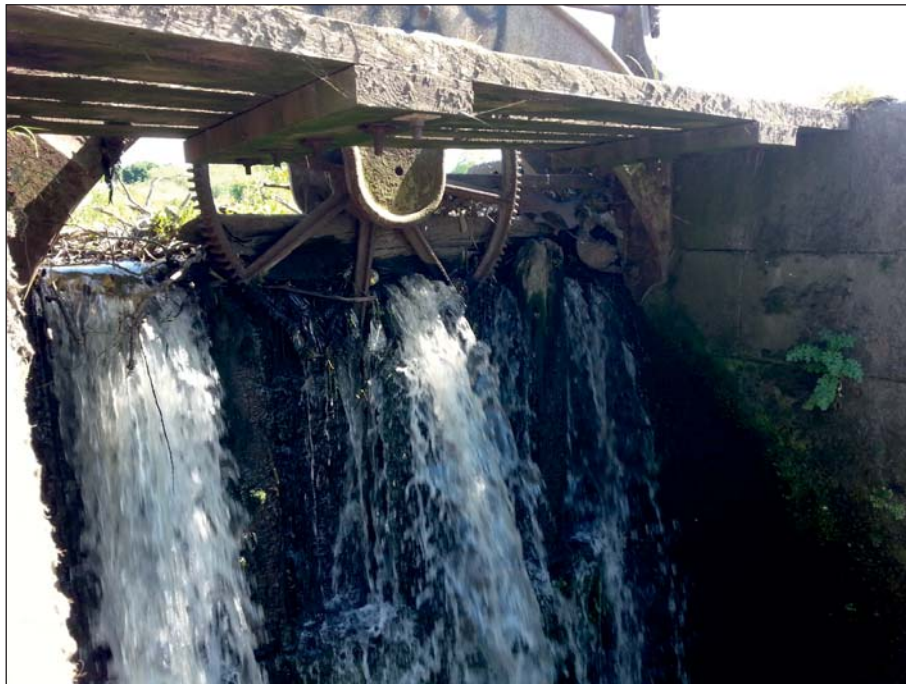
Plate 12: Detail of the central sluice and mechanism from downstream, prior to works (Client Digital 12)
