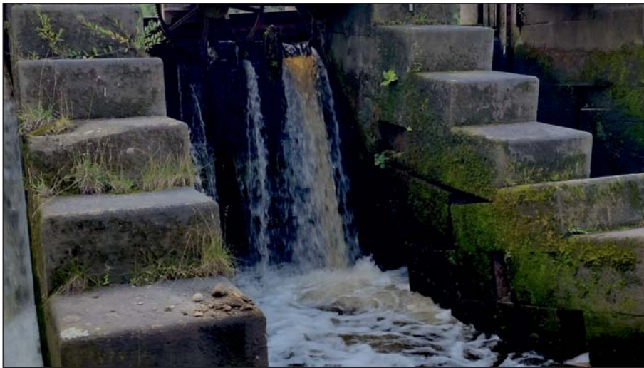
Plate 28: Downstream detail of central sluice and damage to pier (Client Digital 28)
