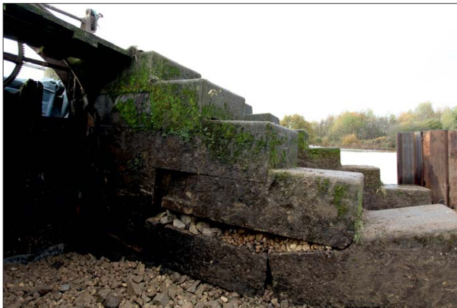
Plate 62: View of the east elevation of the central pier within the central sluice, showing recess and collapse damage (Digital IMG_0248)
