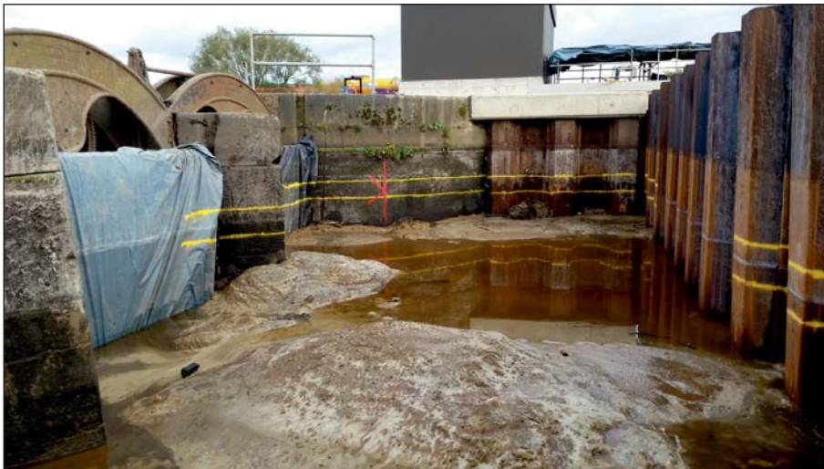
Plate 42: View of the sluices from upstream post-piling, showing levels for new concrete slab (Client Digital 42)
