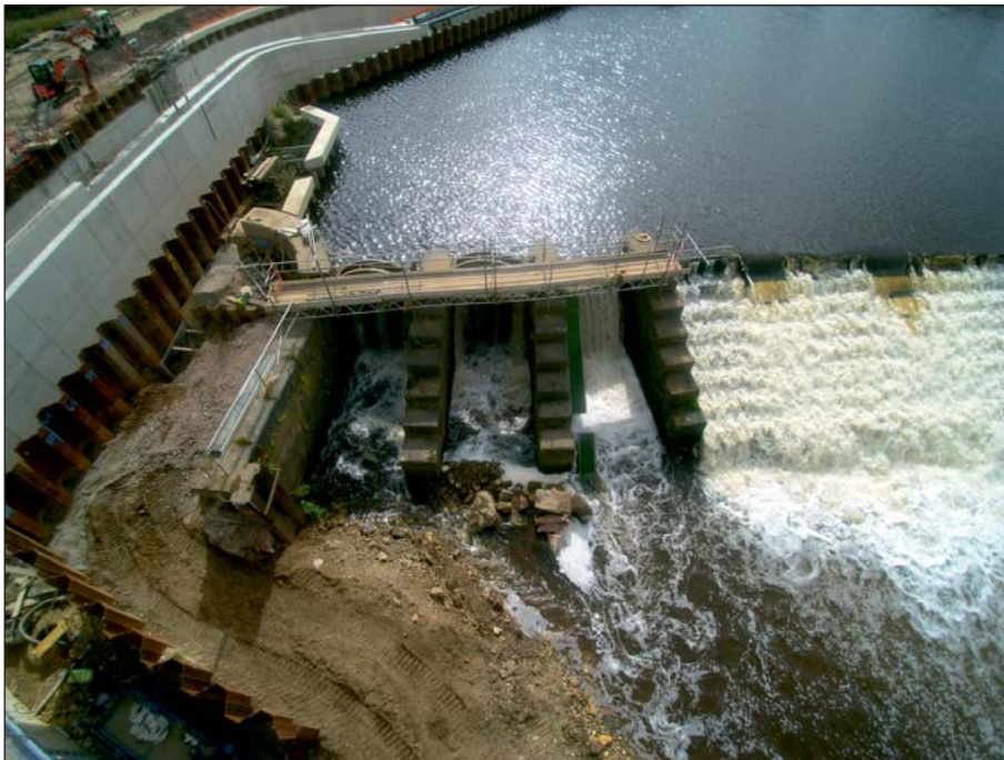
Plate 26: Aerial view of weir and sluices during works on 1st September 2016 following movement of central pier (Client Digital 26)
