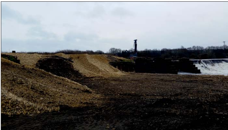
Plate 14: General view of sluices from downstream following commencement of works (Client Digital 14)
