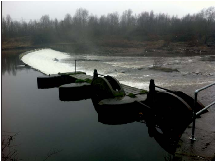
Plate 6: View of the sluices and weir from upstream prior to works (Client Digital 6)
