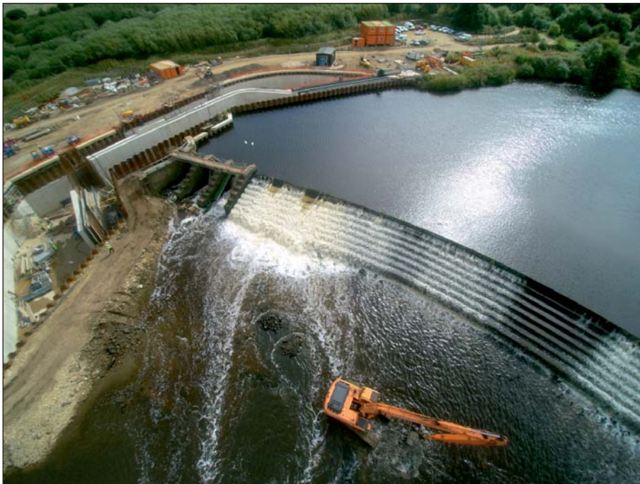
Plate 22: Aerial view of weir, sluices and new hydropower station site during works on 1st September 2016 following movement of central pier (Client Digital 22)
