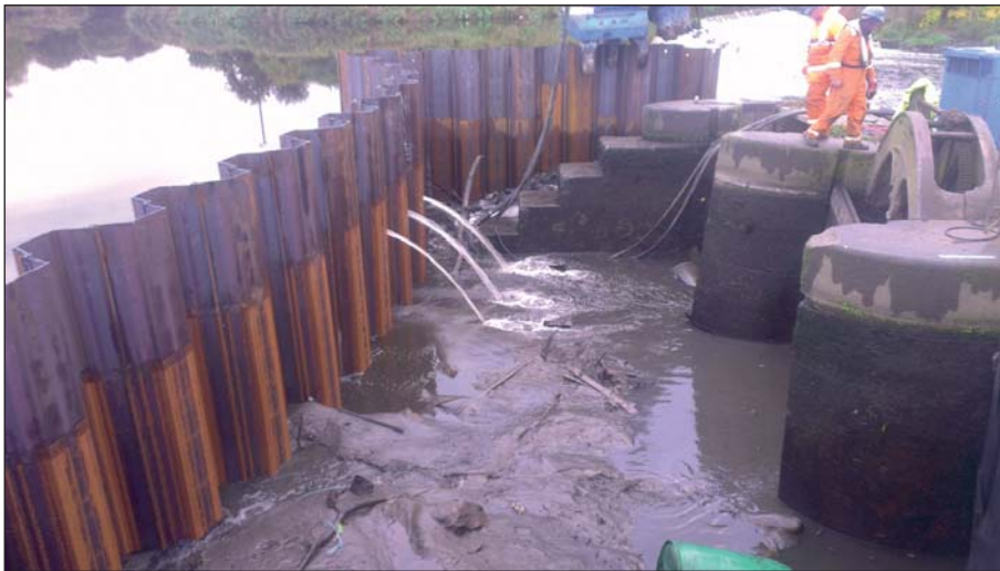
Plate 40: View of the sluices from upstream showing westernmost stepped pier upstream side post-piling (Client Digital 40)
