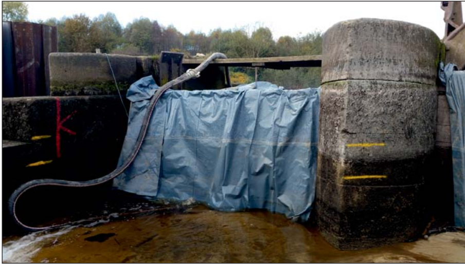
Plate 45: Detail of westernmost sluice from upstream post-piling, showing levels for new concrete slab (Client Digital 45)
