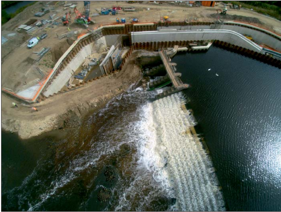
Plate 23: Aerial view of weir, sluices and new hydropower station site during works on 1st September 2016 following movement of central pier (Client Digital 23)
