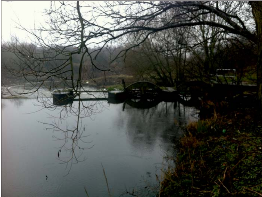
Plate 7: View of the sluices and weir from upstream prior to works (Client Digital 7)
