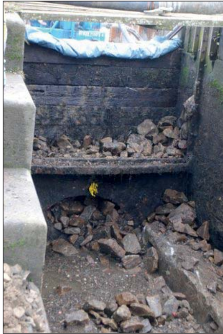
Plate 47: Detail of exposed arched opening at the base of the westernmost sluice from downstream (Client Digital 47)
