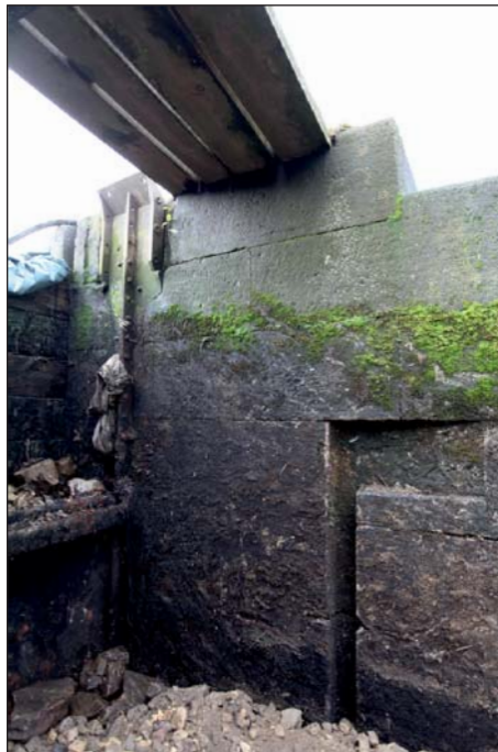
Plate 68: Detail of sluice recess with angle within the western pier of the westernmost sluice from downstream (Digital IMG_0242)
