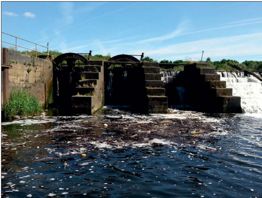
Plate 10: General view of the sluices from downstream prior to works (Client Digital 10)
