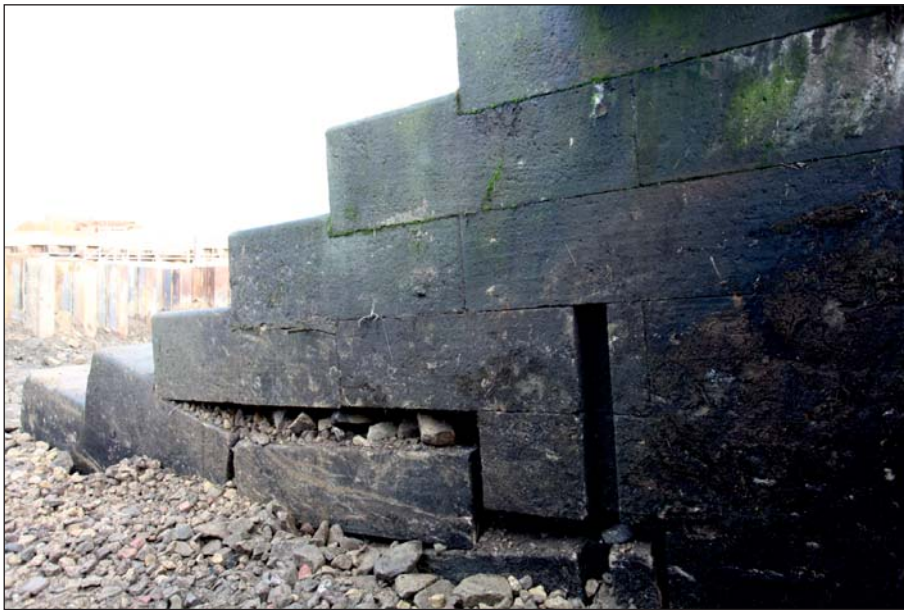
Plate 66: Detail of the west elevation of the central pier within the westernmost sluice, showing recess and collapse damage from downstream (Digital IMG_0245)
