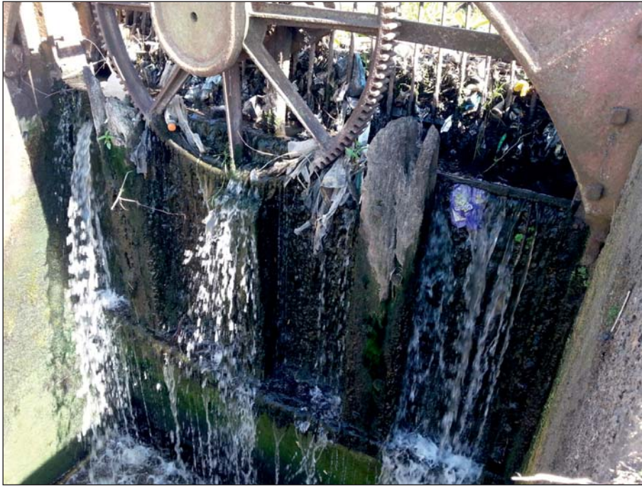
Plate 13: Detail of easternmost sluice and mechanism from downstream, prior to works (Client Digital 13)
