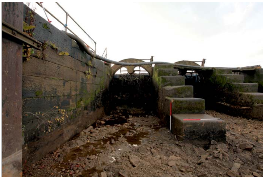
Plate 58: General view of the easternmost sluice with pier and wingwall from downstream (Digital IMG_0227)
