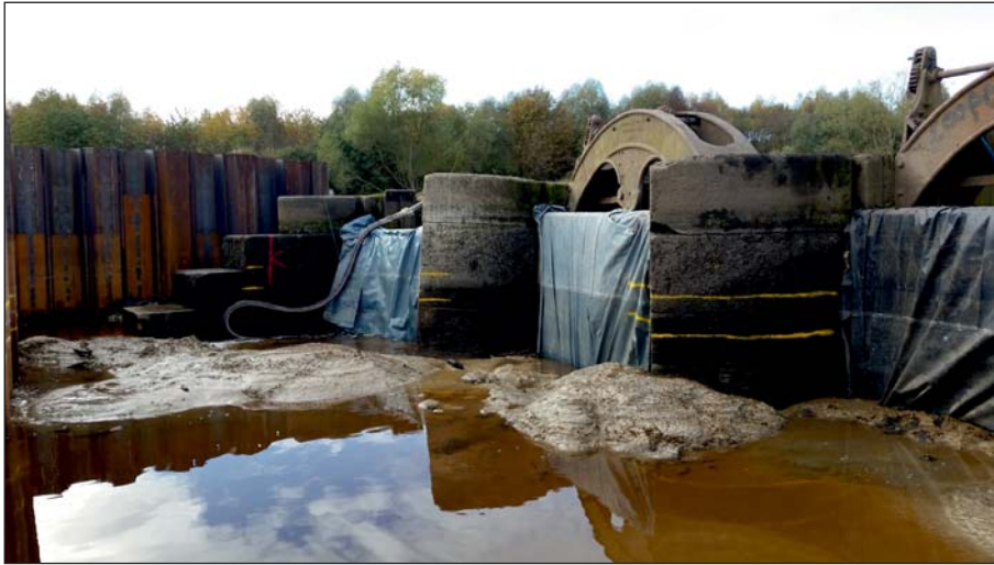
Plate 41: View of the sluices from upstream post-piling, showing levels for new concrete slab (Client Digital 41)
