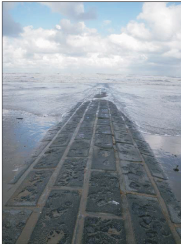
Plate 15: Example of a modern breakwater dating from the 1960's, near Blankenberge, facing NW
