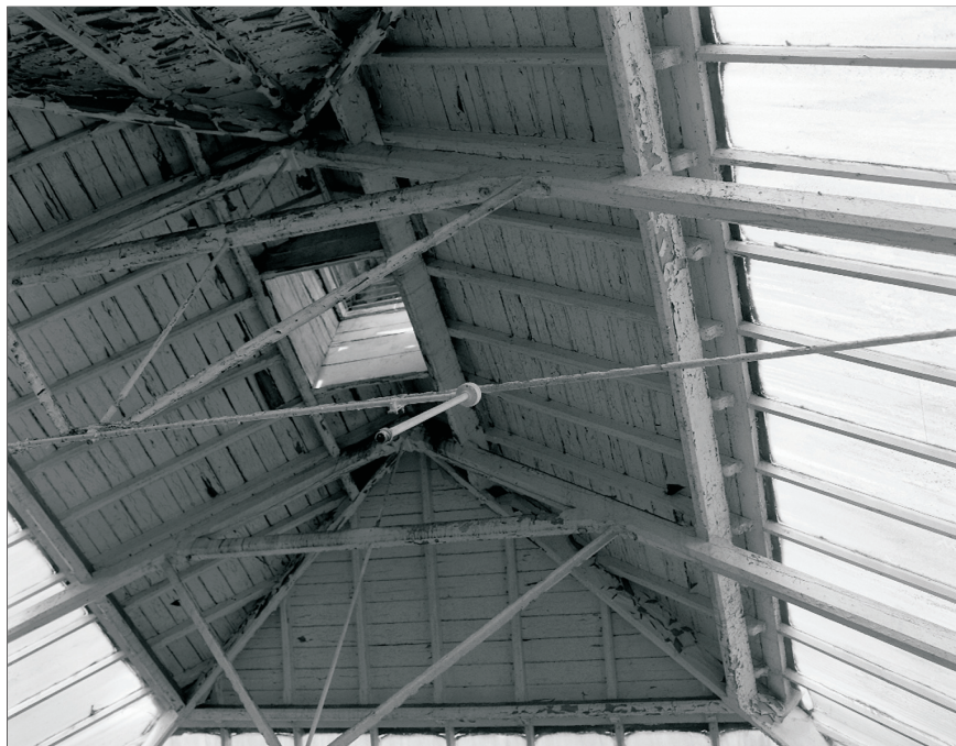
Plate 26: Detail of timber and iron trussed pyramidal roof of G1, showing glazed lower section, Building 1 (film 6.3)
