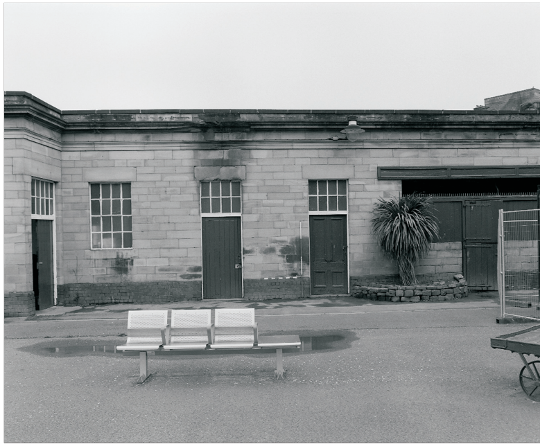
Plate 10: General view of west elevation of Building 2, showing doorways to G3, G4 and G5 and heat damaged stonework (film 1.3)
