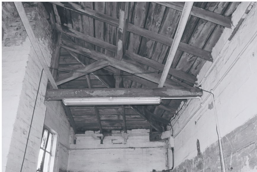
Plate 41: Detail of timber trusses, with hip to the north, G5, Building 2 (film 7.13)
