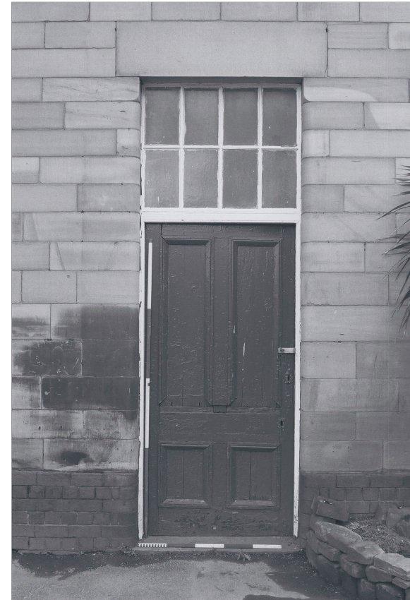
Plate 15: Detail of timber panelled door with over-light to G3, west elevation of Building 2 (film 7.17)
