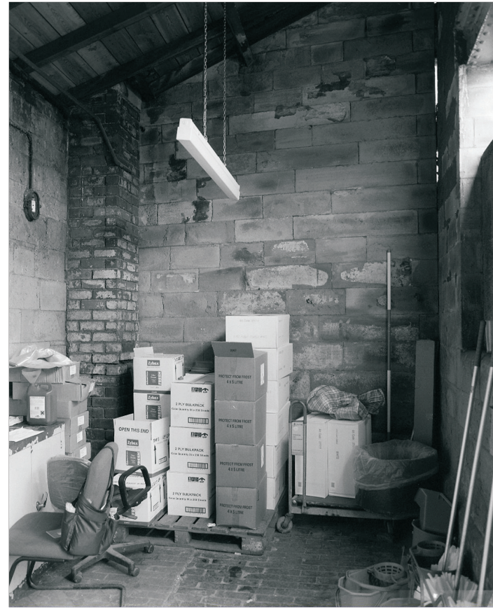
Plate 28: General view of G2, Building 2 showing brick chimney flue in south-east corner (film 2.3)
