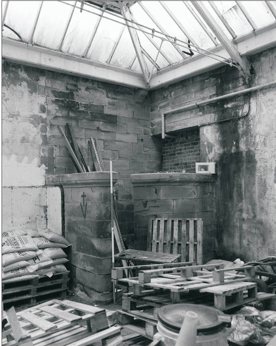
Plate 20: General view of G1, showing ashlar baffle partitions and blocked doorway (film 5.5)
