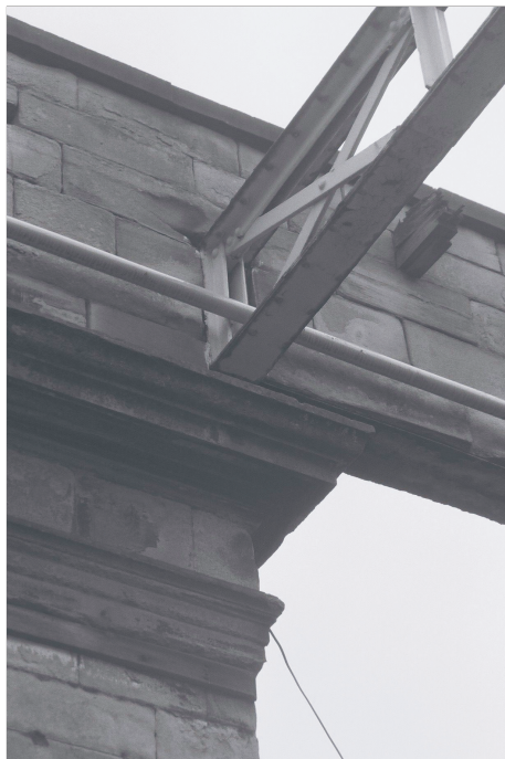
Plate 6: Detail of lattice girder of former platform roofing attached to parapet of Building 1 (film 7.30)
