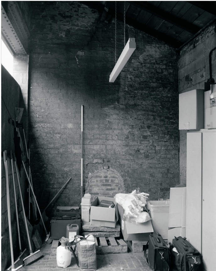
Plate 29: General view of G2, showing blocked arched opening in north wall, Building 2 (film 2.2)
