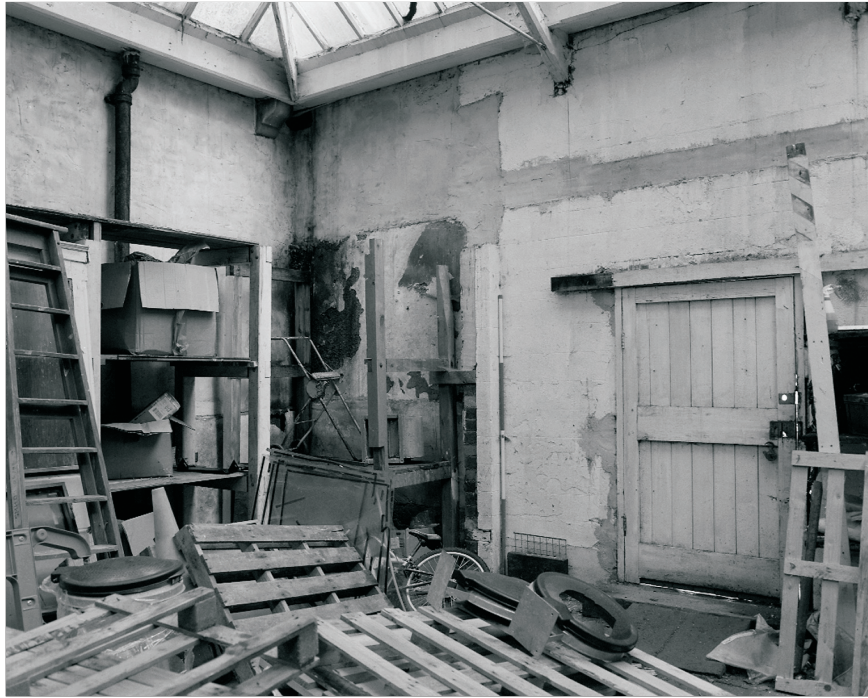
Plate 25: General view of north-east corner of G1, showing modern doorway in east wall and scars of former toilet cubicles, Building 1 (film 6.1)
