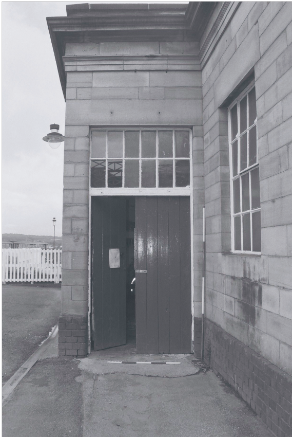
Plate 14: Detail of doorway, with over-light, to G5 in south elevation of stepped north end of Building 2 (film 7.10)
