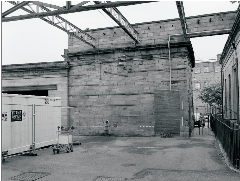
Plate 5: General view of west elevation of Building 1 showing blocked doorway and raised parapet with remains of former platform roofing (film 1.7)
