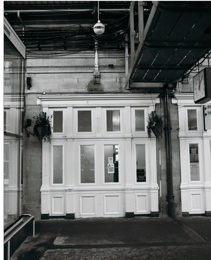
Plate 30: View of northernmost double door/window from Booking Hall to platforms, west elevation of Central Block (film 4.1)
