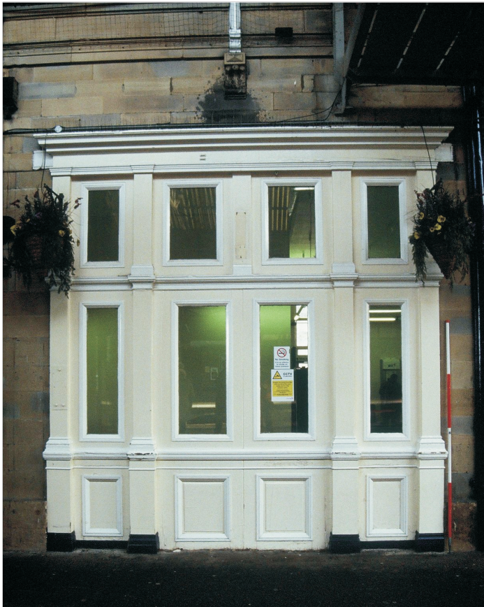
Plate 31: View of northernmost double door/window from Booking Hall to platforms, west elevation of Central Block (film 7.9)
