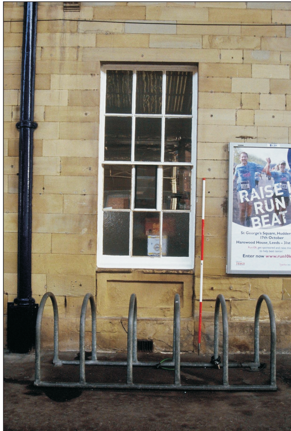
Plate 19: Detail of altered door to window, west elevation of South Wing (film 7.5)
