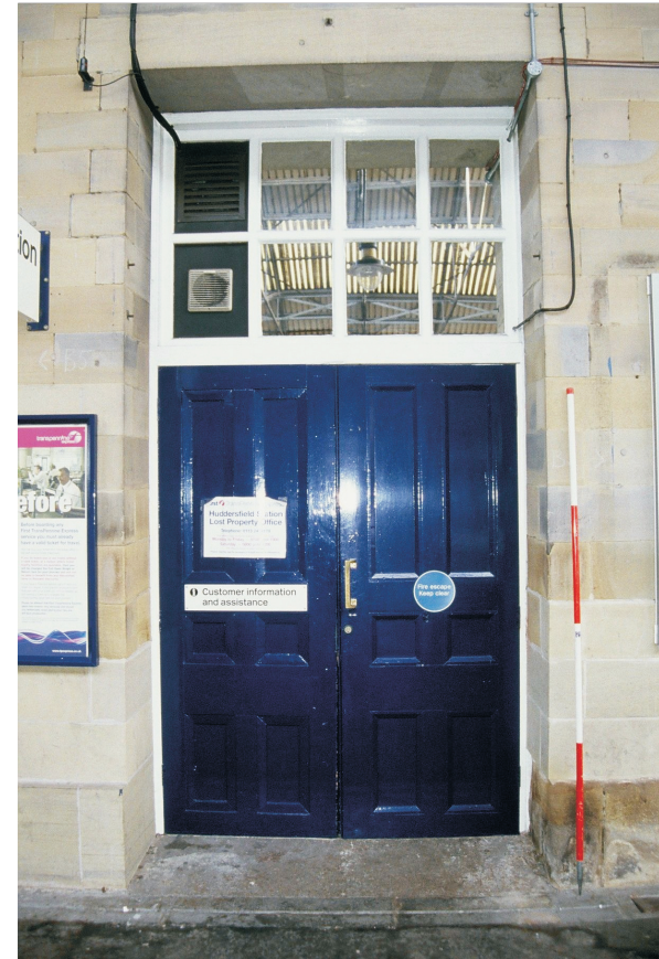
Plate 24: Detail of altered window to double door, west elevation of Central Block (film 7.8)
