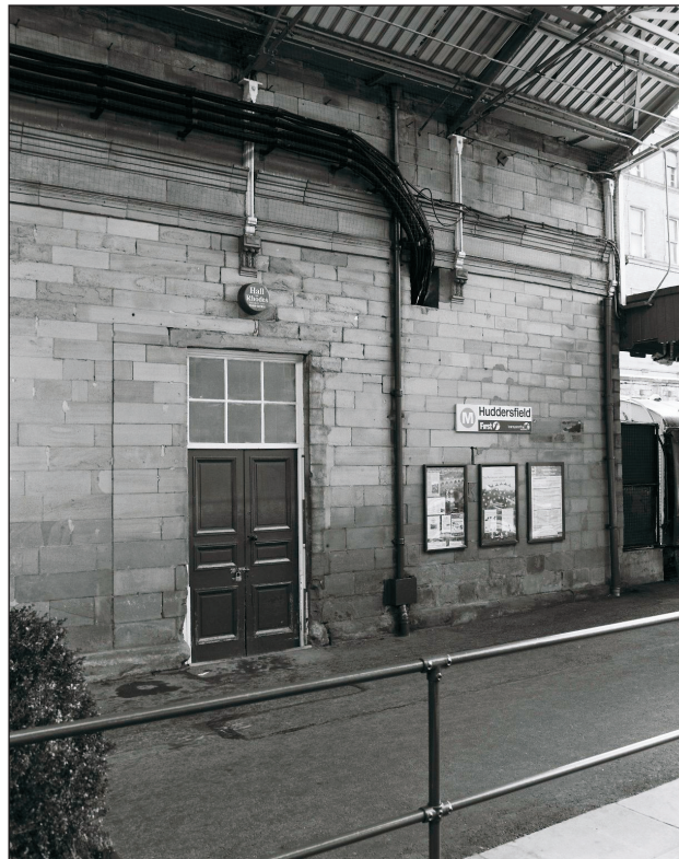
Plate 10: View of west elevation of later southern toilet block, showing inserted door (film 1.1)
