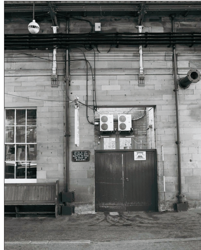
Plate 12: Detail of passageway between southern extent of South Wing and later southern toilet block, west elevation (film 1.6)
