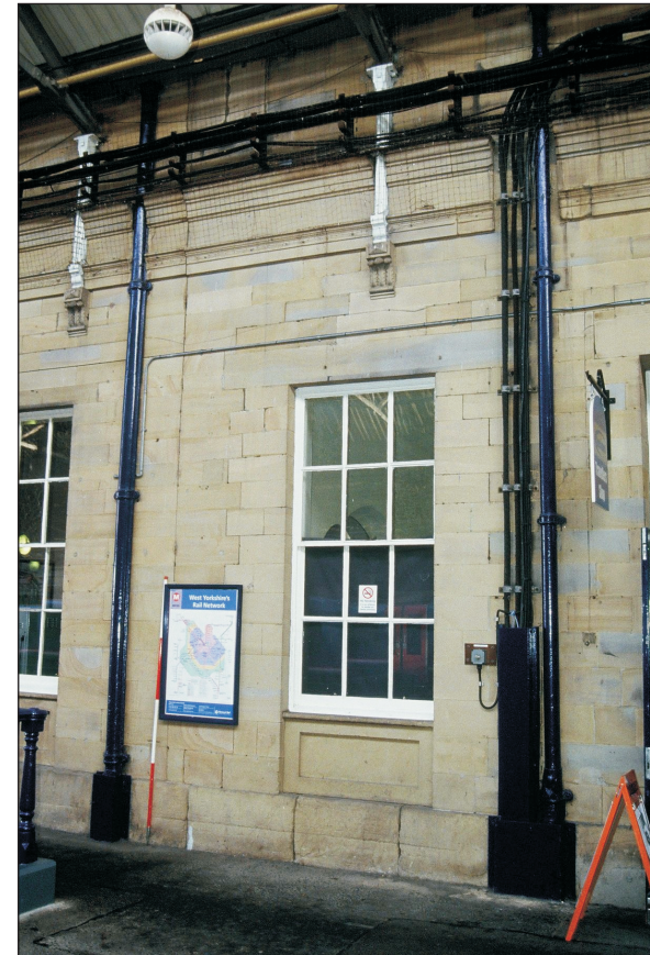
Plate 34: View of reinstated window and vertical joint in stonework delineating join between Central Block and North Wing, west elevation (film 7.3)
