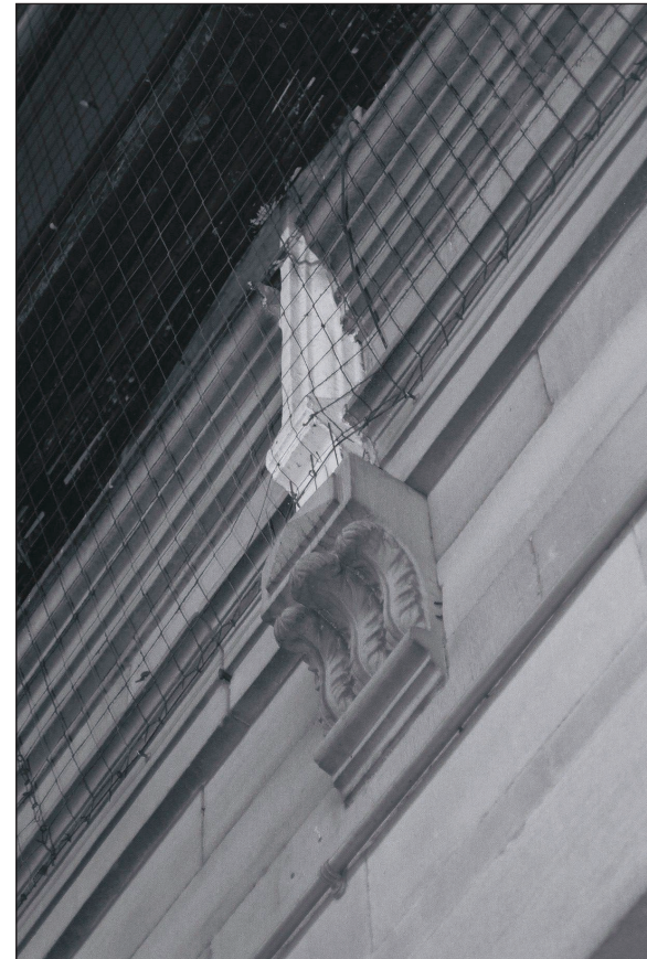
Plate 38: Detail of inserted decorative stone corbel supporting secondary roof structure over platform (film 6.29)
