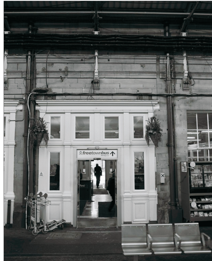
Plate 28: View of southernmost double door main entrance from Booking Hall to platforms, west elevation of Central Block (film 3.8)
