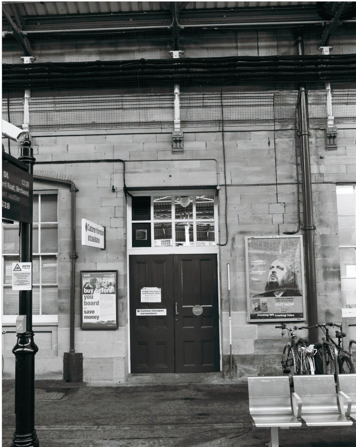
Plate 23: View of altered window to double door and vertical joint in stonework between Central Block & South Wing, west elevation (film 3.1)
