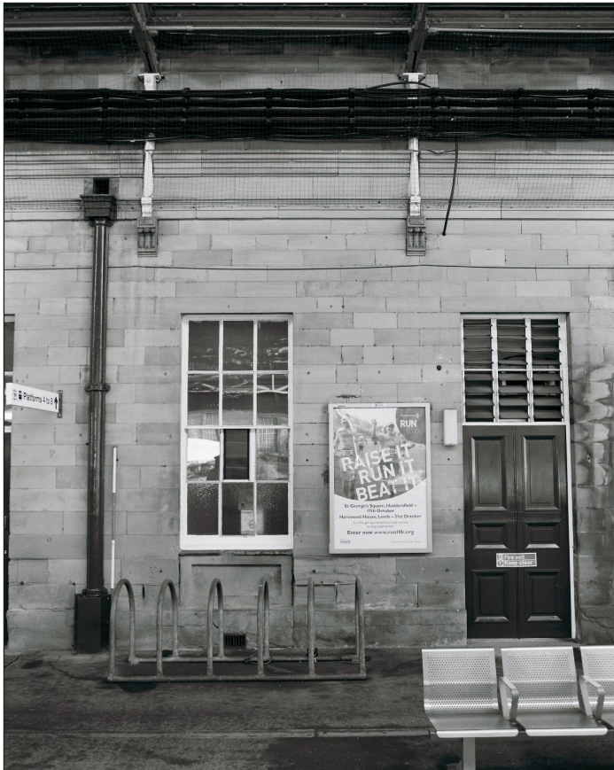
Plate 17: View of primary door and altered door to window, west elevation of South Wing (film 2.6)
