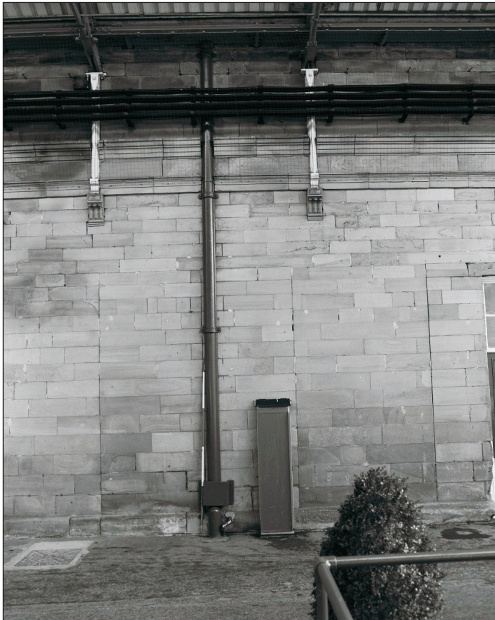
Plate 11: View of west elevation of later southern toilet block showing blocked door (film 1.3)
