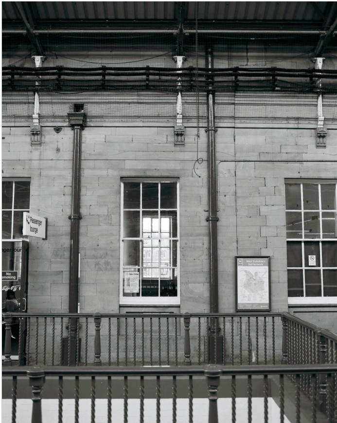
Plate 35: View of primary window and vertical joint in stonework delineating join between Central Block and North Wing, west elevation (film 4.6)
