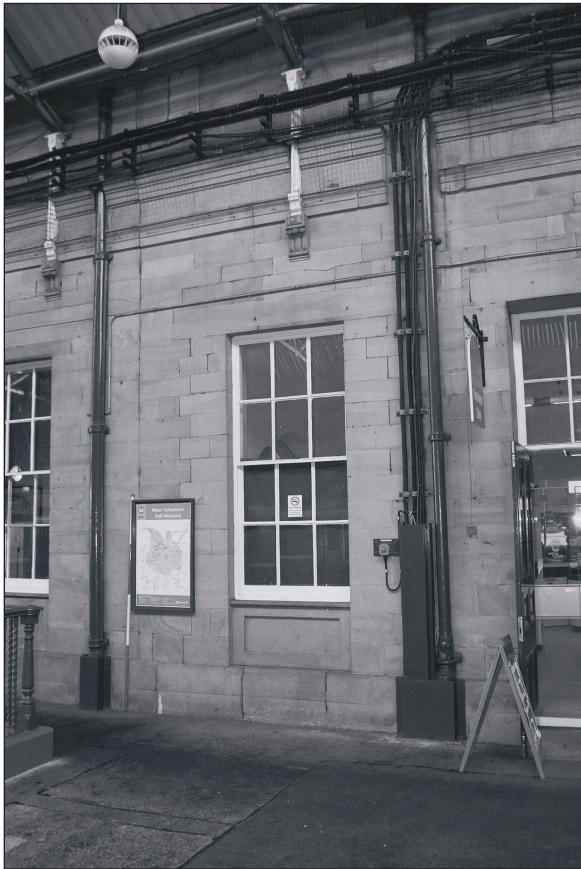
Plate 33: View of reinstated window and vertical joint in stonework delineating join between Central Block and North Wing, west elevation (film 6.16)
