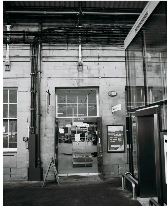
Plate 32: View of primary door, north end of west elevation of Central Block (film 4.4)
