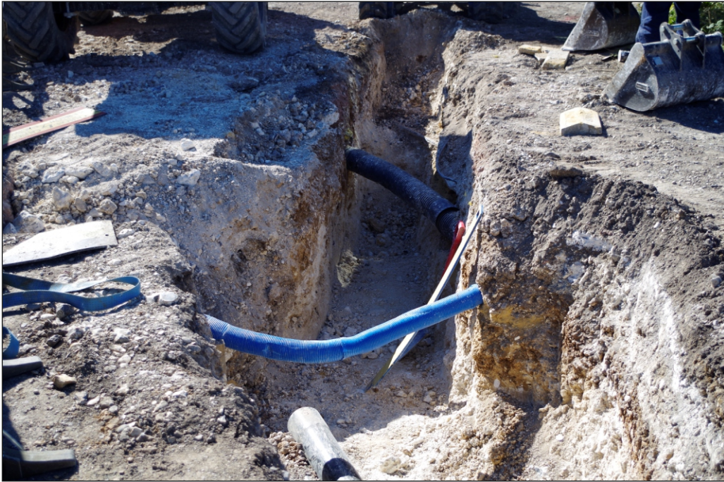
Plate 1: Exposed services in trench near the substation, view from north east
