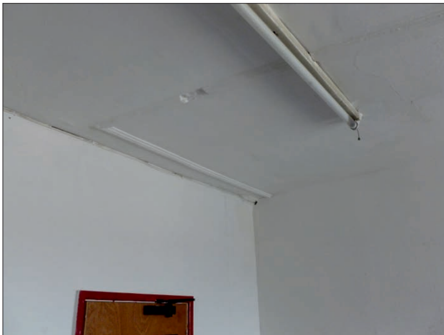
Plate 64: Detail of remnant of cornice in north end of Room 3F1
