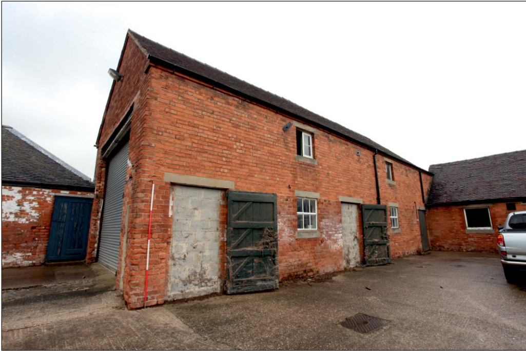
Plate 61: Building 5 viewed from the south-east. Note the blocked doors
