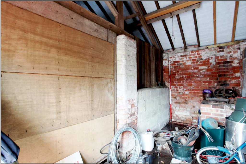
Plate 45: View of G12, Building 2, showing dividing partition with G11 and the King-post truss overhead
