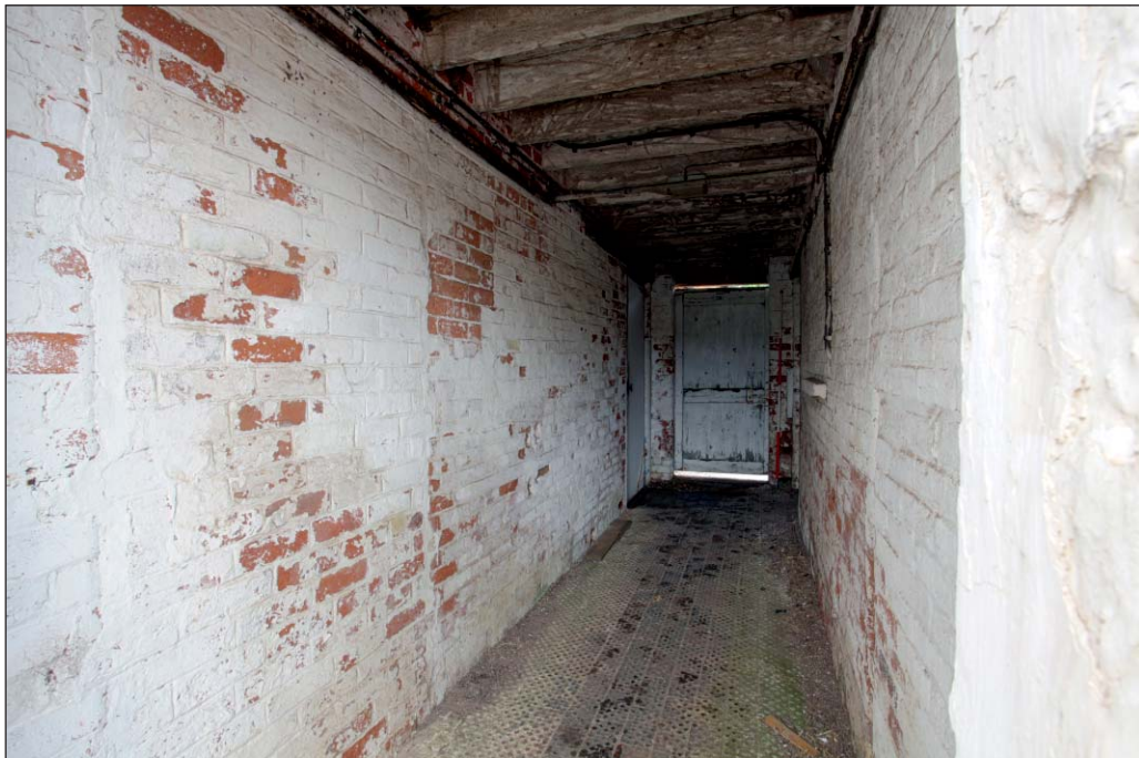
Plate 64: Passage G29, Building 5, viewed from the west. Note the opposing blocked doors in the foreground
