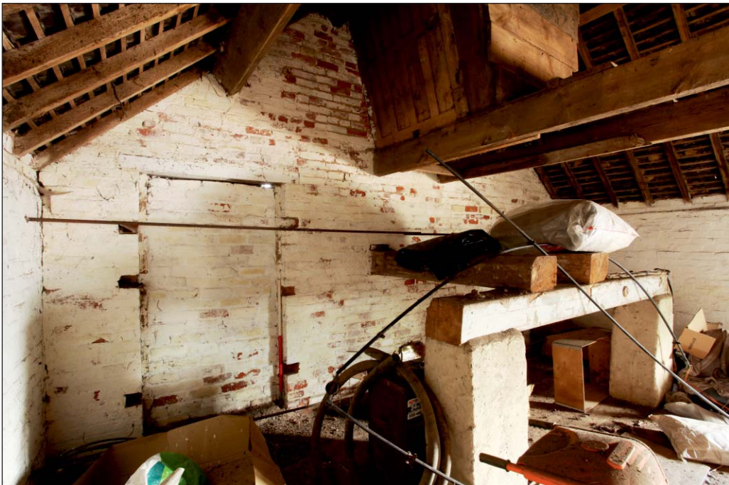
Plate 66: F08, Building 5, viewed from the south-west, showing the hopper overhead, the support platform and blocked door
