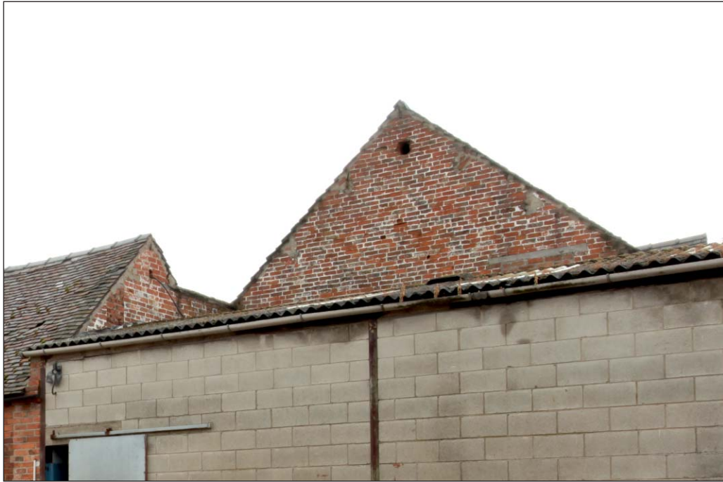
Plate 63: Building 3 west gable and Building 5 north gable viewed from the north-west. Note the partially visible blocked first floor door in the latter
