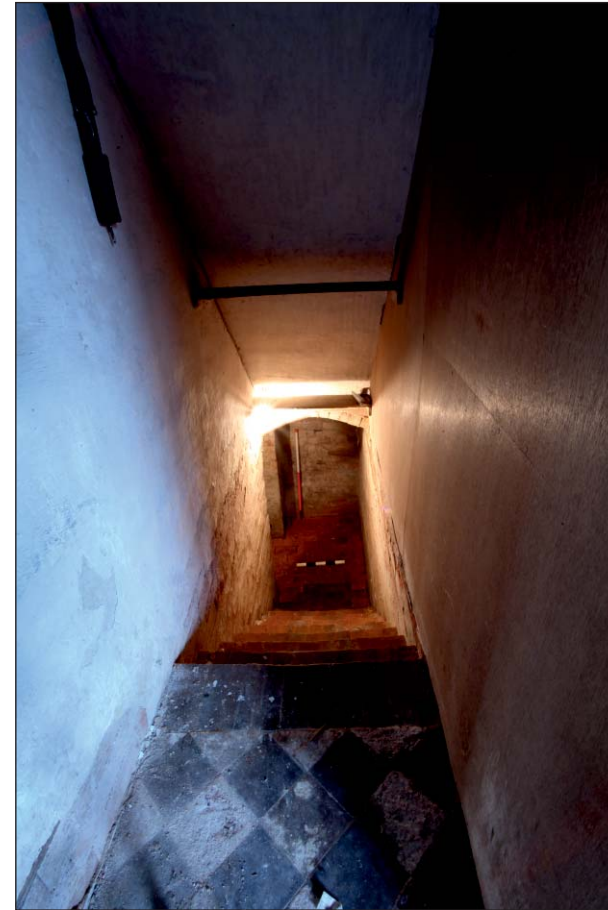
Plate 6: View down basement stairwell, Building 1, showing quarry tiles at the stair head
