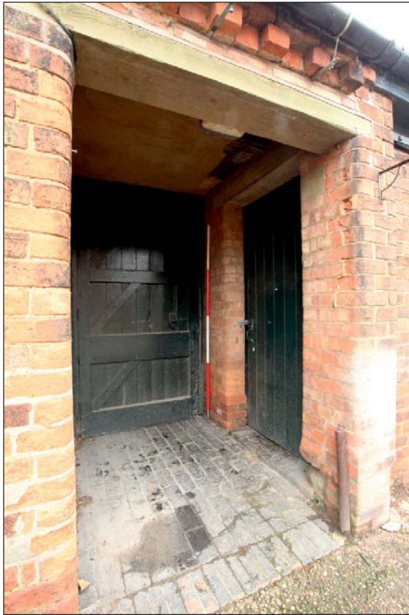
Plate 37: View of Building 2, north end showing the entrance to G08 (right) and the garden (left) within the covered passage. Viewed from the north-east
