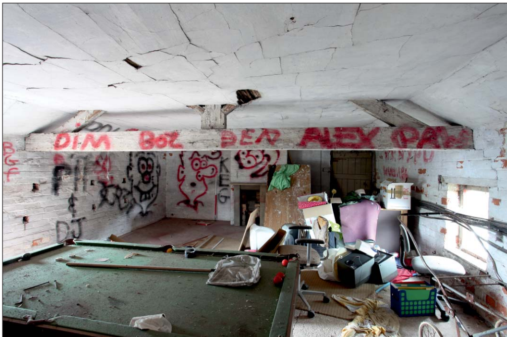
Plate 34: View of the west wing room F07, Building 1, partially showing the King-post roof truss
