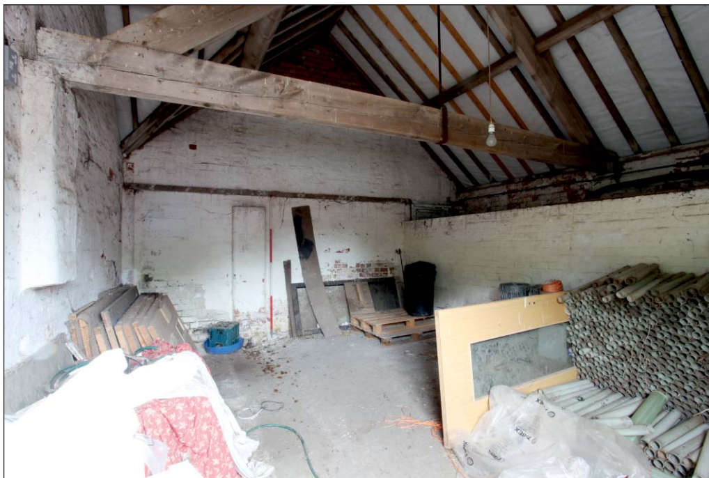
Plate 74: View of G17, Building 6, from south-east. The half wall (right) separates it from G16
