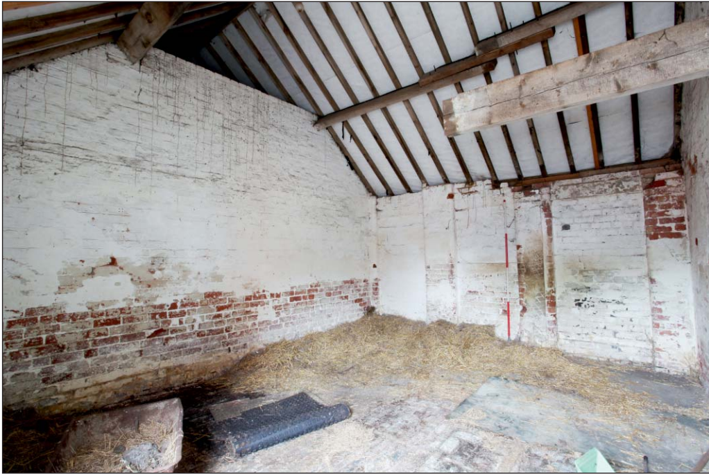
Plate 75: View of G18, Building 6, from the north-east. Note the stepped and bolted join in the purlins overhead and blocked doors and window in the west wall
