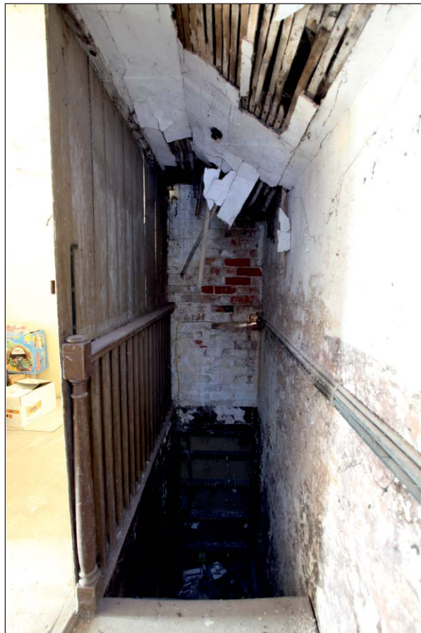
Plate 33: View of west wing blocked stairwell at the south end of F06, Building 1
