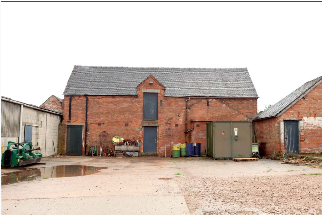
Plate 62: Building 5 viewed from the west. Note the pitched roof scar of a demolished building
