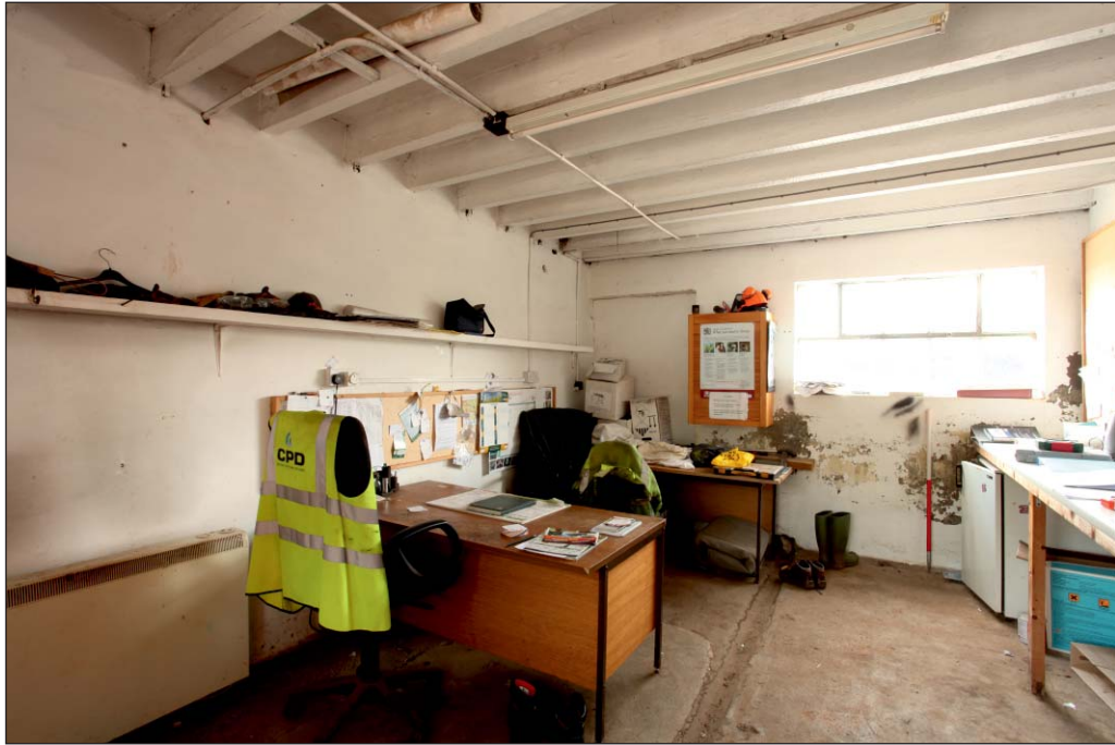
Plate 25: View of office G25 in the west wing, Building 1. Note the blocked door and drainage channel
