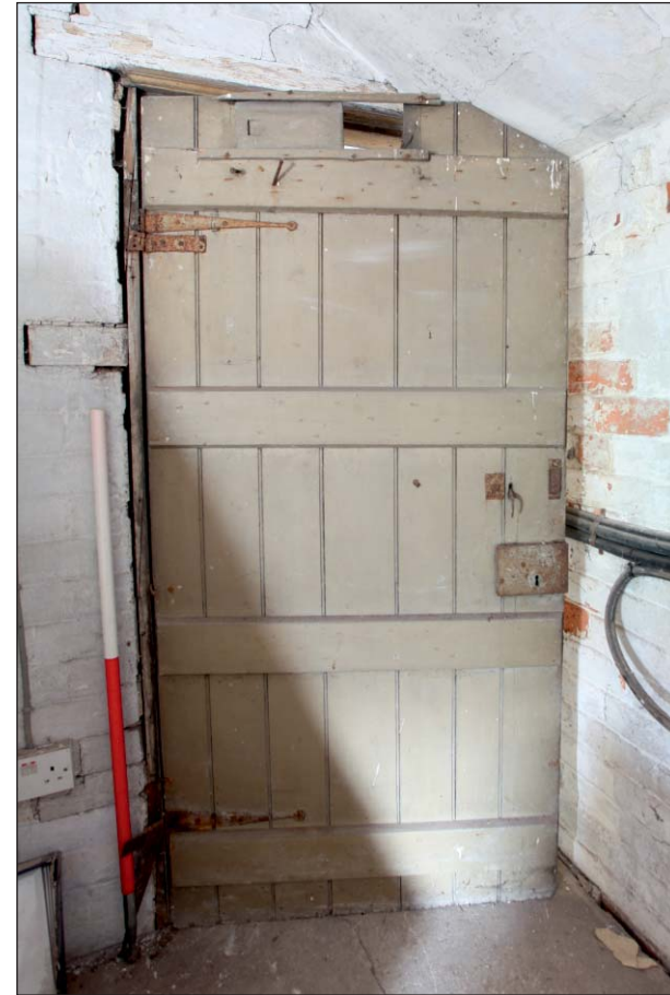
Plate 36: Detail of timber plank and batten door between F07 and F06, west wing of Building 1
