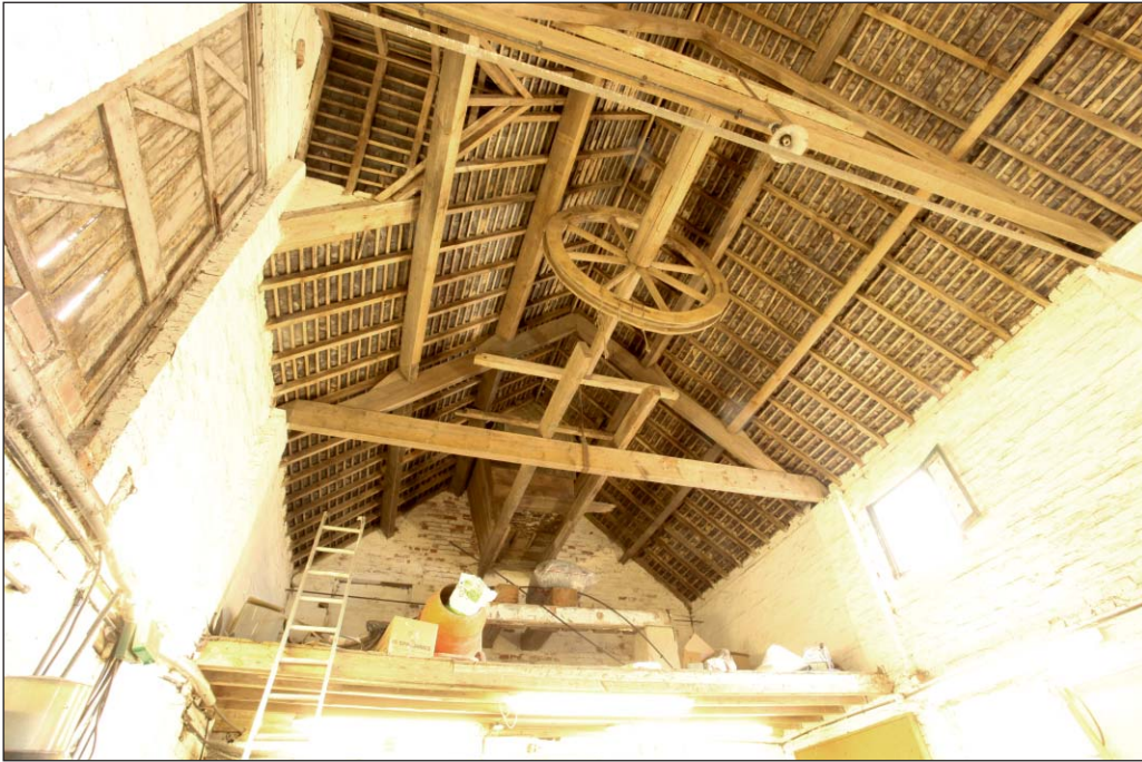
Plate 67: Building 5 roof structure with the wheel mechanism and hopper viewed from the south
