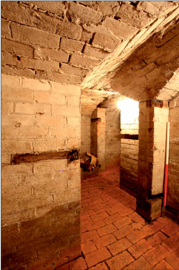
Plate 9: Remnants of door fittings and voids from removed timbers in the door openings within the basement of Building 1
