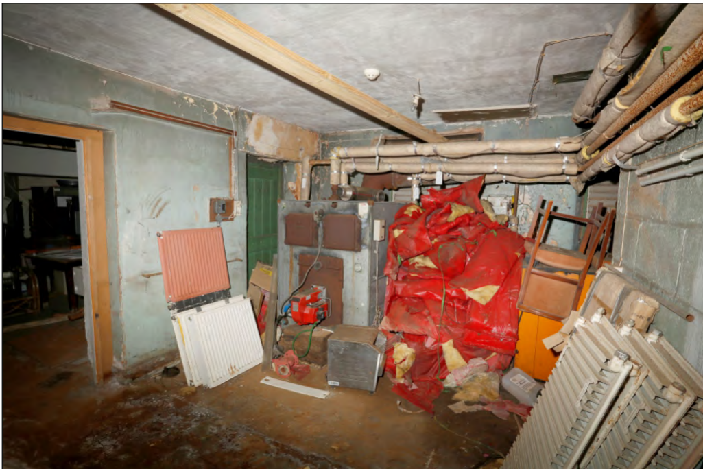
Plate 16: Lower ground floor boiler room LG02
