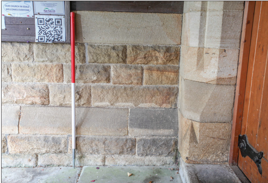
Plate 8: Detail of the masonry to be partially removed to enable the insertion of a doorway
