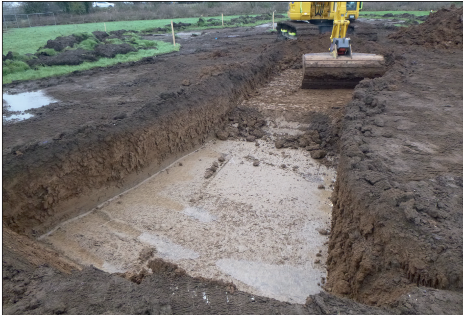
Plate 2: Trench excavated down to alluvial deposits. Showing topsoil, subsoil, possible palaeochannel infill and alluvium at the base
