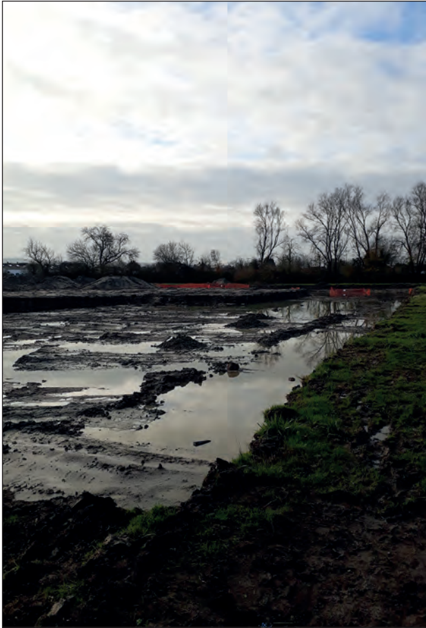
Plate 3: Working/site conditions following rainfall and groundwater ingress: south-west facing view from the northern edge of the excavation area
