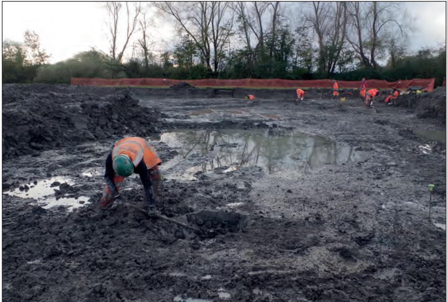
Plate 2: Working/site conditions at the start of the fieldwork: west-facing view during excavation of ditches in north-east corner of the site
