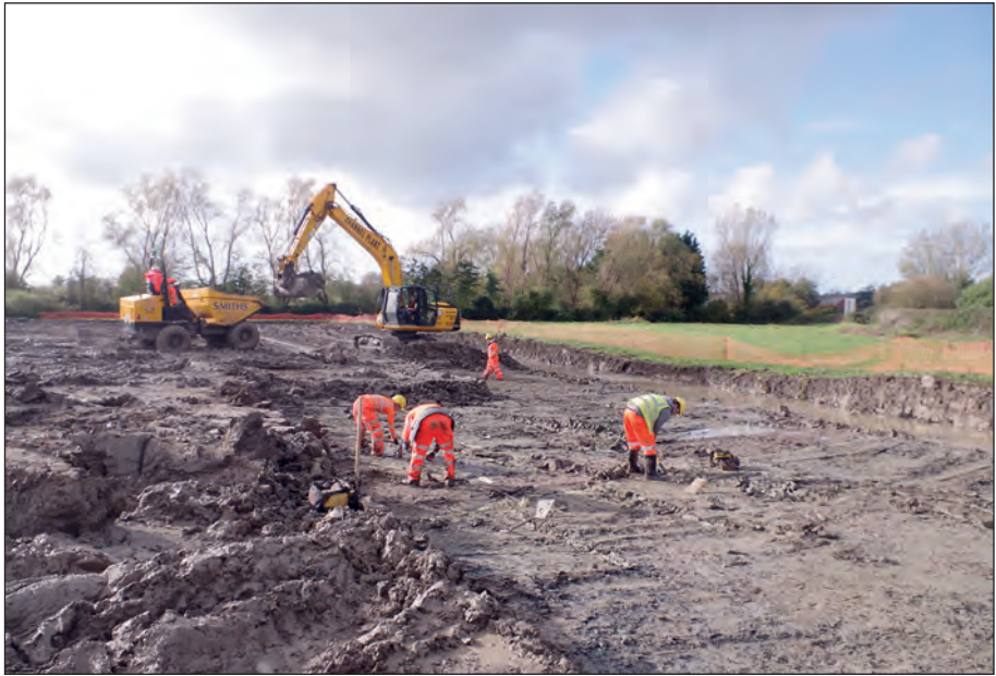
Plate 1: Working/site conditions at the start of the fieldwork: west-facing view during excavation of ditches in north-east corner of the site
