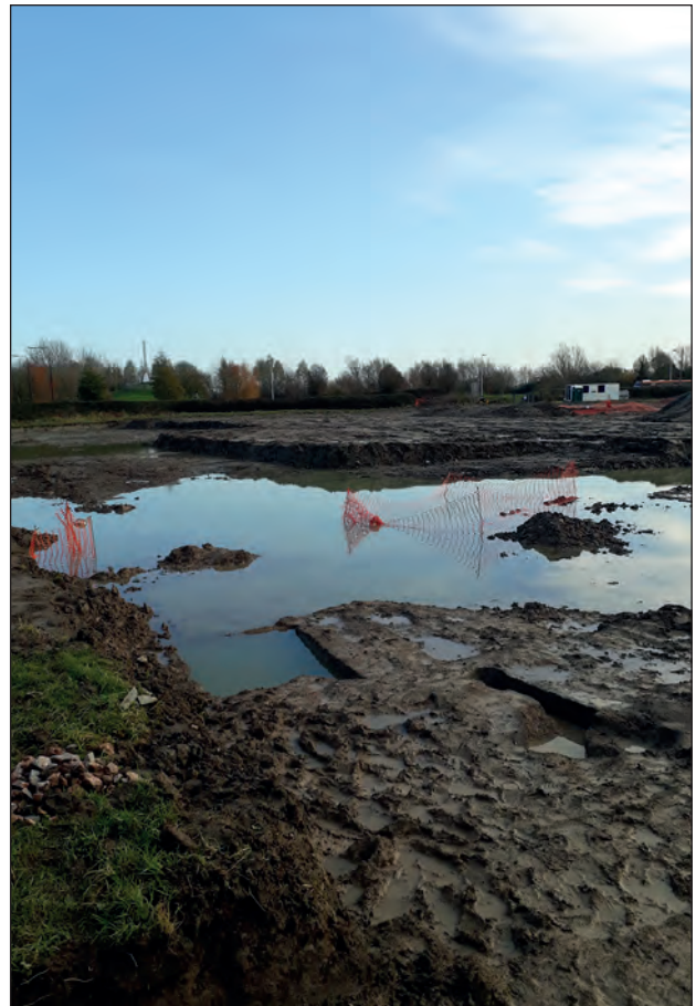
Plate 4: Working/site conditions following rainfall and groundwater ingress: east facing view from the north-west corner of the excavation area
