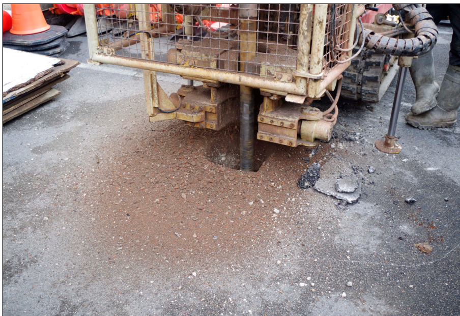
Plate 28: BH 16, made ground at around 2.0 m
