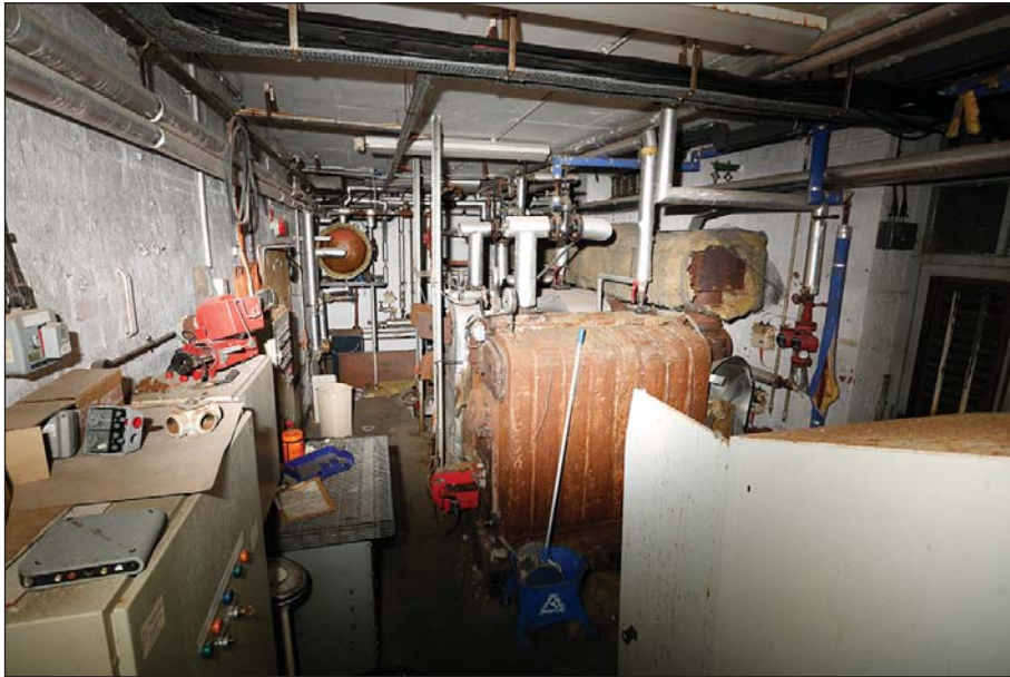
Plate 36: Main range lower ground floor: plant room (LG29)
