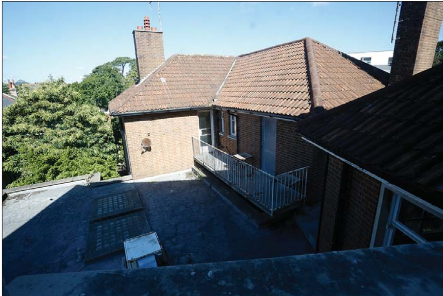
Plate 61: The roof of the Western Cell Block to illustrate how it joins the Annexe
