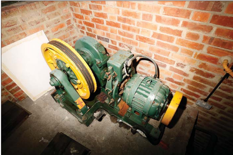
Plate 33: Main range third floor: OTIS lift A.C. motor
