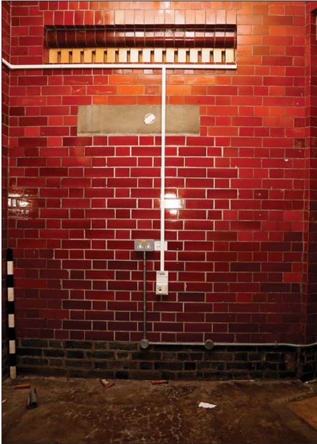
Plate 52: Detention lower ground floor: Blocked door within the former entrance lobby (LG11)
