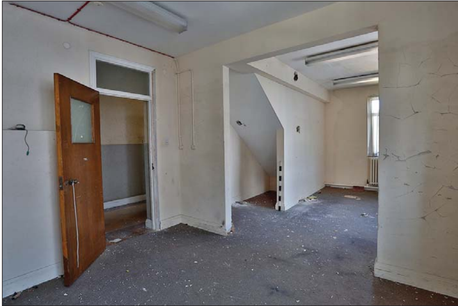
Plate 30: Main range second floor: Inserted second to third floor staircase and cut through partition wall (S05 and S06)
