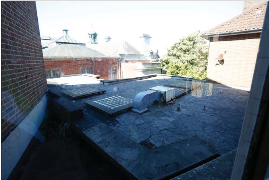
Plate 60: The roof of the Western Cell Block with the Annexe on the right and County Court in the background
