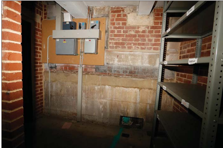
Plate 43: Detention lower ground floor: Previously external wall exposed within store room LG07
