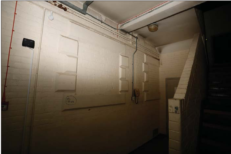
Plate 45: Detention lower ground floor: Previously external wall that includes blocked windows with rusticated surrounds
