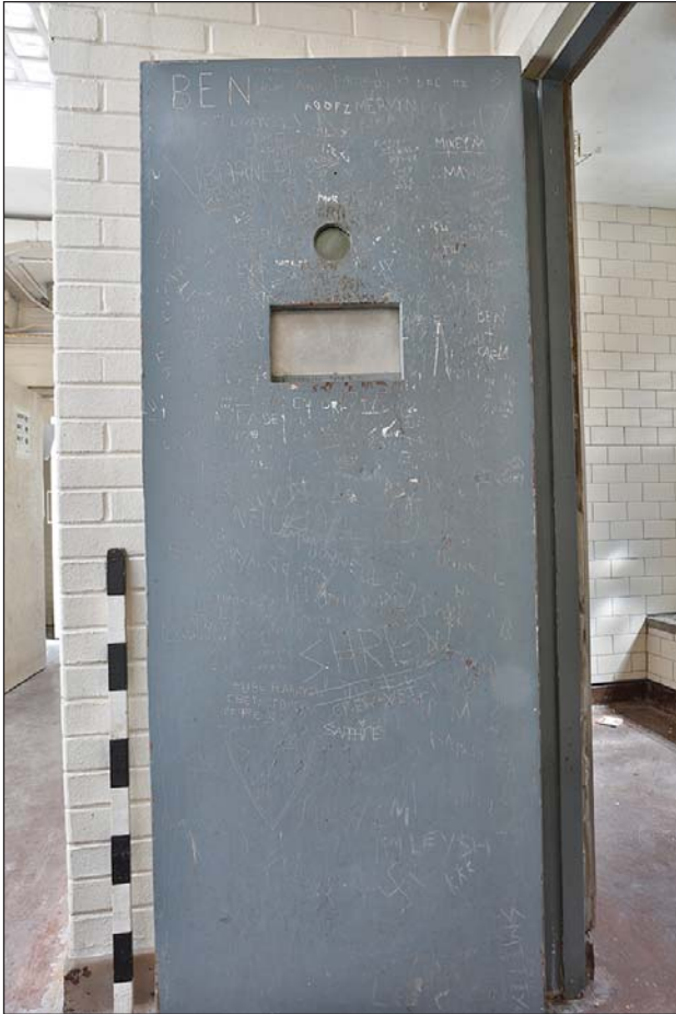
Plate 68: Detention ground floor: Western Cell Block - cell door graffiti (4F)
