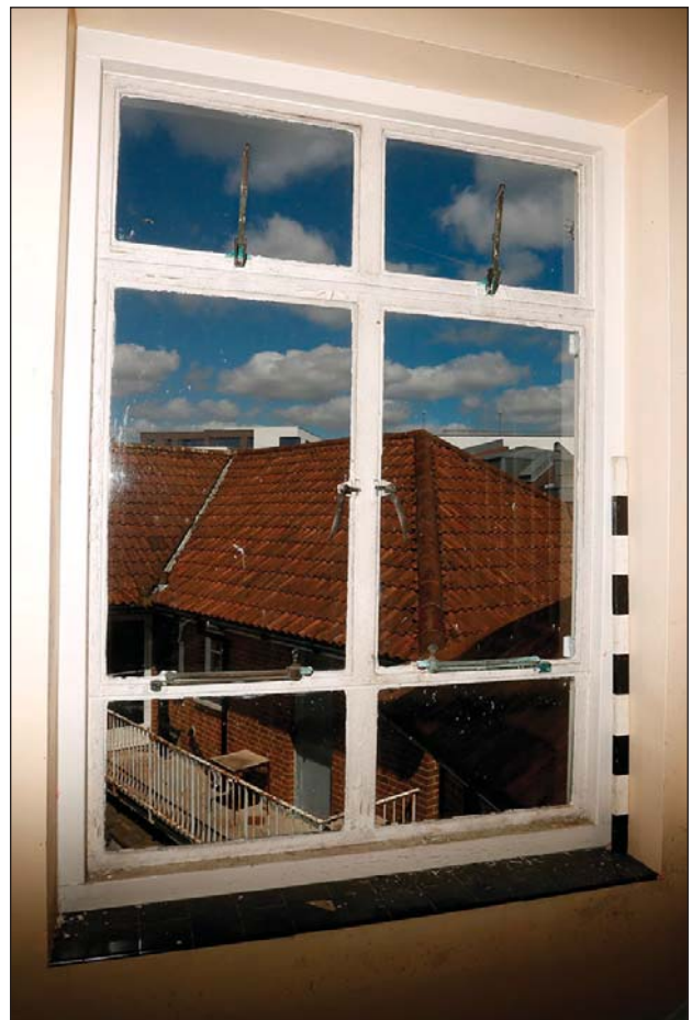
Plate 27: Main range first/second floor: example of a metal framed window complete with brass fittings
