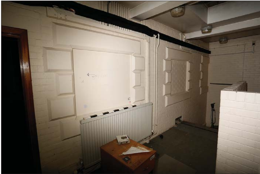
Plate 44: Detention ground floor: Previously external wall that includes blocked windows with rusticated surrounds
