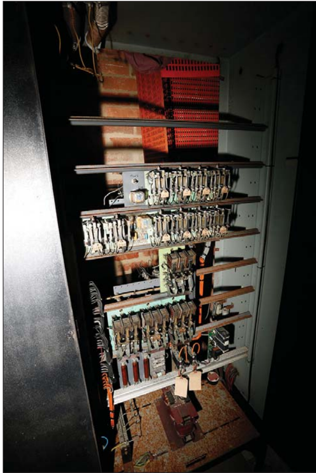
Plate 34: Main range third floor: OTIS lift A.C. motor
