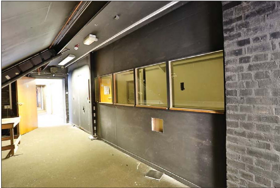
Plate 32: Main range third floor: Identification suite observation and parade rooms (T06 and T07)
