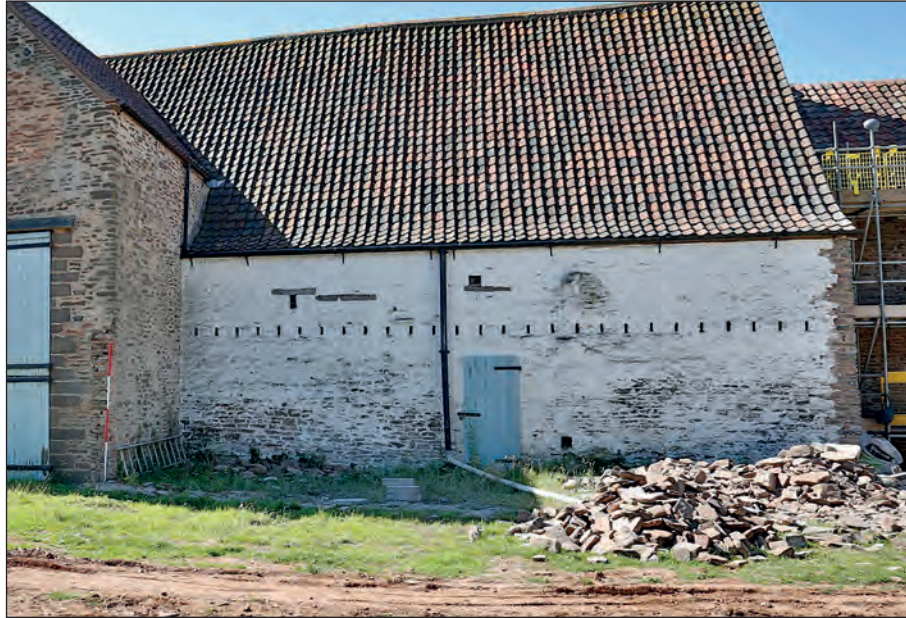
Plate 15: Main Barn north wall showing joist holes from earlier stables
