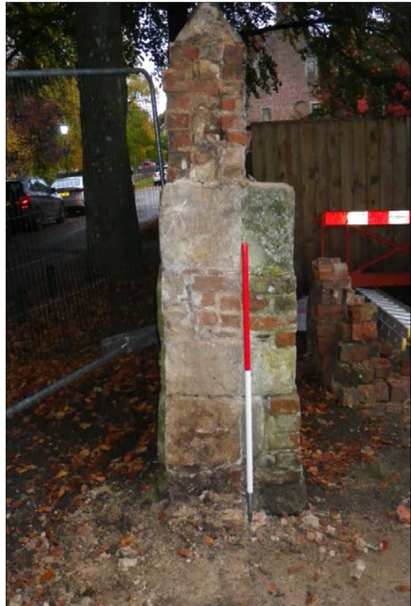
Plate 8: Detail of end of north section of wall and buttress following removal of blocking, viewed from the south
