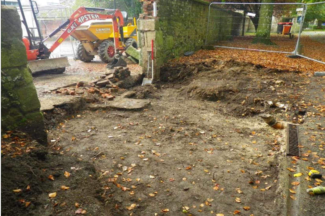
Plate 11: Ground reduction in progress to west of wall, viewed from the north
