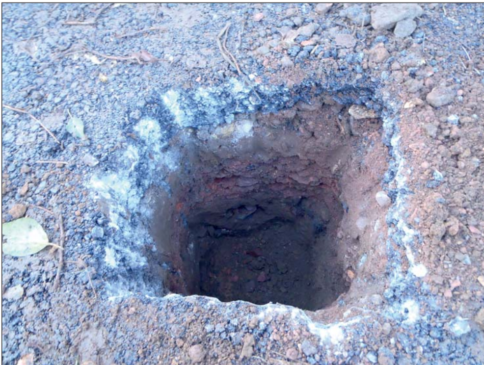
Plate 6: Post hole dug for gate post at south end of Site, showing, from base, silt 10003 , crushed brick 10004 , topsoil 10000 and tarmac laid down during works. Intervention is 0.6m deep in total
