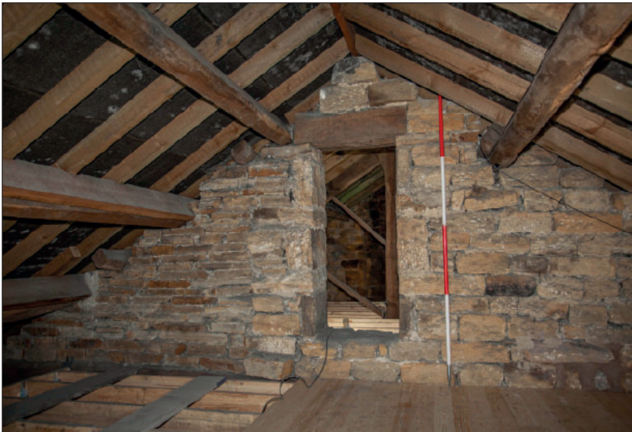
Plate 132: A1, spine wall with doorway to A2, notice the smaller tabular stone to the left
