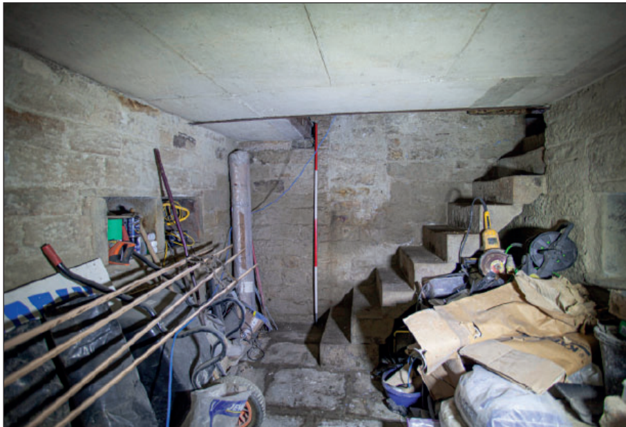
Plate 44: C2, blocked coal chute to the west wall and inserted staircase
