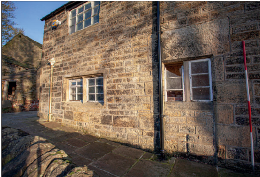
Plate 18: South elevation, primary doorway partially blocked with a later window
