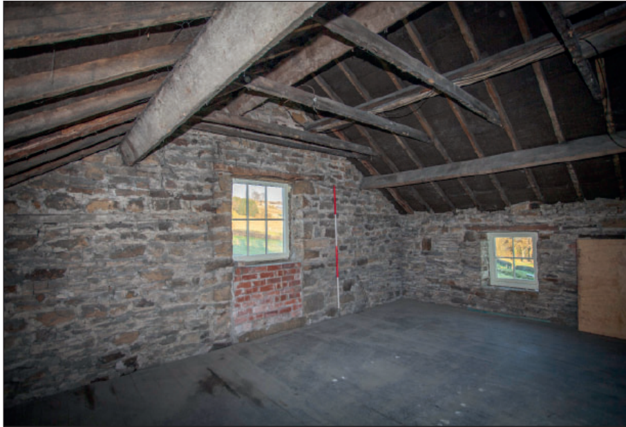
Plate 129: F10, general view
