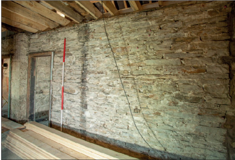
Plate 119: F6, east wall with scars of dismantled stud partition
