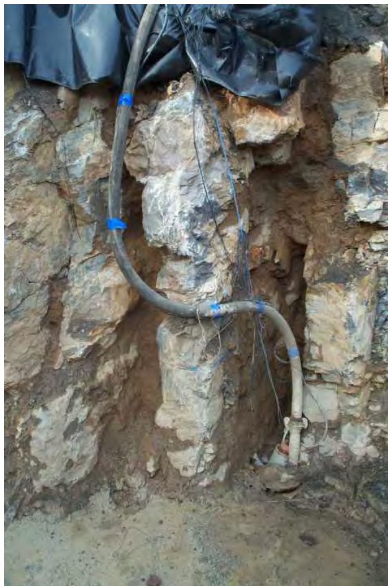
Plate 2: Close-up of fissures
