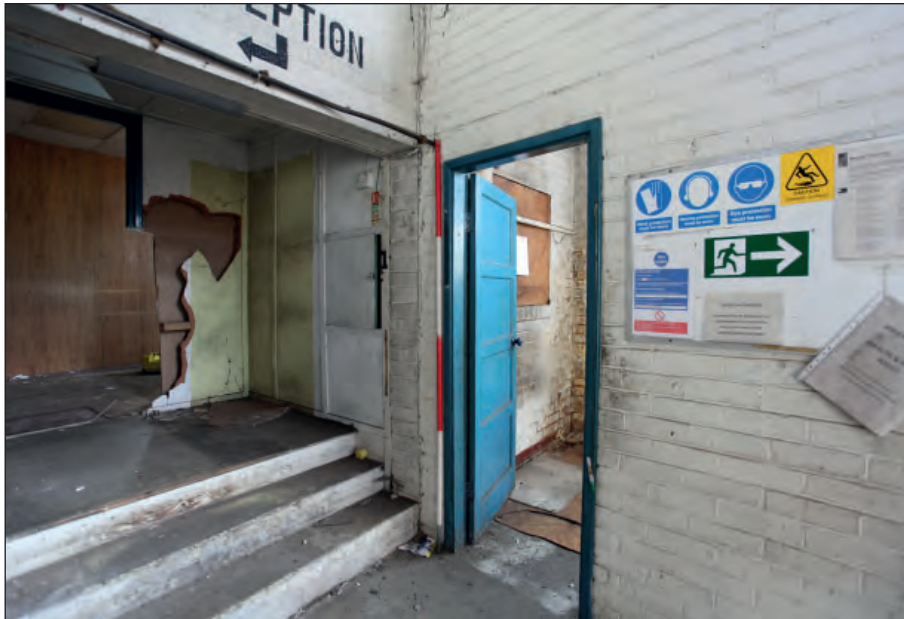
Plate 13: Building 1 - doorway to kitchen and steps to office within the south-eastern range
