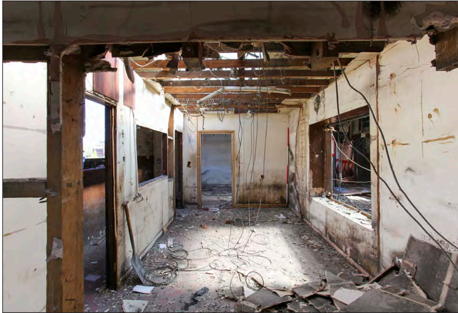
Plate 55: Pithead Baths, first floor, offices off link corridor to the Lamp Room, facing northeast
