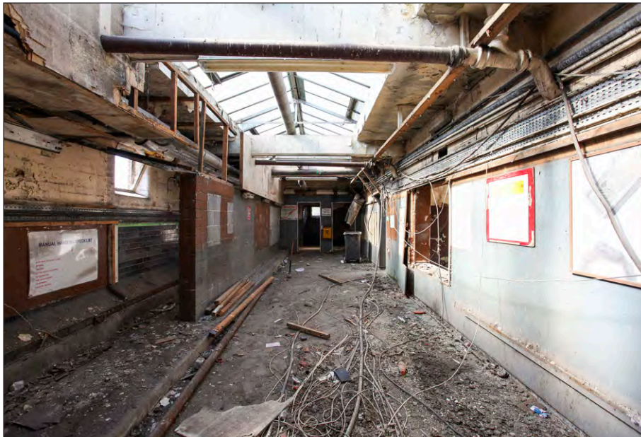
Plate 54: Pithead Baths, first flo , link corridor to the Lamp Room, facing southwest
