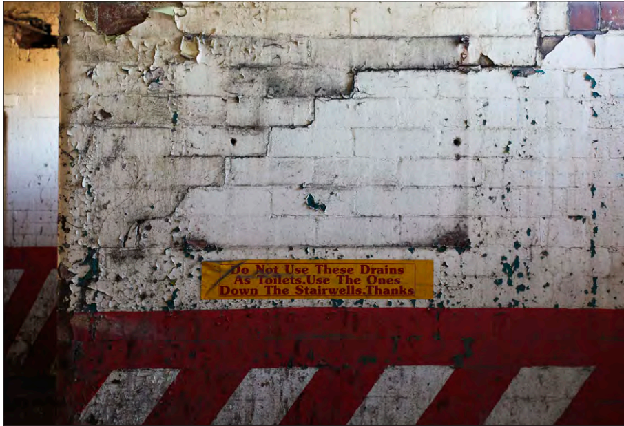
Plate 93: Lamp Room, first floor, detail of sign discouraging urination in the drains in corridor, facing northeast
