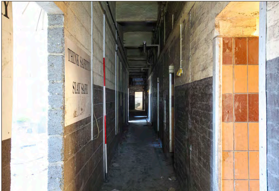
Plate 37: Pithead Baths, first floor, corridor formed by inserted walls within dirty locker room, facing southeast
