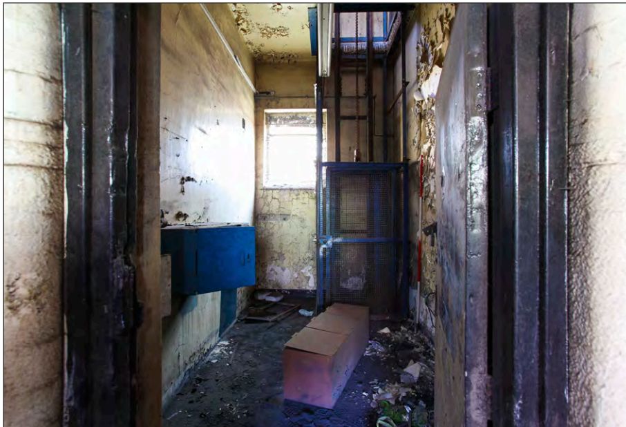
Plate 46: Pithead Baths, ground floor , lift room off clean locker room, facing southeast
