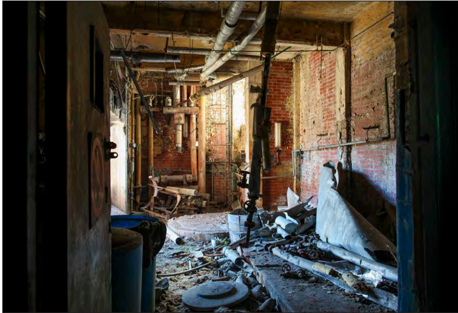
Plate 49: Pithead Baths, ground floor , plantroom viewed from doorway, facing south-west
