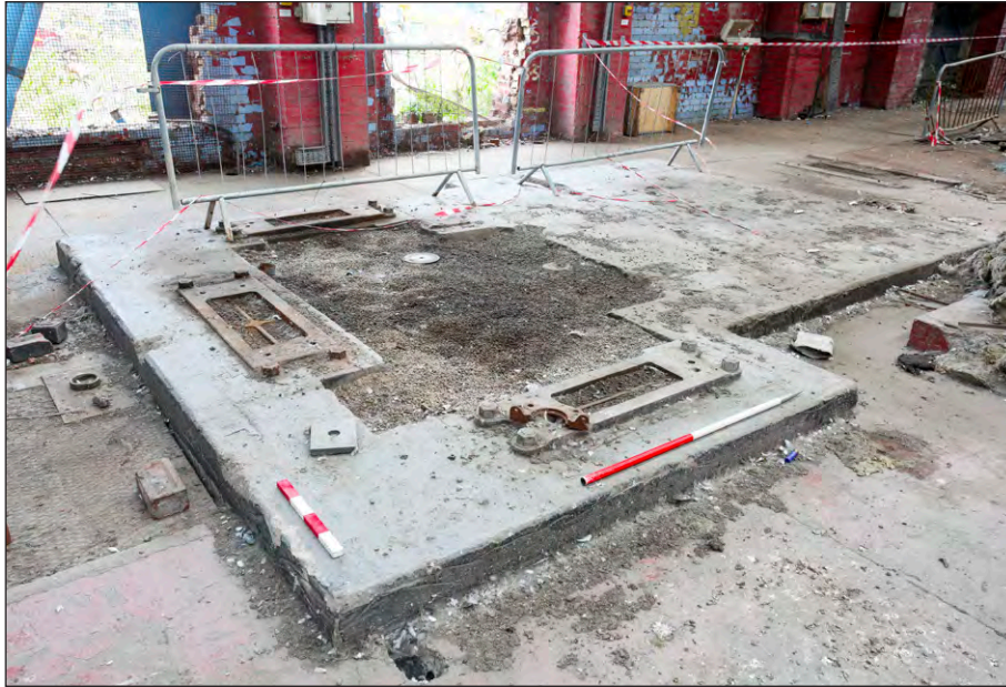
Plate 9: Powerhouse, principal room, plant base, facing east
