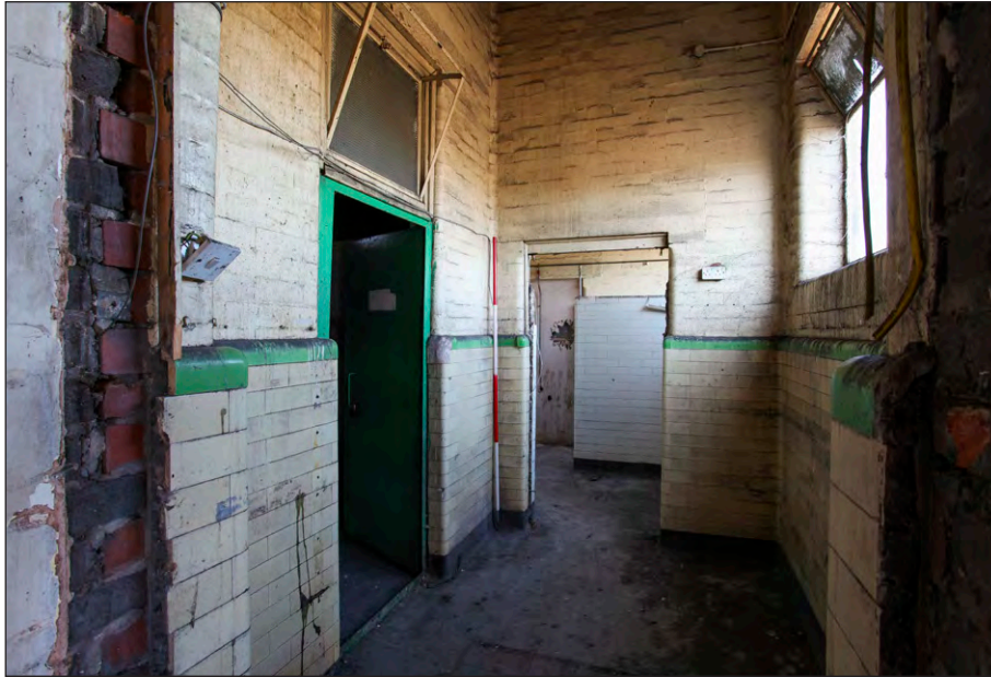
Plate 51: Pithead Baths, ground floor , showers and toilets within northeast section, facing northeast
