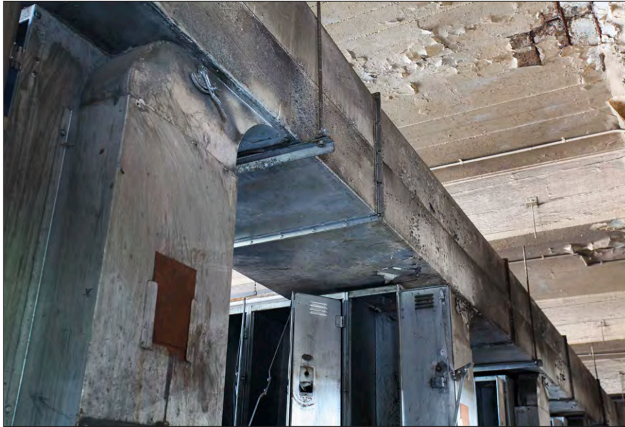
Plate 45: Pithead Baths, ground floor , detail of ducts for heated locker system in dirty locker room, facing east
