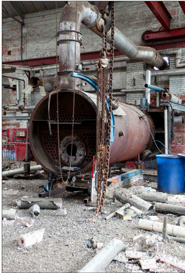
Plate 7: Powerhouse, principal room, boiler, facing north
