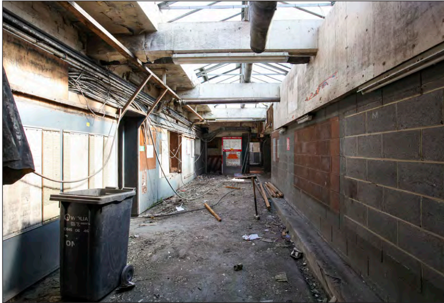
Plate 53: Pithead Baths, first flo , link corridor to the Lamp Room, facing northeast
