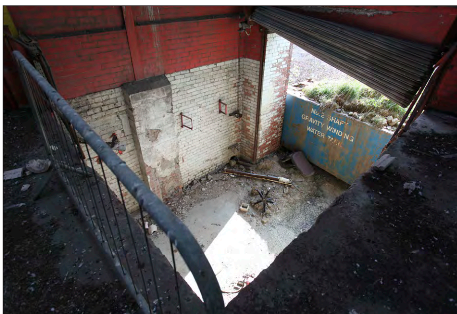
Plate 16: Powerhouse, principal room, garage bay with water tank
