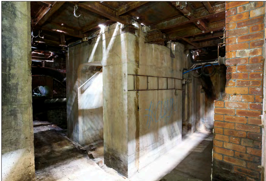
Plate 26: Powerhouse, example of cellar corridor space beneath the southeast end of the principal room, facing east
