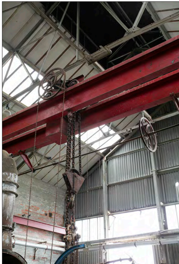
Plate 12: Powerhouse, principal room, traveling crane
