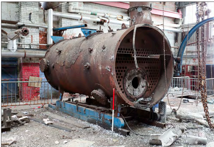
Plate 8: Powerhouse, principal room, boiler, facing east
