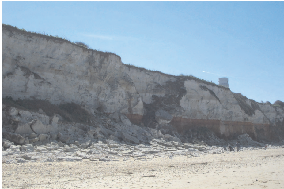
Plate 1. An example of cliff collapse at Hunstanton in the east of the CRSA
