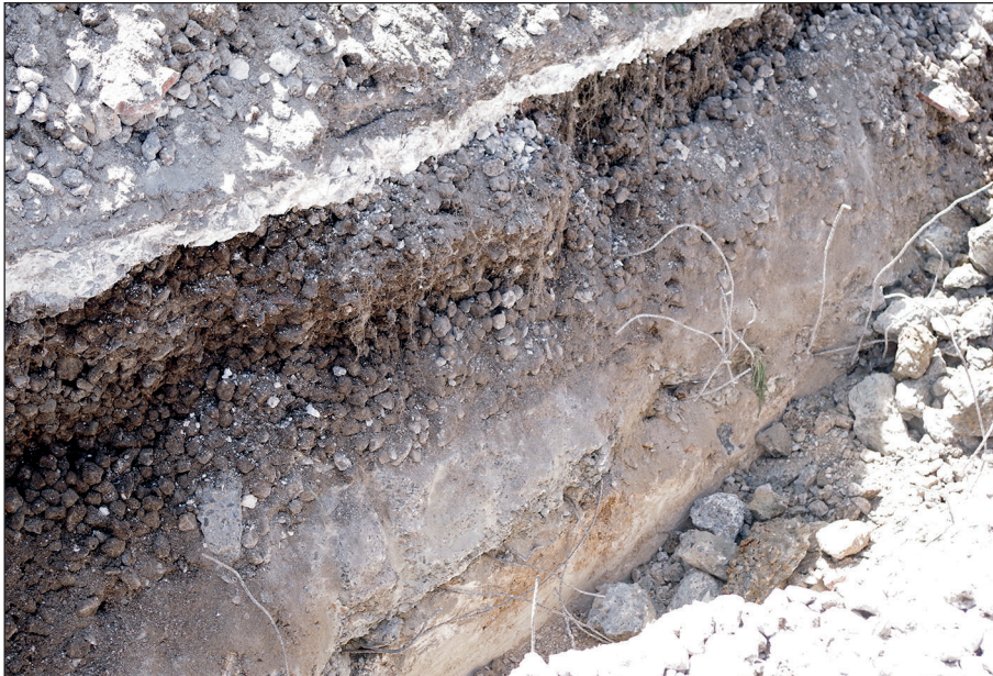
Plate 4: North-east facing representative section of cable trench showing made ground within the old sewage beds at the WWTW
