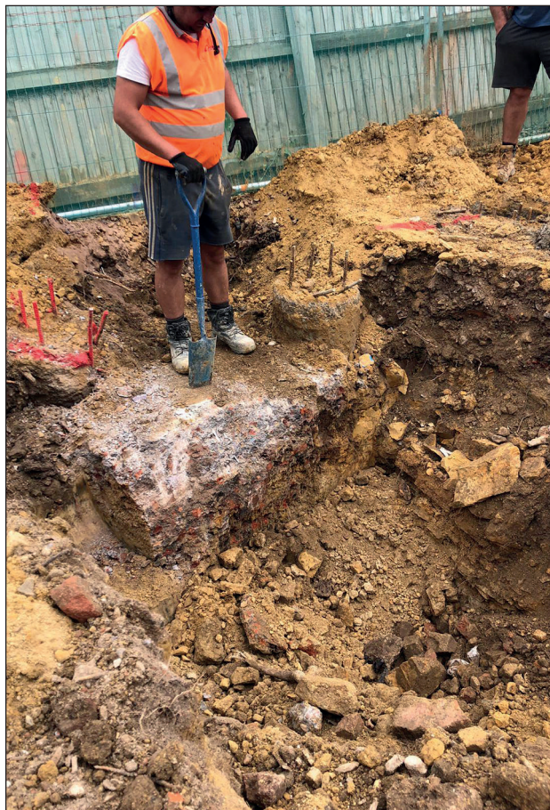
Plate 4: Concrete post in the northwest corner of the site, pre-ex, viewed from the southwest
