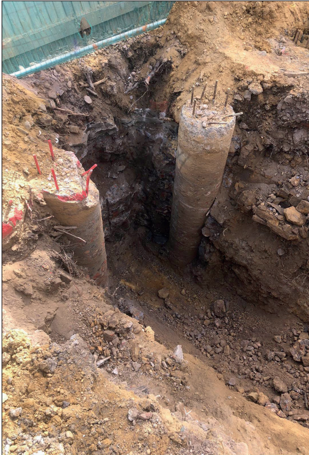
Plate 5: Concrete post in the northwest corner of the site, post-ex, viewed from the southwest
