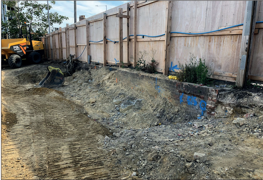
Plate 3: Wall at the eastern edge of the site, viewed from the south
