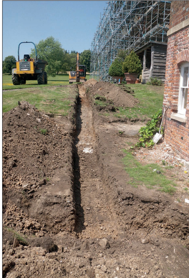
Plate 1: Excavation of oil feed trench (Trench 1) at the rear of the manor house. View from the east.
