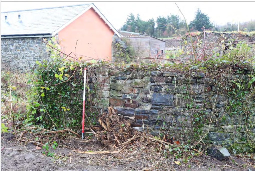
Plate 62: Former farm range building 8 evidence of reduced and blocked window opening
