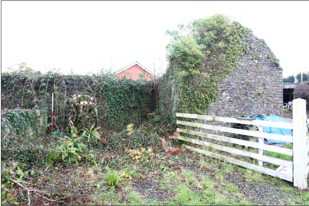
Plate 59: Former farm range building 8 north-west corner showing horse-gin walling to left of image
