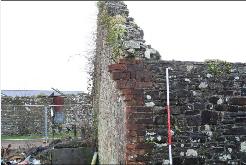
Plate 43: Open fronted cart shed Building 3, detail of characteristic corbel detail in brick
