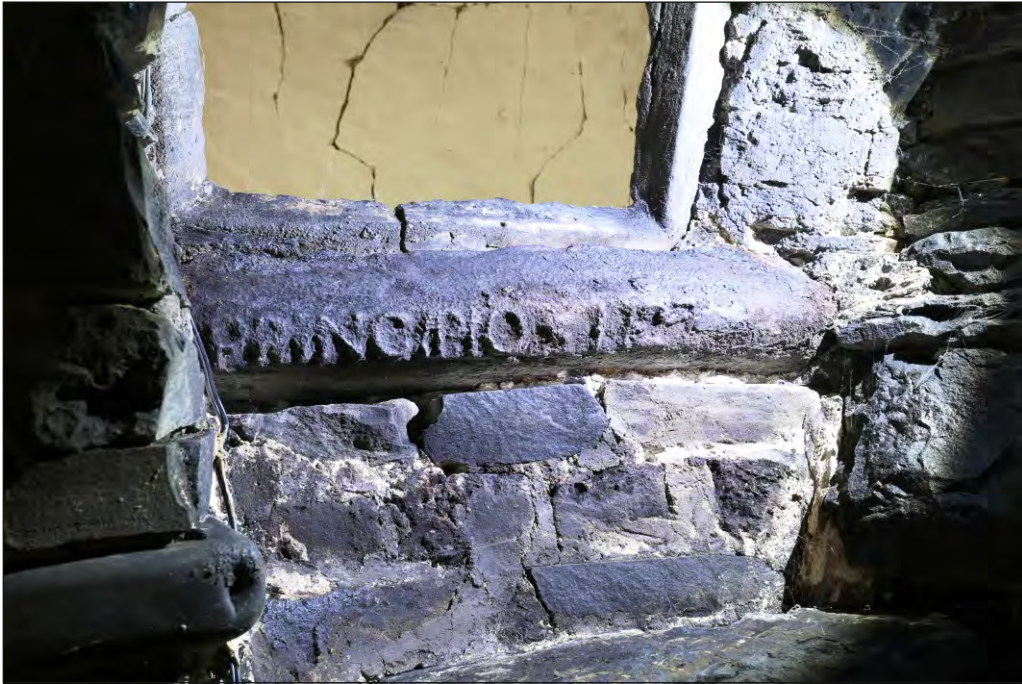
Plate 19: Steart Farmhouse room G4 detail showing inverted view of embossed cast iron lintel above north cloam oven 'Principio 1727'
