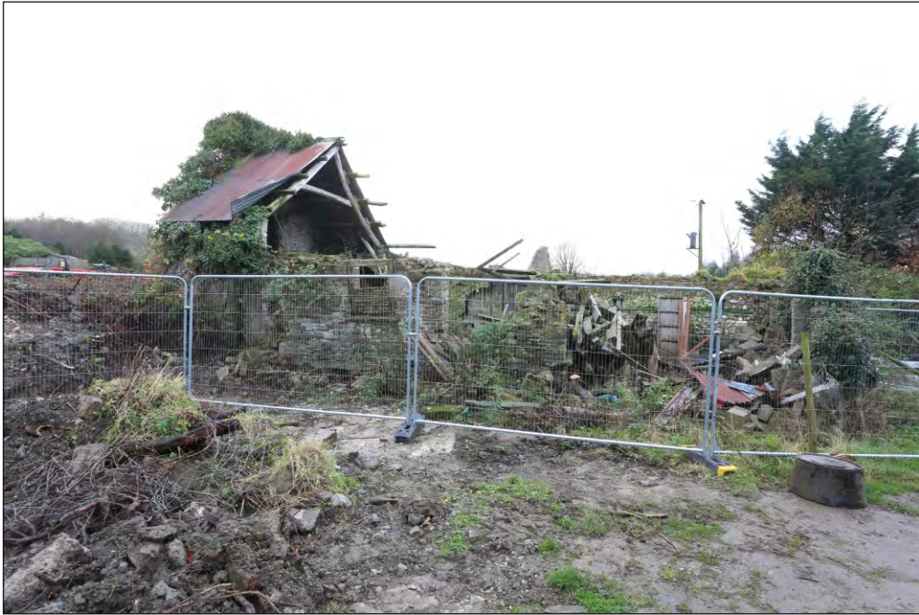
Plate 63: Former barn building 2 collapsed state
