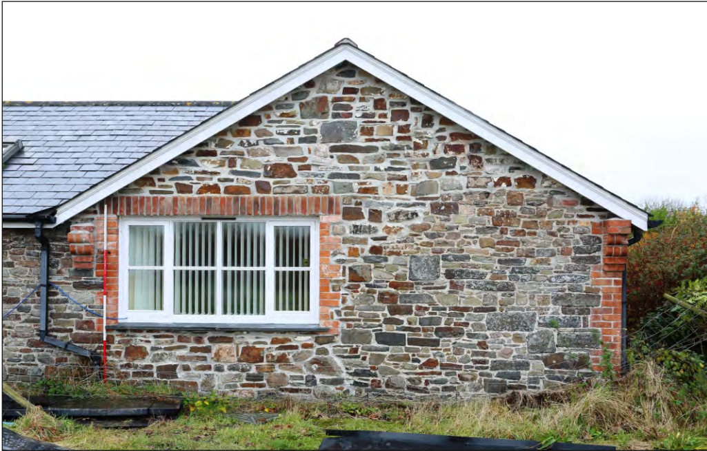
Plate 51: Former farm range building 4 inserted window and rebuilt gable north end of east elevation
