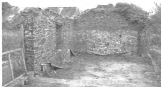
Figure 42a. Exterior and interior of the west end of building 08. (Interior from RPS plate 16, Appendix 12). The damp proof membrane (blue plastic sheet) beneath a concrete floor indicates that work to convert/repair the building have commenced but have never been finished
