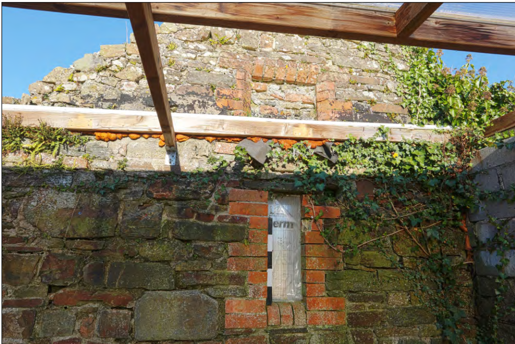
Plate 44: Open fronted cart shed Building 3, south gable wall showing window and commemorative plaque recess
