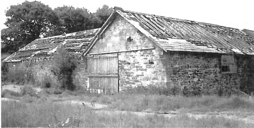
Figure 44. 1995 photograph, north elevation of building 08 and east elevation of building 04. Rolle corbels to the gable that extends building 08 to master the end of building 04 newly built as part of the Rolle improvements
