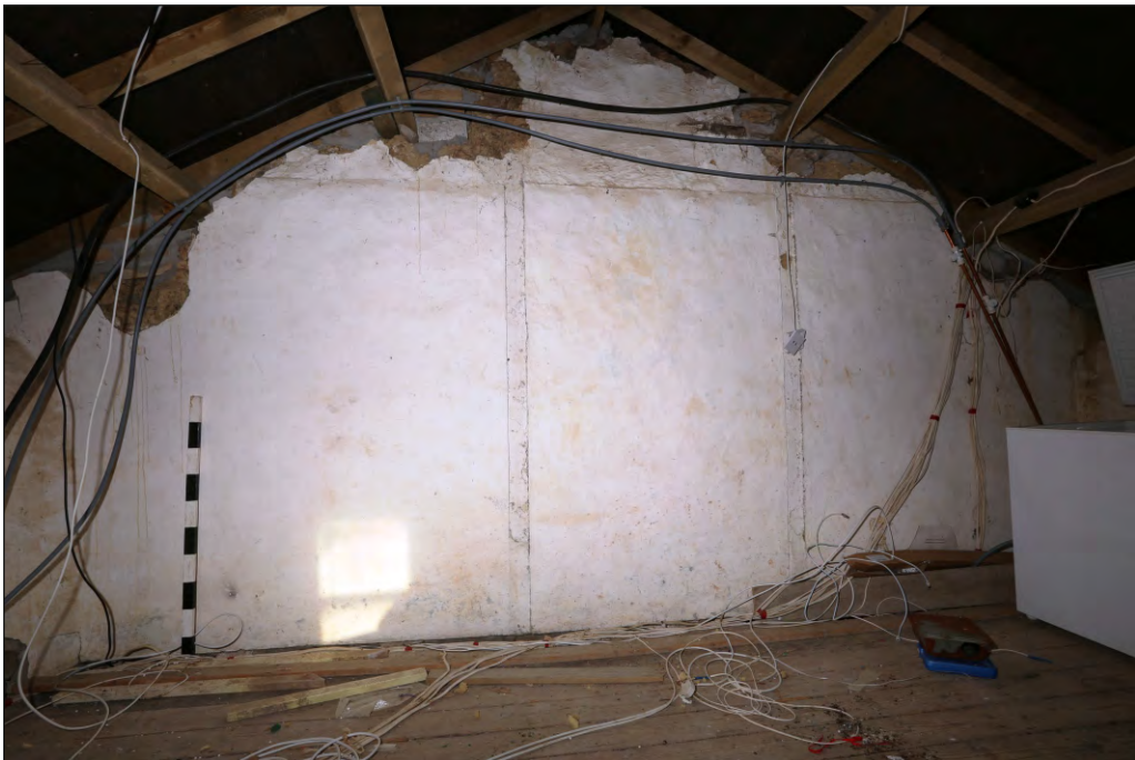
Plate 40: Steart Farmhouse south-west wing first floor room F6 north cob dividing wall and timber studs
