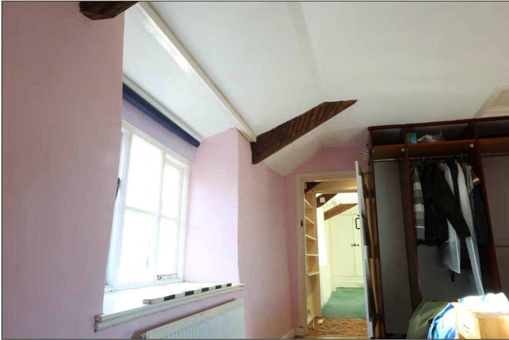
Plate 35: Steart Farmhouse first floor view along south side showing exposed original principal rafters to roof
