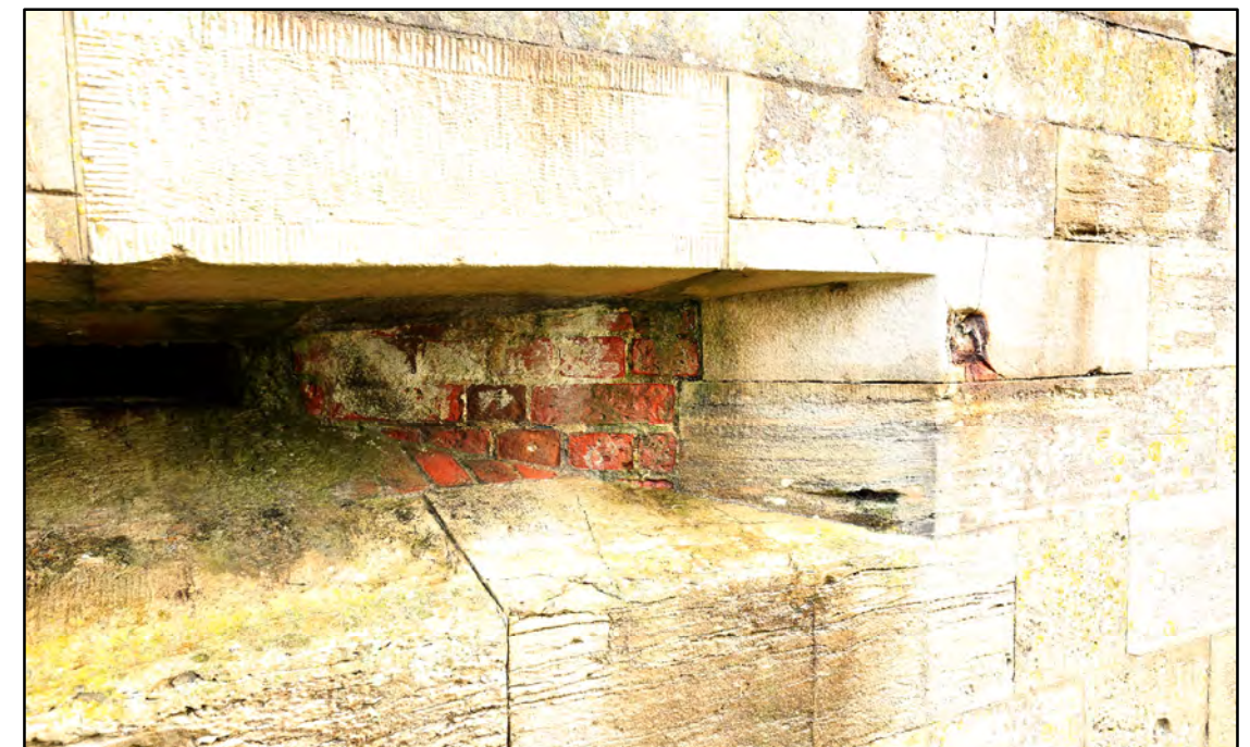
Gun embrasure within wall of counterscarp tunnel showing brick and stone construction
