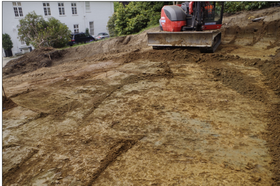
Plate 4: Ground reduction within a garage footprint in progress, viewed from the north east
